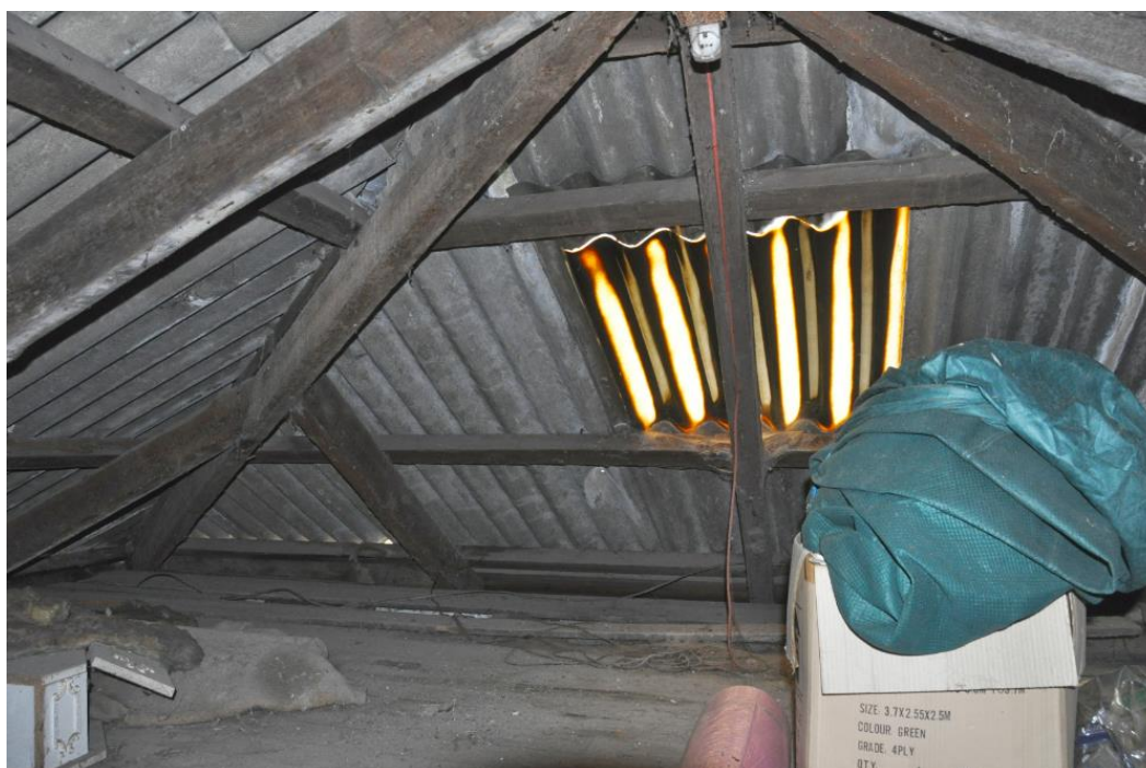
Image showing unlined roof void with light incursion and lack of available dark sheltered roost features.
