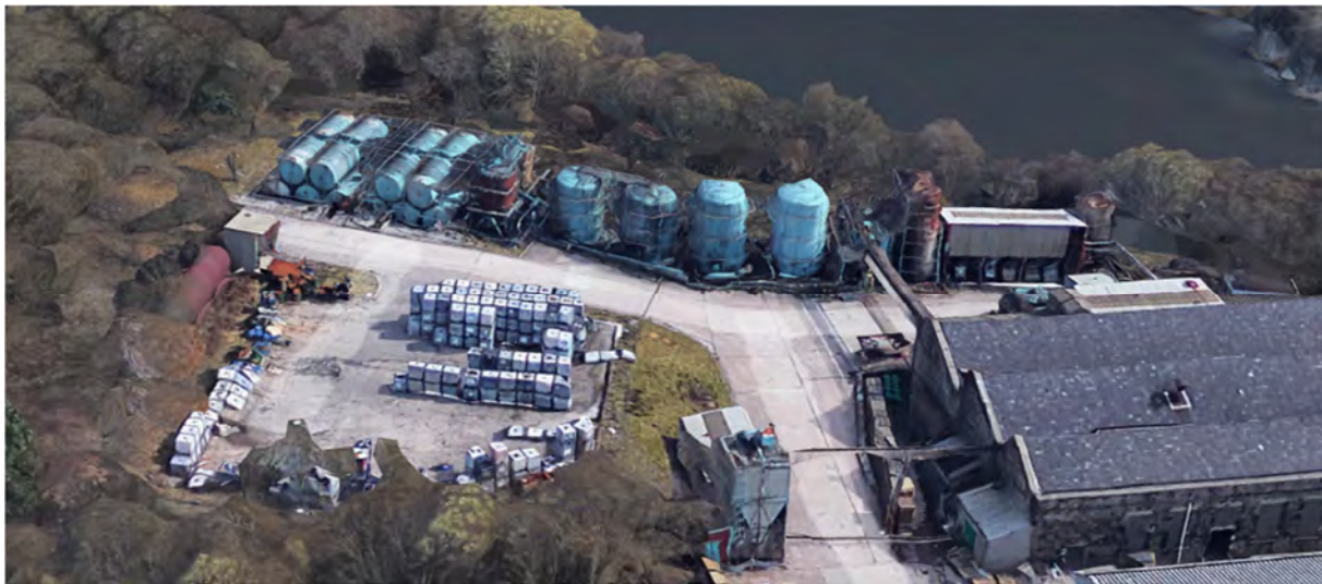
Above Ground Storage Tanks (ASTs)
