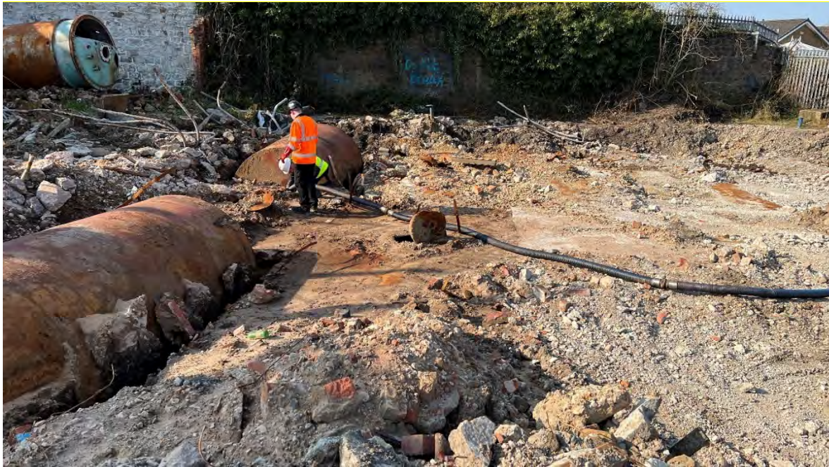
Underground Storage Tanks (USTs)
