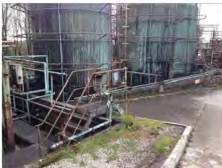
Plate 9 - Large Solvent Storage Tanks in Northern Tank Farm
