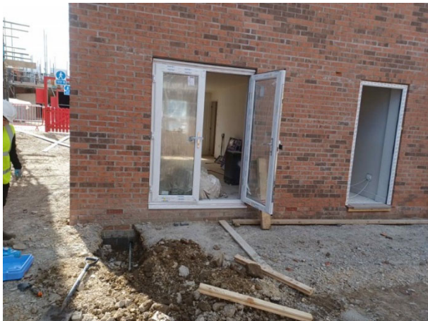
Plot 58 (VP3) sub-floor void installation location
