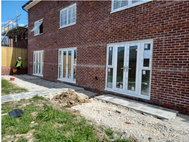
Plot 63 (VP1) sub-floor void installation location
