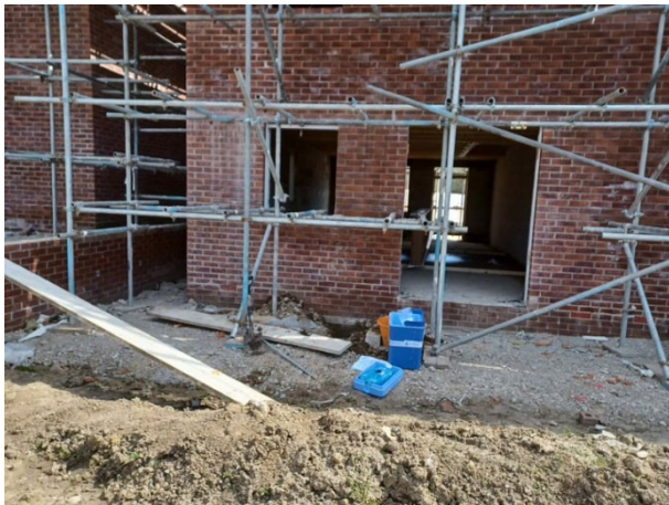
Plot 61 (VP2) sub-floor void installation location
