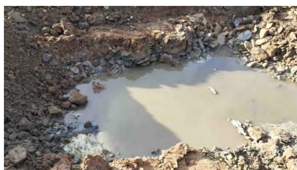
Photograph 34 – Exposed drainage run flooded excavation
