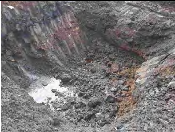
Ingress of water at base in competent rough rock
