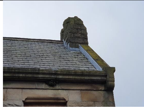
B1 Visible gaps within the ridge line and surrounding flashing
