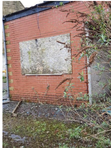
B2 Ground floor boarded up window
