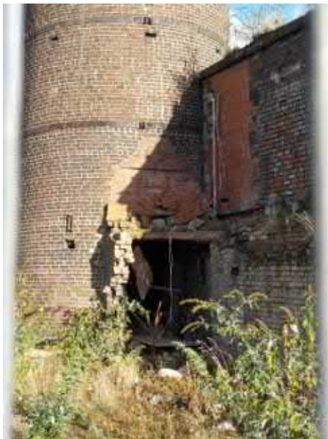
Concrete soffit to entrance partially collapsed
