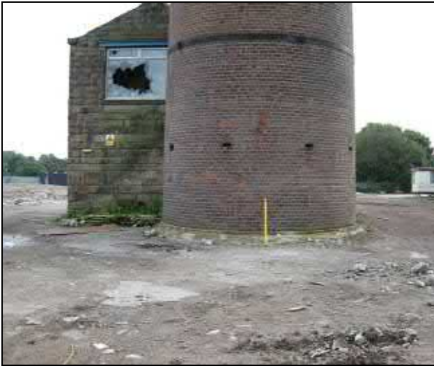
North elevation showing recent impact damage and evidence of base movement in past
