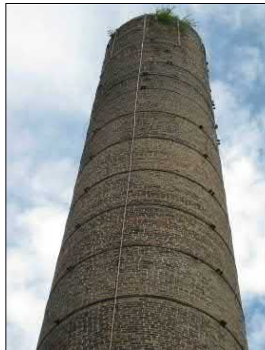
West elevation showing outwards movement of walls
