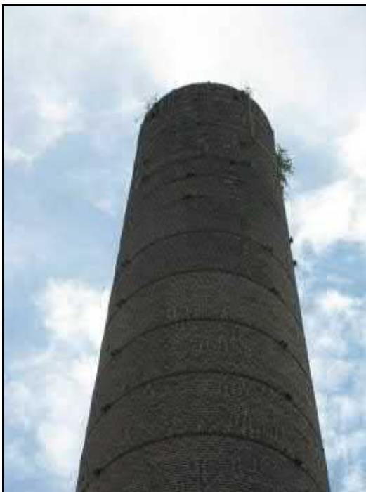
North elevation showing cracks to top
