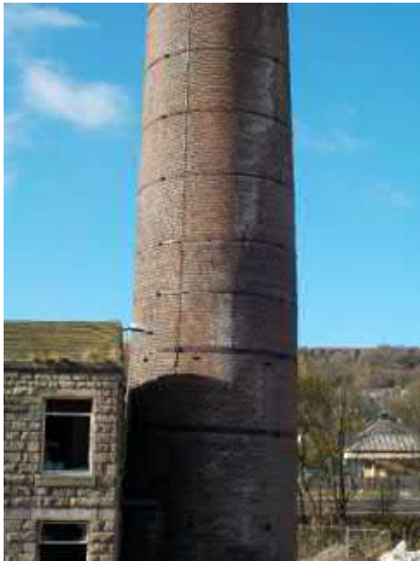
Efflorescence to East Elevation
