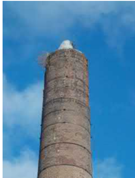
Mortar deterioration to South Elevation
