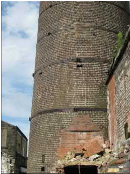
South elevation showing previous repairs near bottom
