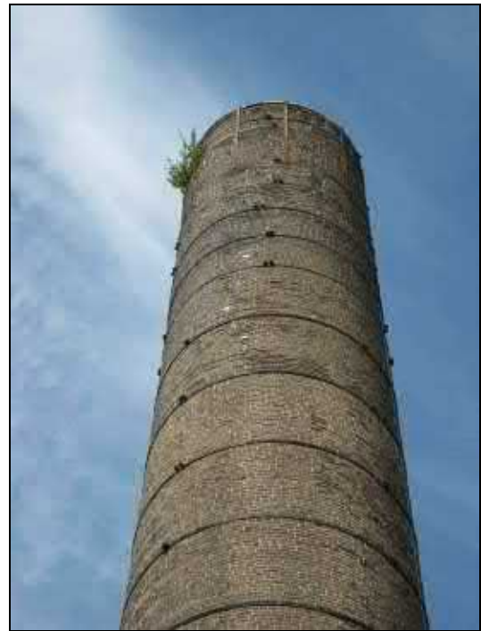
South elevation showing masonry re-pointing erosion and cracking
