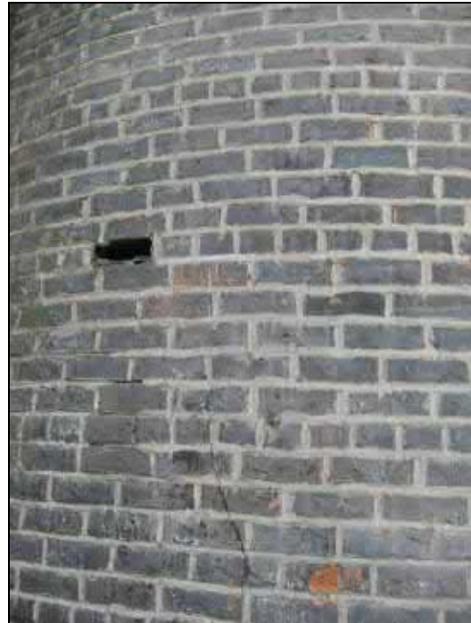
Crack recently propagated in east elevation
