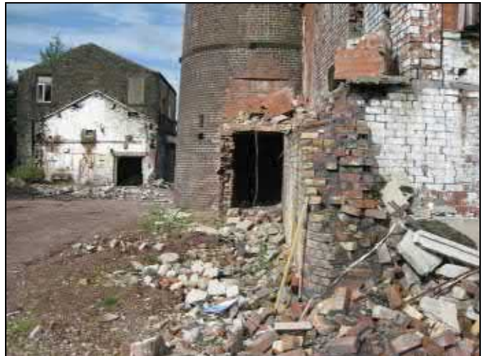
South elevation showing extremely unstable building connected to bottom of chimney
