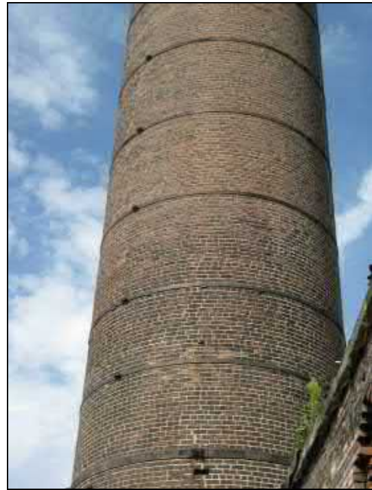
South elevation showing weathering of masonry and mortar
