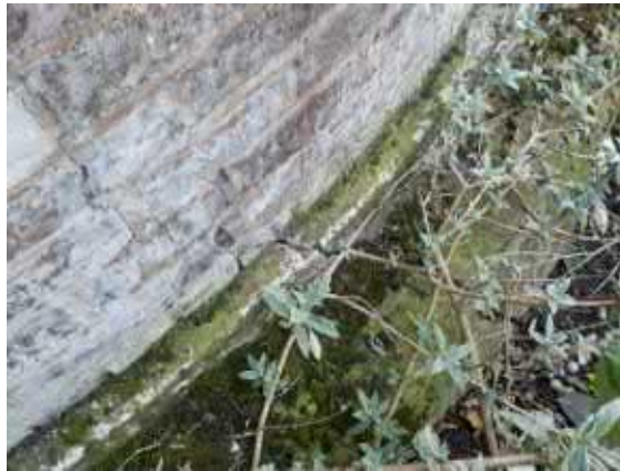
Cracking to base of East Elevation
