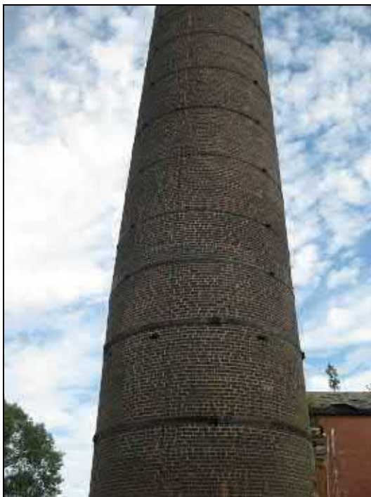
West elevation showing previous repair at approximately 10m.
