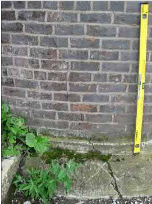
Historic crack of foundation to east elevation with recent movement apparent
