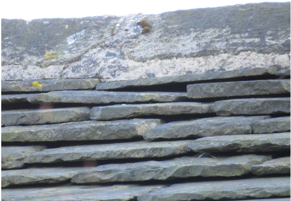
7 - There are gaps between stone roof tiles.
