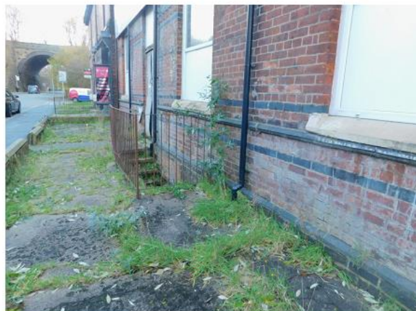
PHOTO 6 View of Closed Basement Entrance
