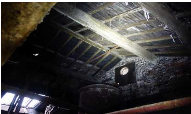
Exposed slates with evidence of considerable water penetration.
