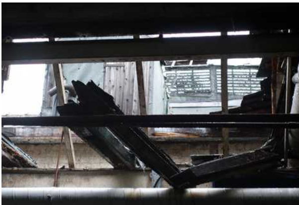
Area of missing slates and roof beyond in poor condition
