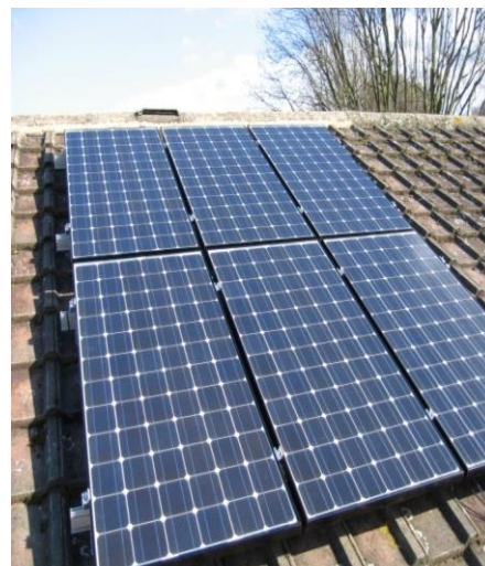
Figure 5 - Photovoltaic array on a pitched roof
