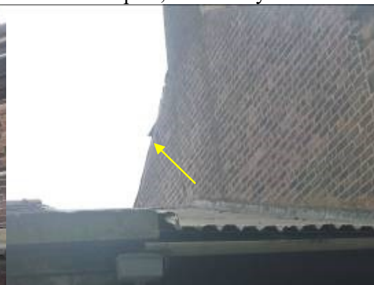
P4 Loose slate at North end of property
