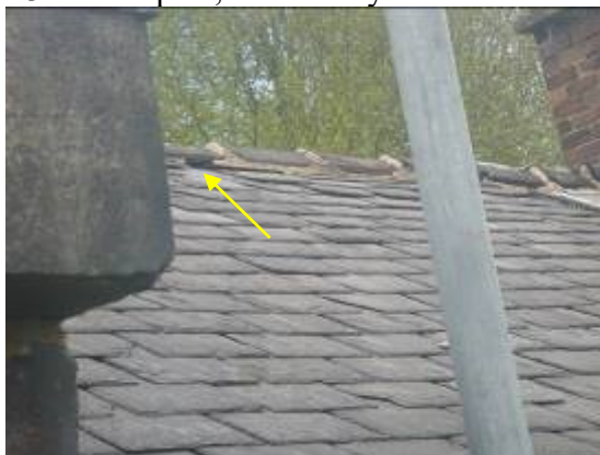
P5 Smithy roof from East, gap under tile
