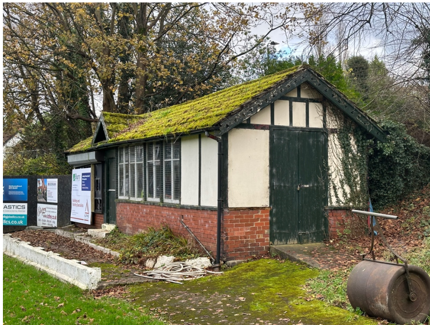
The dilapidated original pavilion building.
