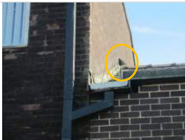
Photo 10: Minor gaps at lifted lead flashing on Building 4
