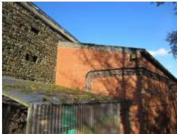
Photo 6: East elevation of Building 3 showing holes in stone elevation wall and cement sheeting fascia at a brick annex
