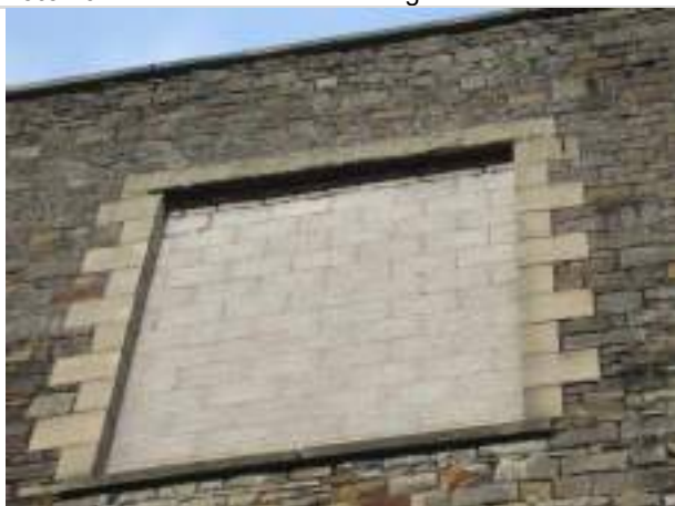
Photo 21: Gaps beneath window lintels at south elevation of Building 7
