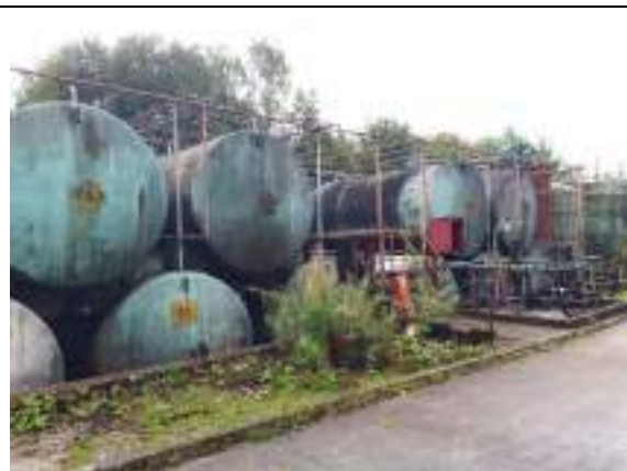
Tank Farm at area 11
