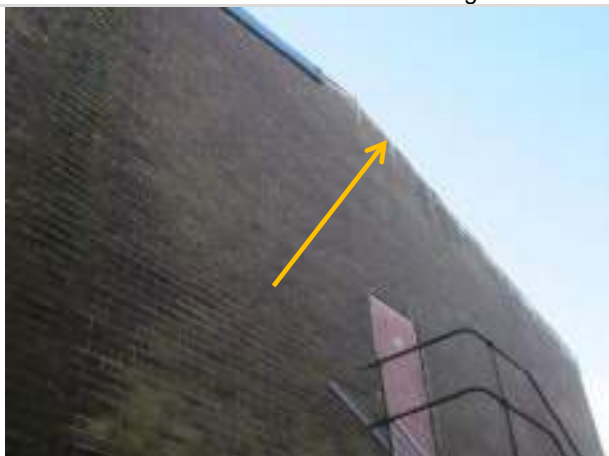
Photo 11: North elevation of Building 4a and missing fascia
