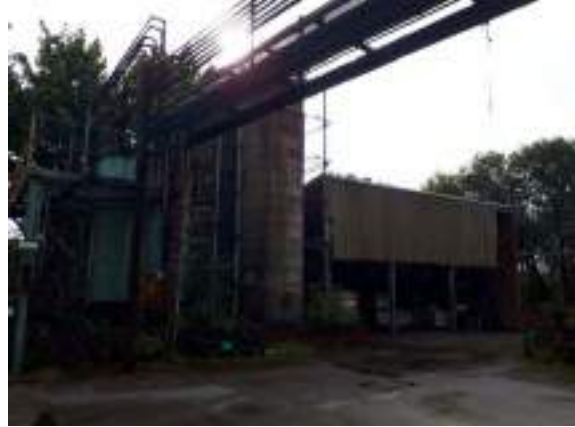
Solvent recovery plant at area 11
