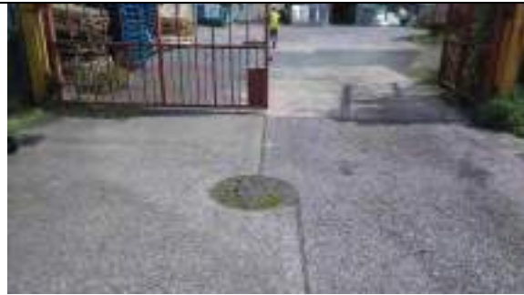
Off-site drain cover on Mill Road associated with elevated PID readings in chamber
