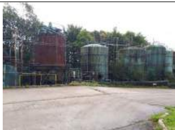
Tank Farm at area 11
