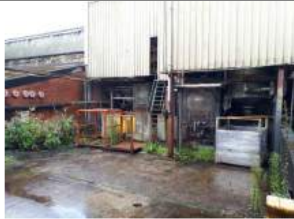
Solvent Filling room at Area 10
