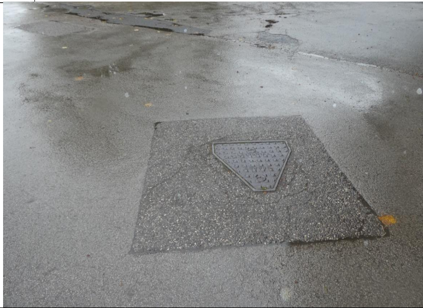
Photograph 24. Reinstatement to inspection chamber cracked and eroding
