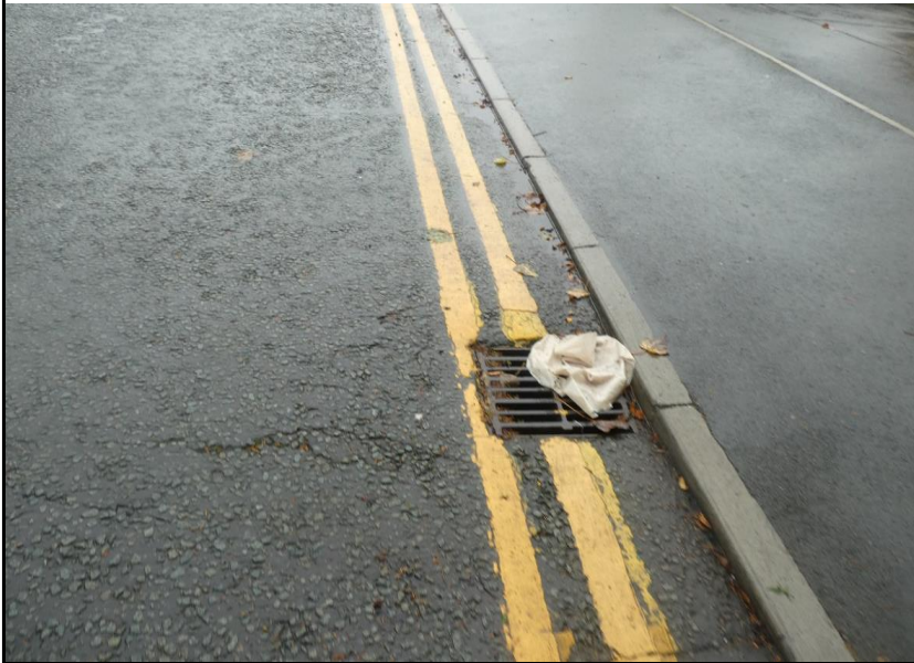
Photograph 43. Localised erosion to surfacing.
