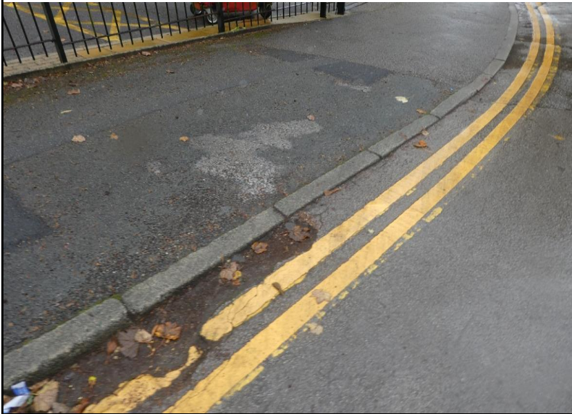
Photograph 23. Uneven and damaged kerb to George Street
