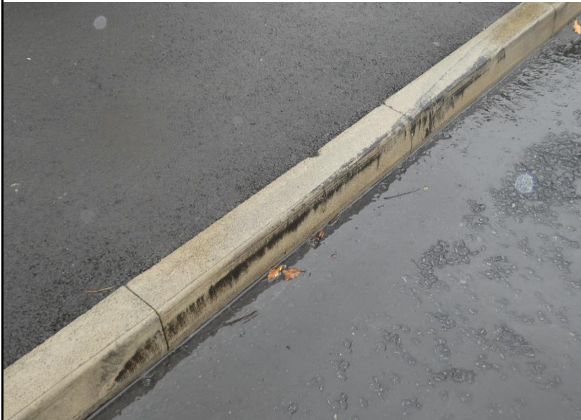
Photograph 7. Staining to the kerbing
