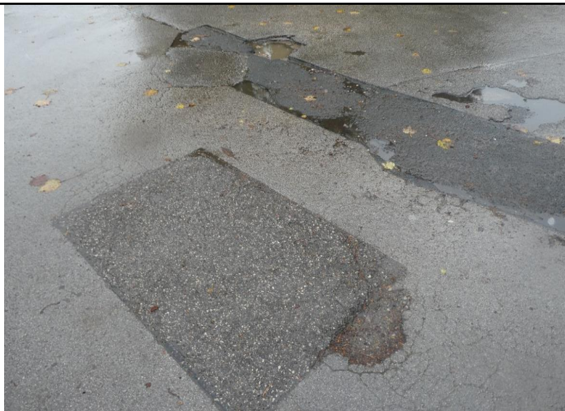
Photograph 26. Reinstated area of surfacing damaged and eroded
