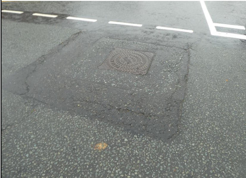
Photograph 51. Cracking and erosion to surfacing.
