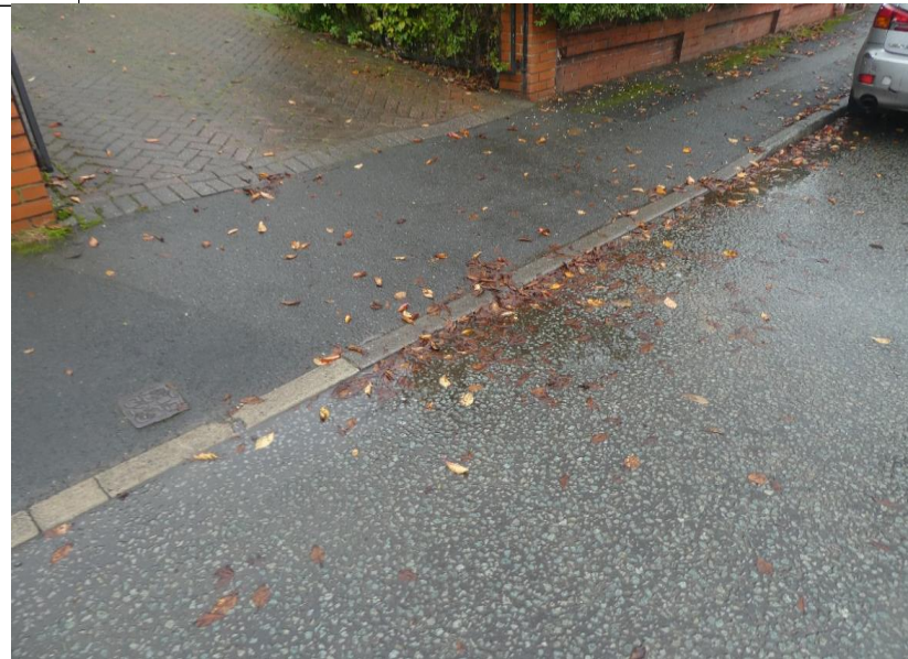
Photograph 60. Localised damage to kerbing
