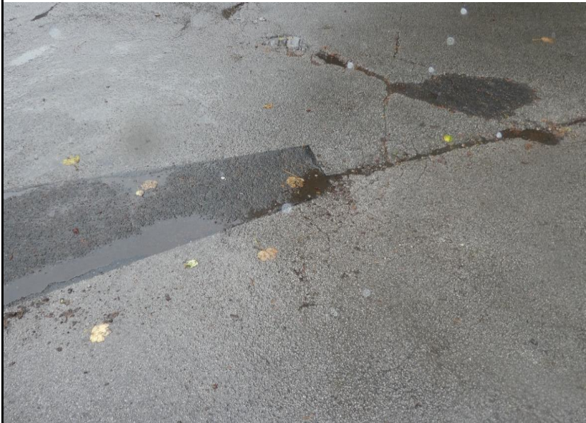
Photograph 27. Reinstated area of surfacing damaged and eroded
