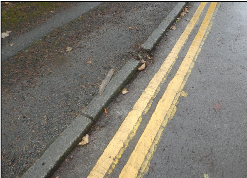
Photograph 21. Uneven and damaged kerb to George Street
