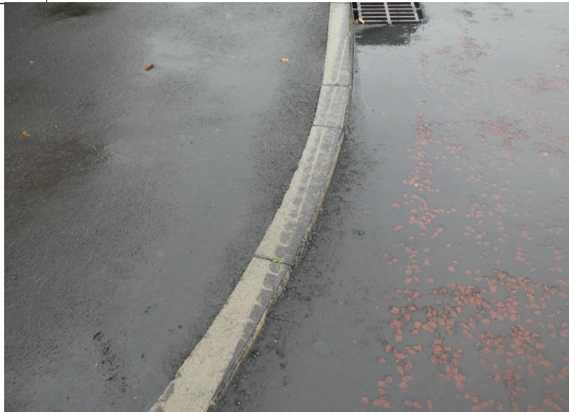
Photograph 4. Kerbing is stained and marked on both sides of the roadway
