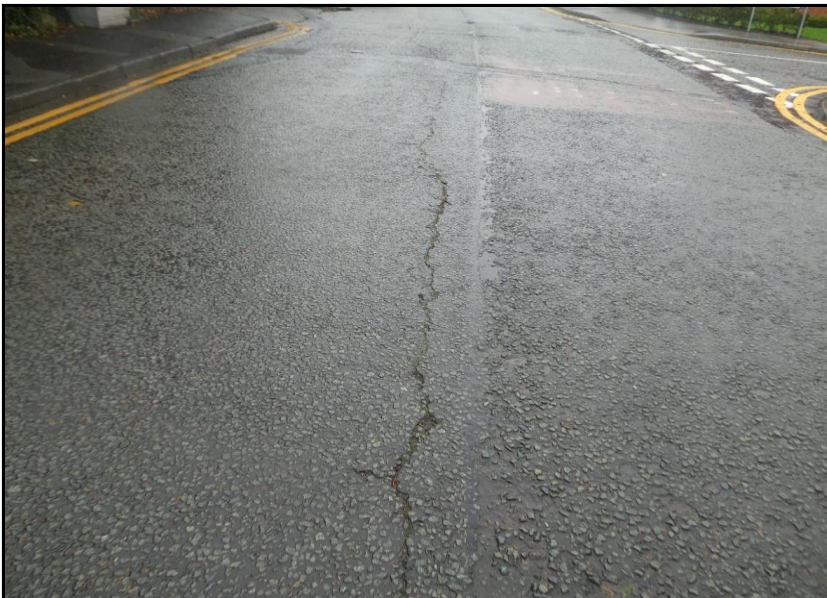
Photograph 45. Cracking to surfacing to centre of roadway.
