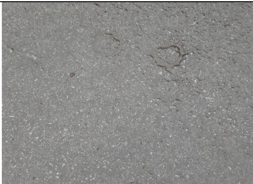
Photograph 10. Localised indentations to footpath areas
