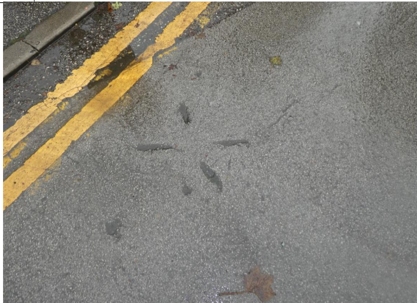
Photograph 28. Localised indentations to road surfacing
