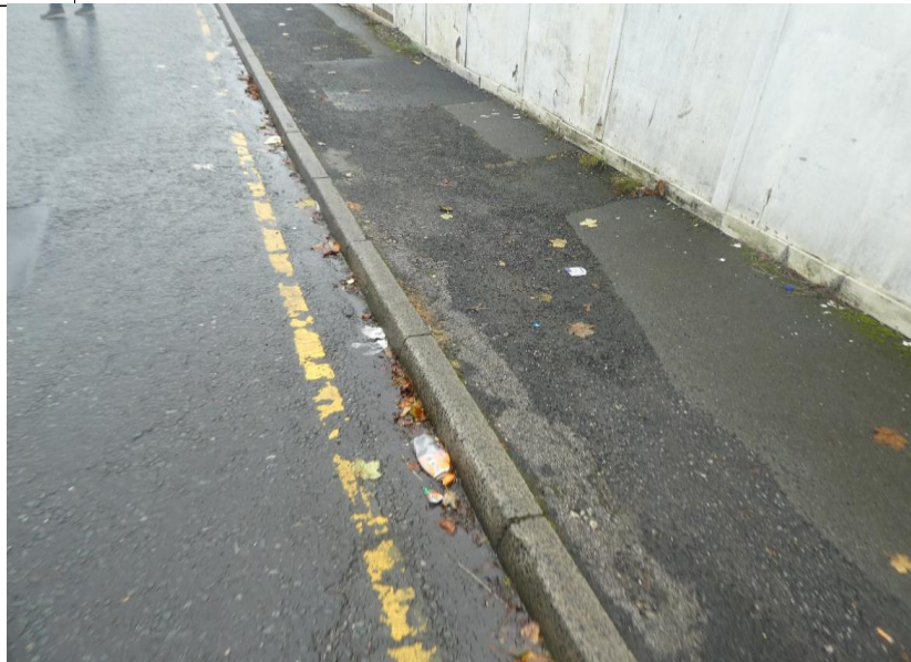
Photograph 84. Localised erosion to footpath.
