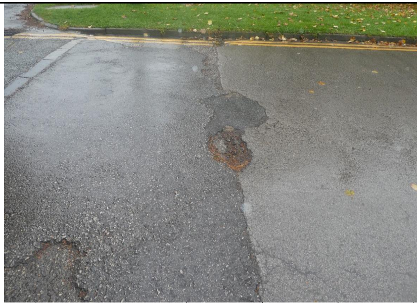
Photograph 30. Localised erosion to surfacing
