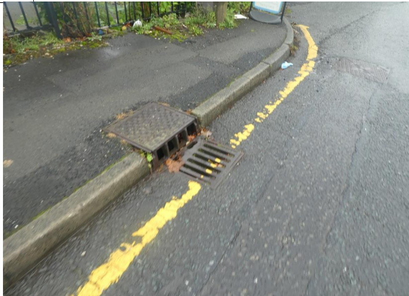
Photograph 88. Erosion to line marking.
