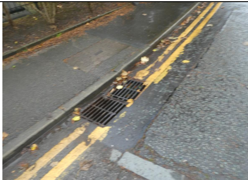
Photograph 34. Localised erosion to surfacing
