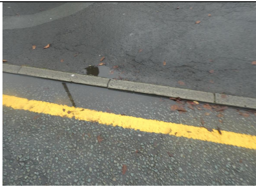
Photograph 62. Erosion to footpath surfacing of junction to business premises
