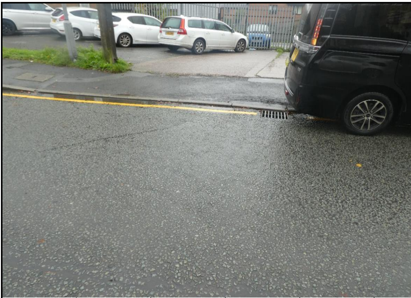
Photograph 61. Minor erosion to surfacing
