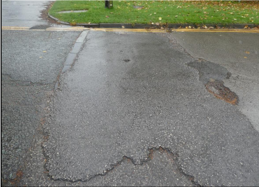
Photograph 31. Localised erosion to surfacing
