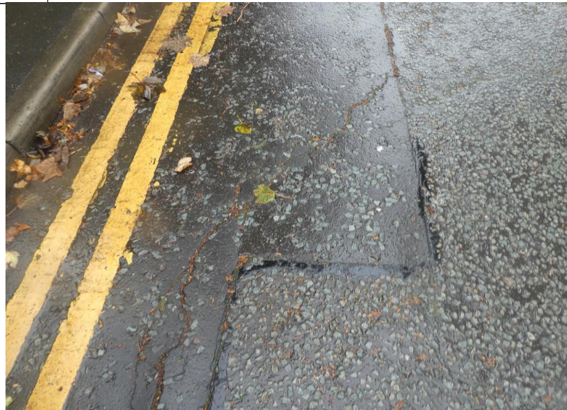
Photograph 36. Cracking to surfacing
