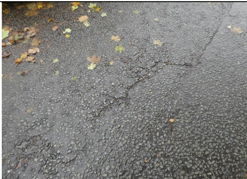
Photograph 78. Localised cracking to surfacing.
