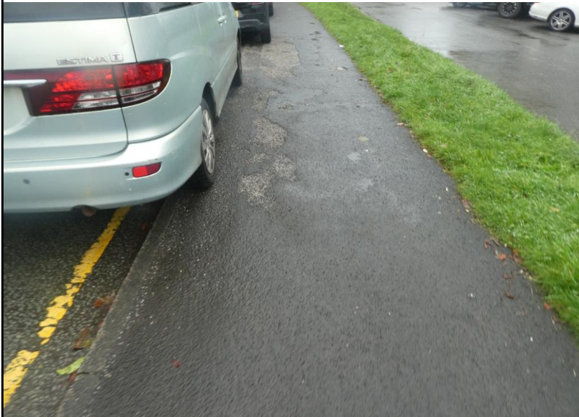
Photograph 67. Erosion to footpath
