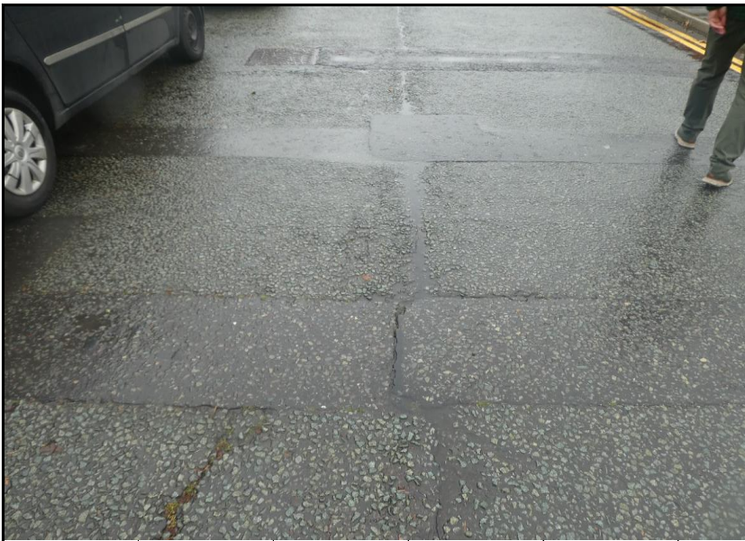
Photograph 53. Cracking to surfacing
