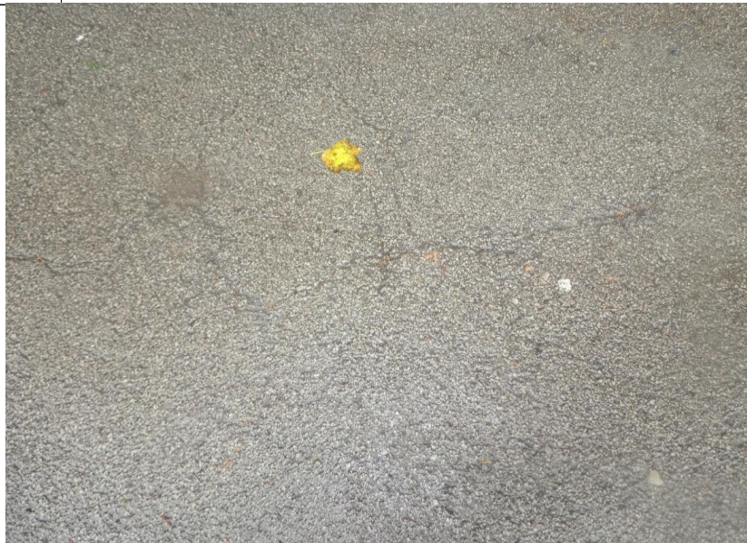
Photograph 20. Localised cracking to road surface
