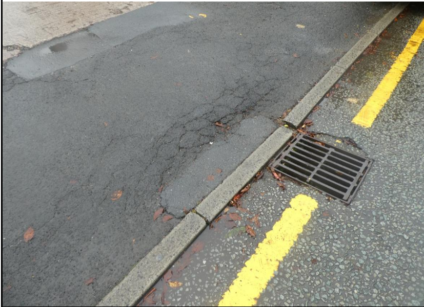
Photograph 63. Erosion to footpath surfacing of junction to business premises
