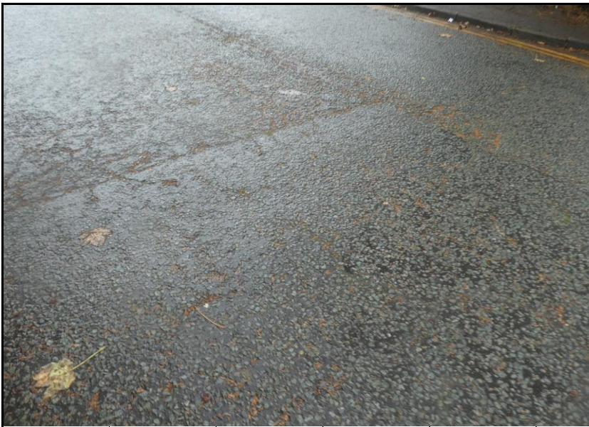
Photograph 37. Erosion of wearing coat of surfacing
