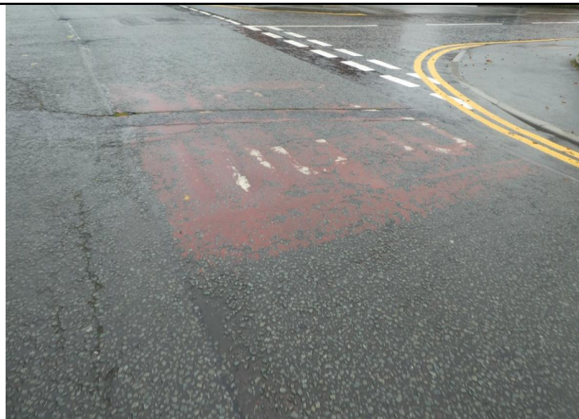
Photograph 46. Cracking to surfacing to centre of roadway.
