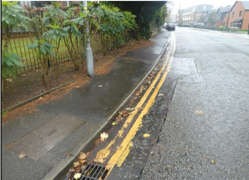
Photograph 35. Line marking eroding
