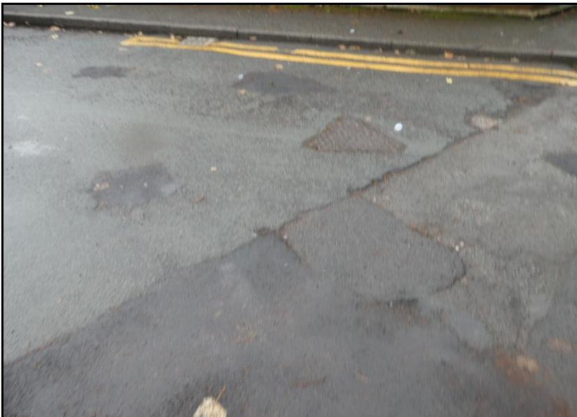
Photograph 17. Localised reinstatement of road surfacing to Norwood junction slightly eroded
