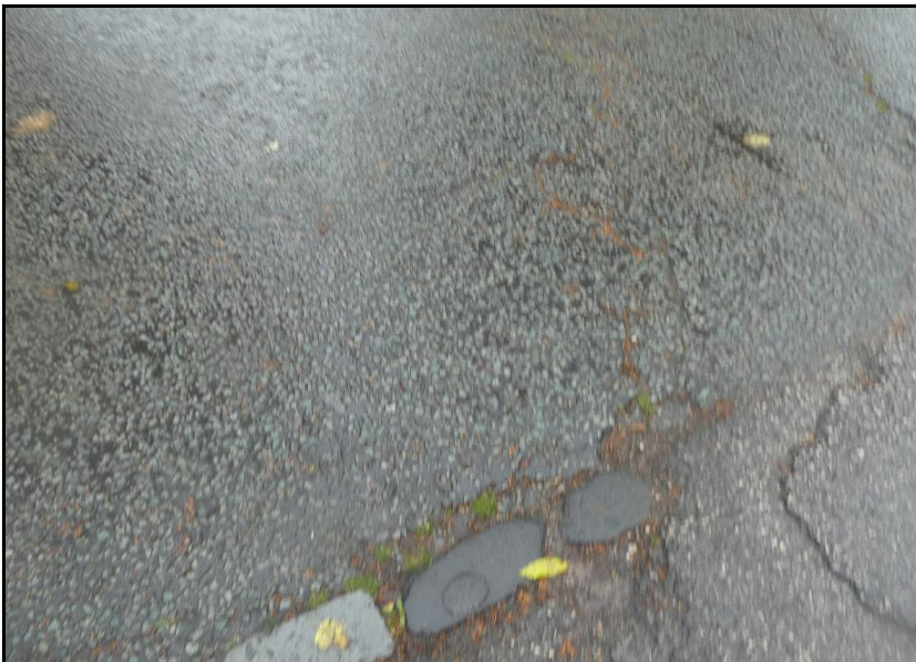
Photograph 33. Localised erosion to surfacing
