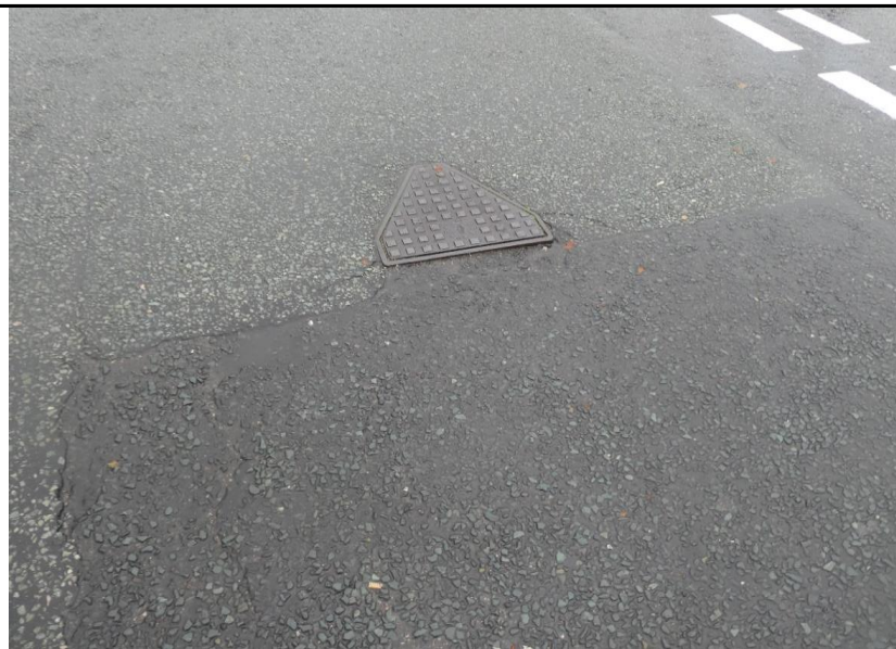
Photograph 90. Localised erosion to surfacing.
