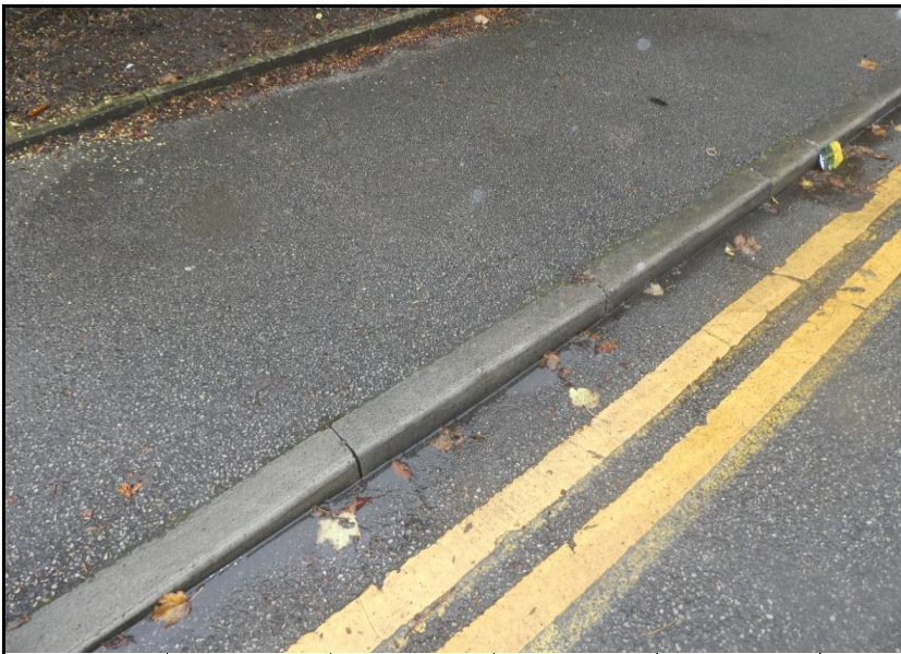
Photograph 29. Adjoining footpath in reasonable condition
