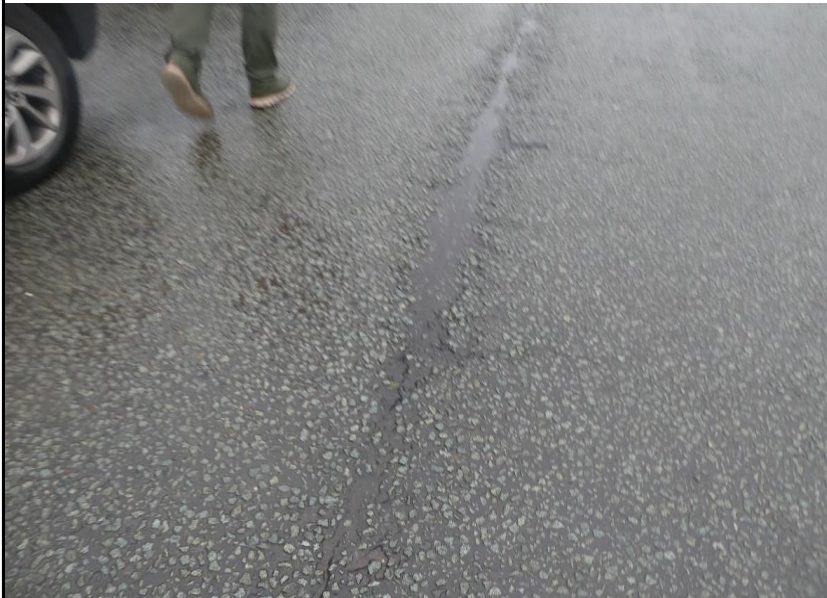
Photograph 59. Erosion to central section of roadway
