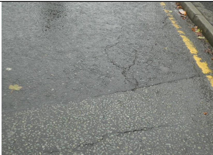
Photograph 82. Localised cracking to road surfacing.
