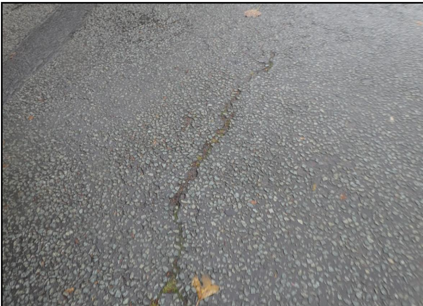
Photograph 49. Cracking and erosion to surfacing.
