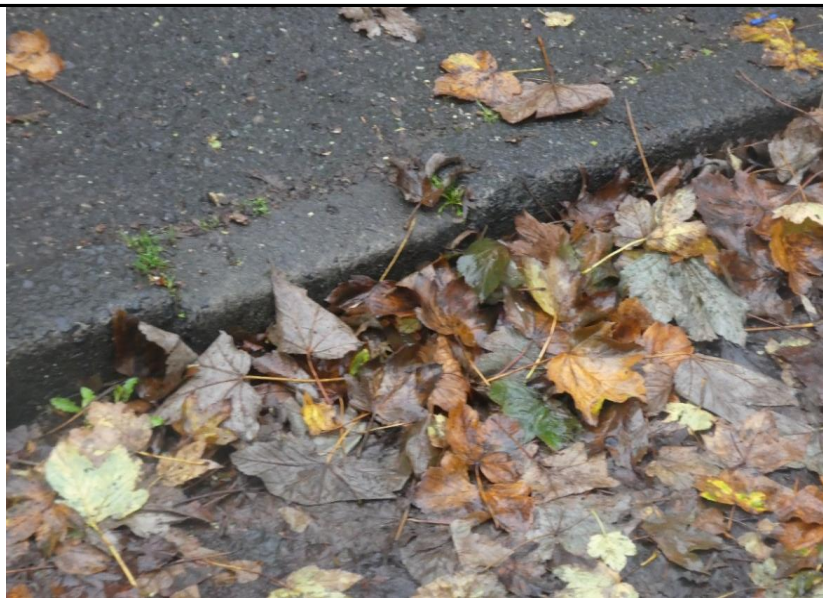
Photograph 74. Uneven kerbs to footpath
