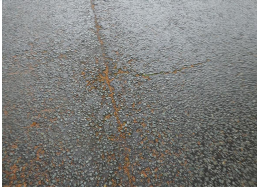
Photograph 40. Badly eroded and cracked surfacing.
