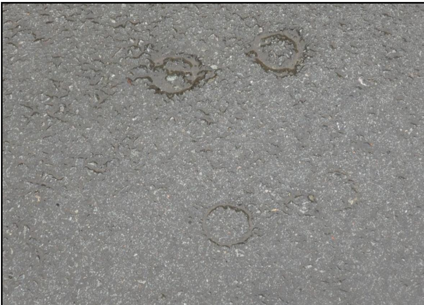
Photograph 9. Localised indentations to footpath areas
