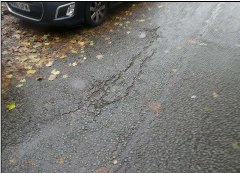
Photograph 77. Localised cracking to surfacing.
