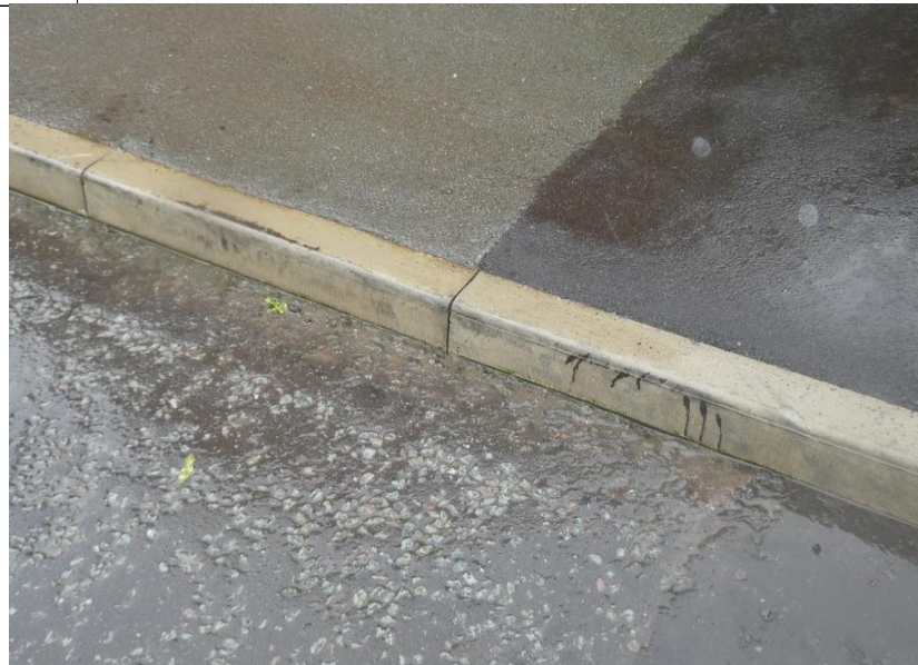
Photograph 8. Staining to the kerbing
