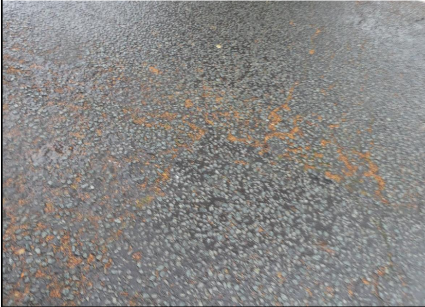
Photograph 39. Badly eroded and cracked surfacing.
