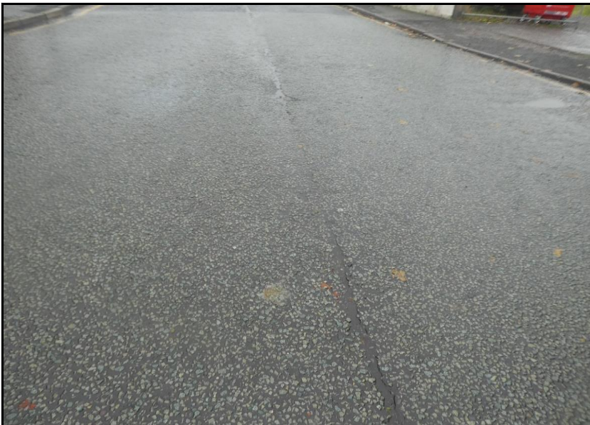
Photograph 81.Exposed joint to centre of roadway
