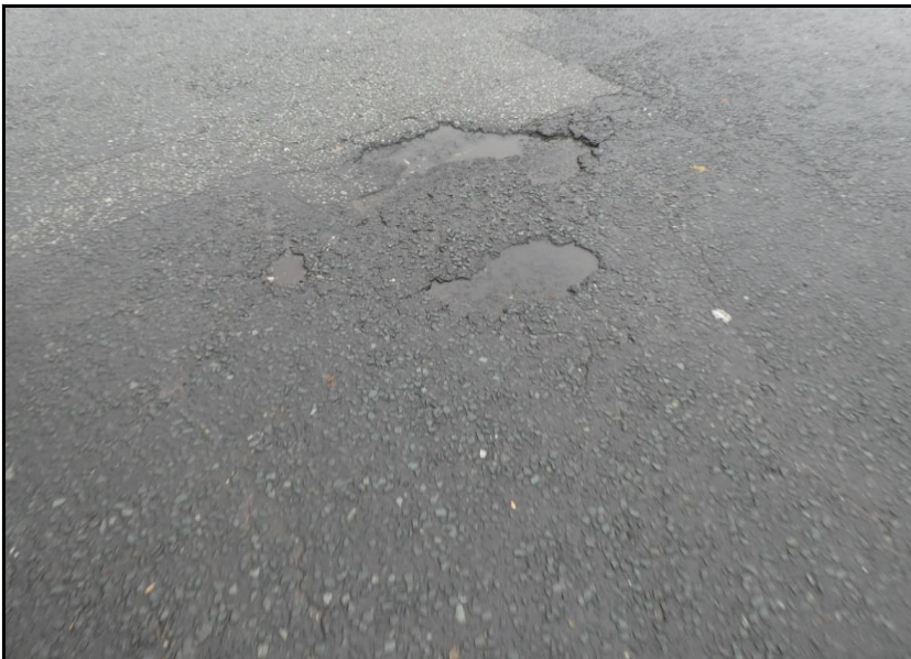
Photograph 89. Localised erosion to surfacing
