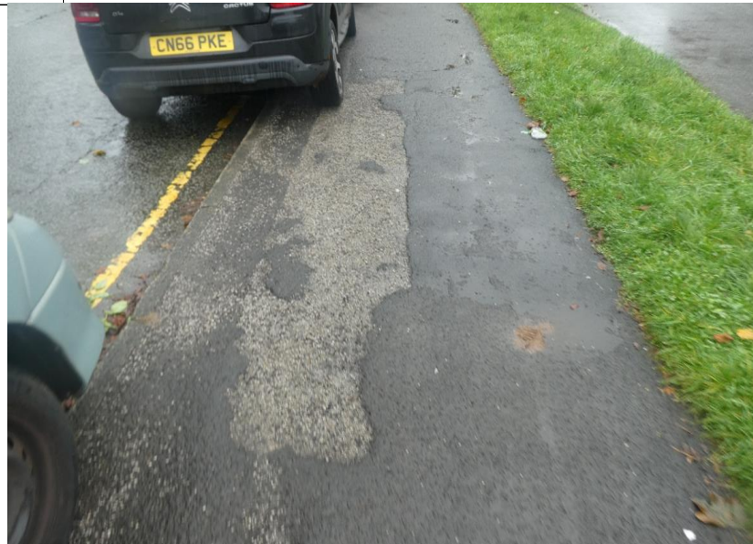
Photograph 68. Erosion to footpath
