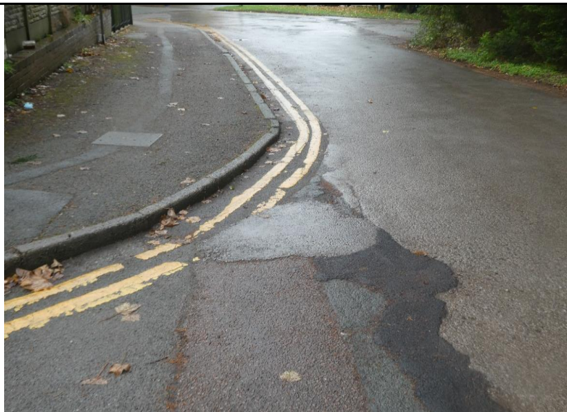
Photograph 18. Localised reinstatement of road surfacing to Norwood junction slightly eroded
