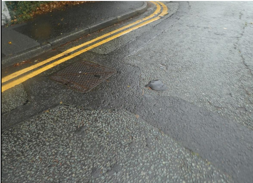
Photograph 47. Localised erosion to surfacing.
