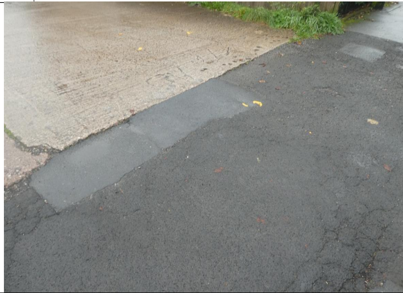
Photograph 64. Erosion to footpath surfacing of junction to business premises
