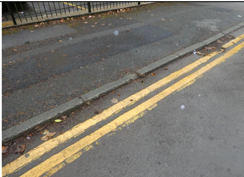
Photograph 22. Uneven and damaged kerb to George Street
