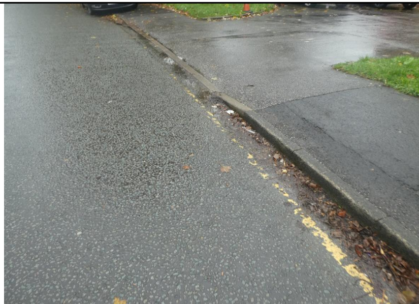
Photograph 70. Erosion to footpath
