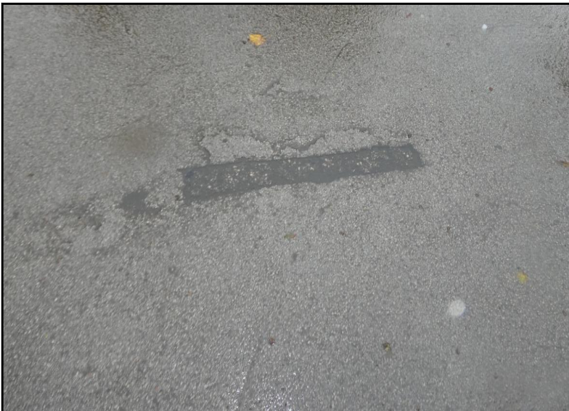
Photograph 25. Localised erosion to surfacing
