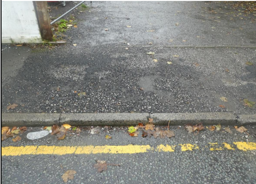
Photograph 83. Localised erosion to footpath
