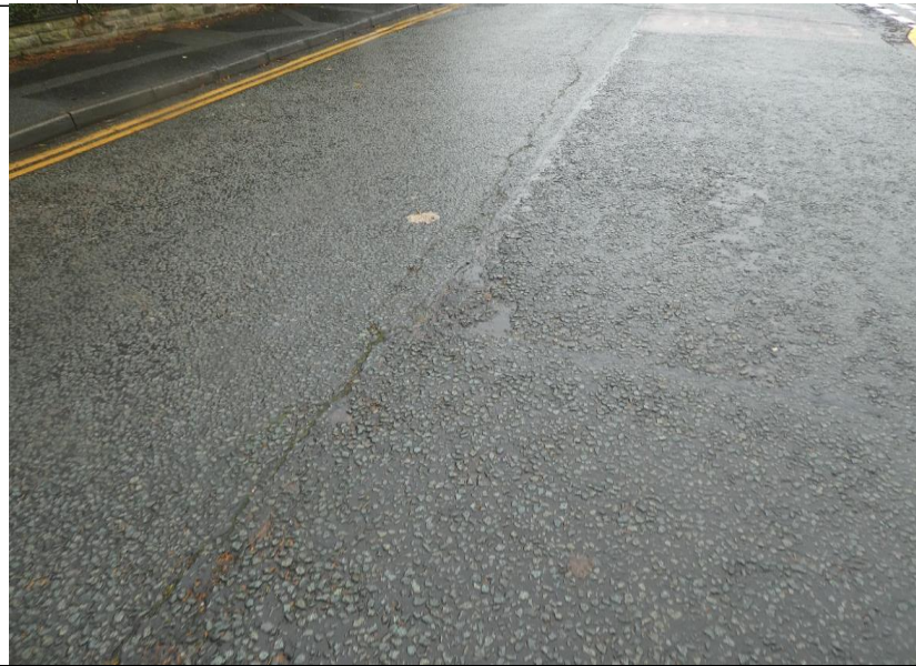
Photograph 44. Cracking to surfacing to centre of roadway.
