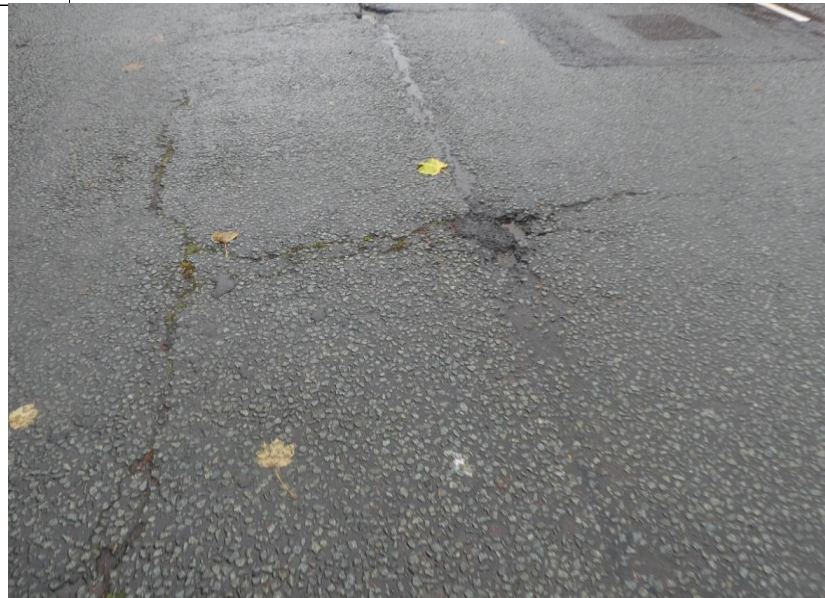
Photograph 48. Cracking and erosion to surfacing.
