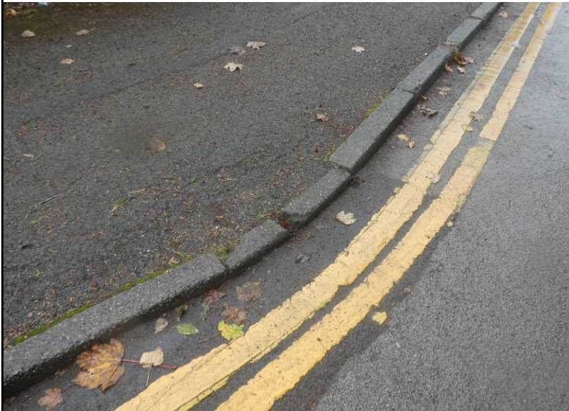
Photograph 19. Damaged and uneven kerbs to Norwood junction
