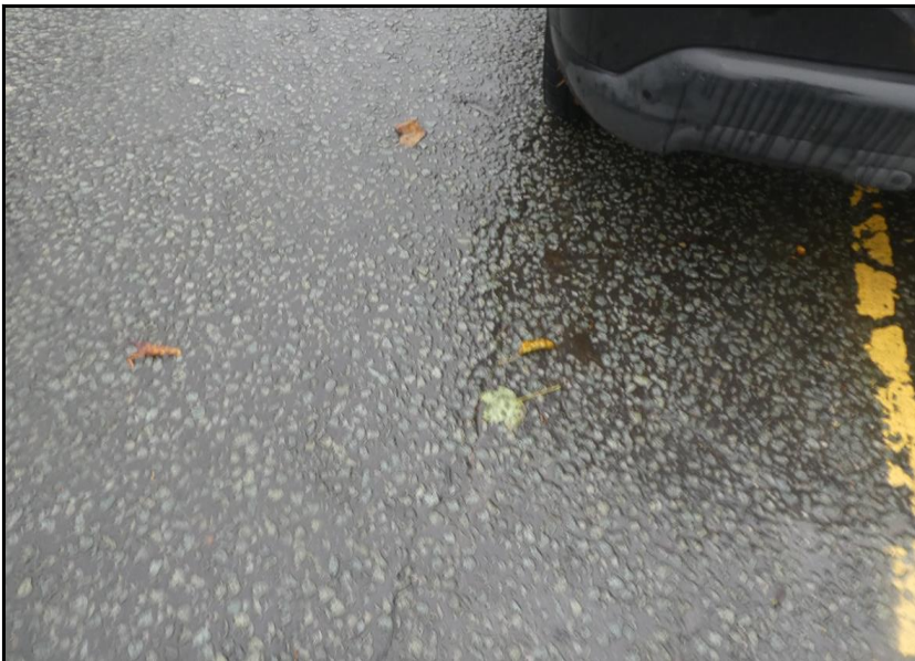
Photograph 69. Cracking to surfacing
