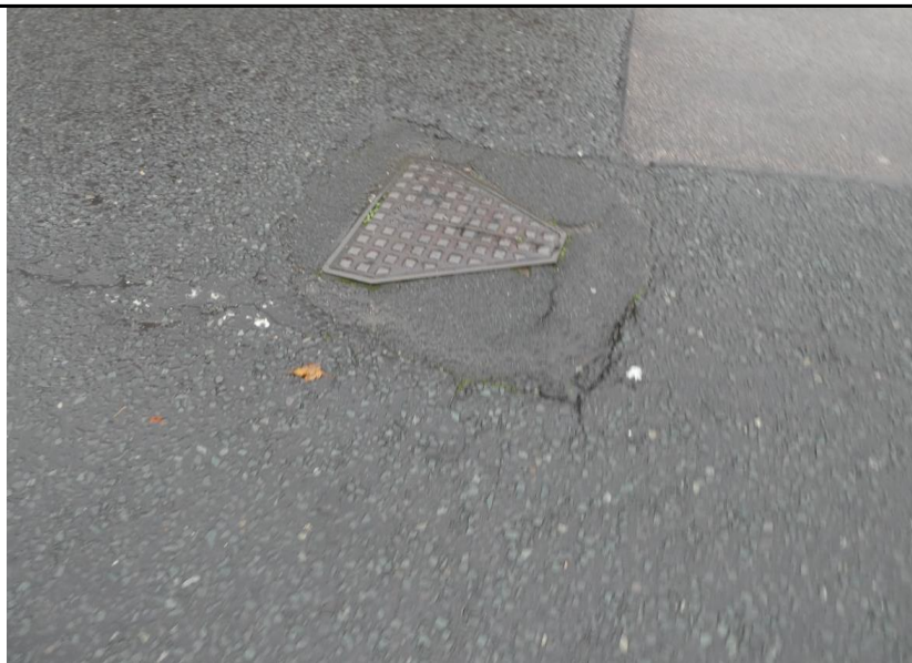
Photograph 86. Erosion to surfacing around inspection chamber.
