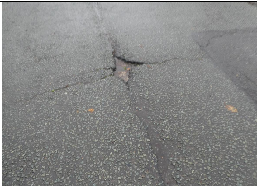
Photograph 50. Cracking and erosion to surfacing.
