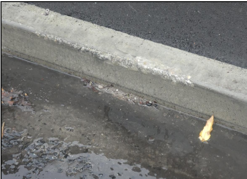
Photograph 5. Localised impact damage to the kerbs
