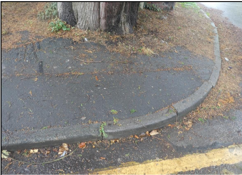
Photograph 41. Damaged and uneven kerbing.
