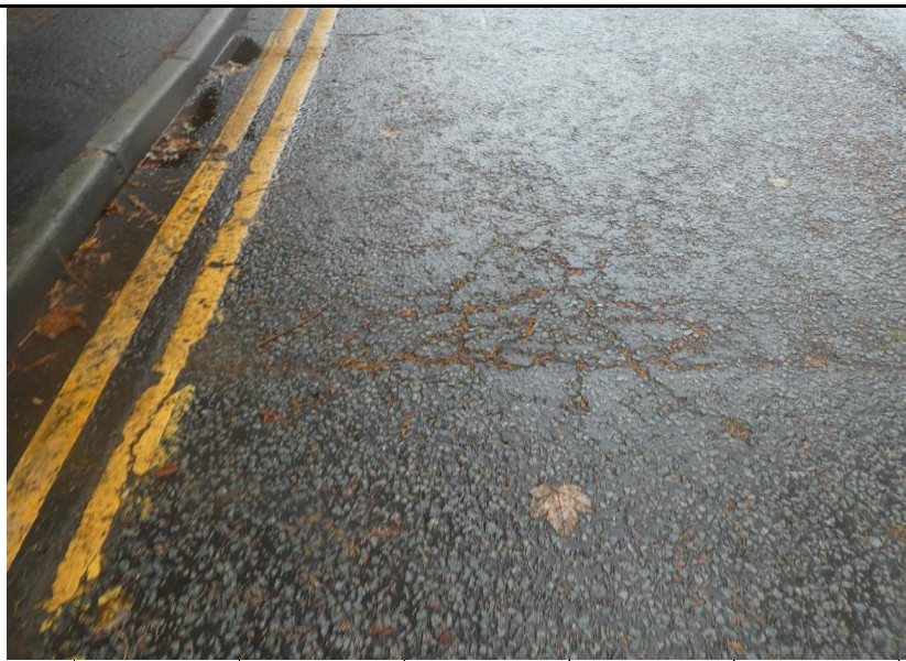
Photograph 38. Badly eroded and cracked surfacing
