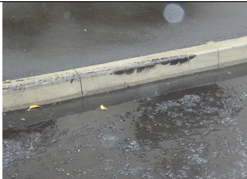
Photograph 6. Staining the kerbing
