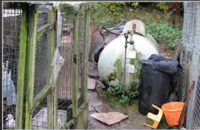
Poorly-sited tank with clutter around it
