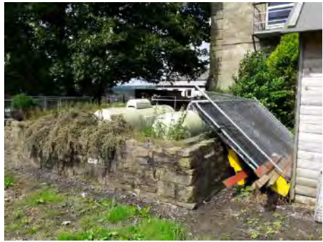
Photograph 3 (P3) Above ground propane tanks.
