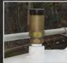
Pressure release valve
