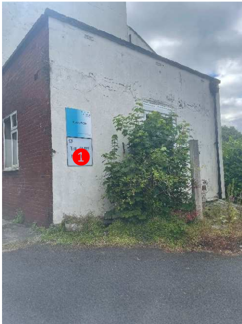
Site Notice No. ① posted on gable end of building
