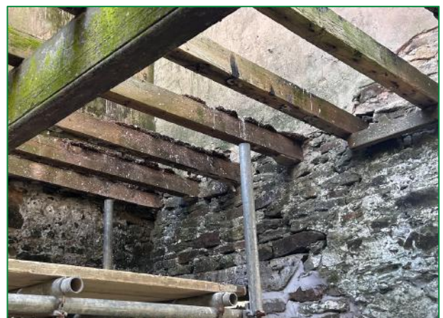
Showing evidence of roosting on the beams in the structure
