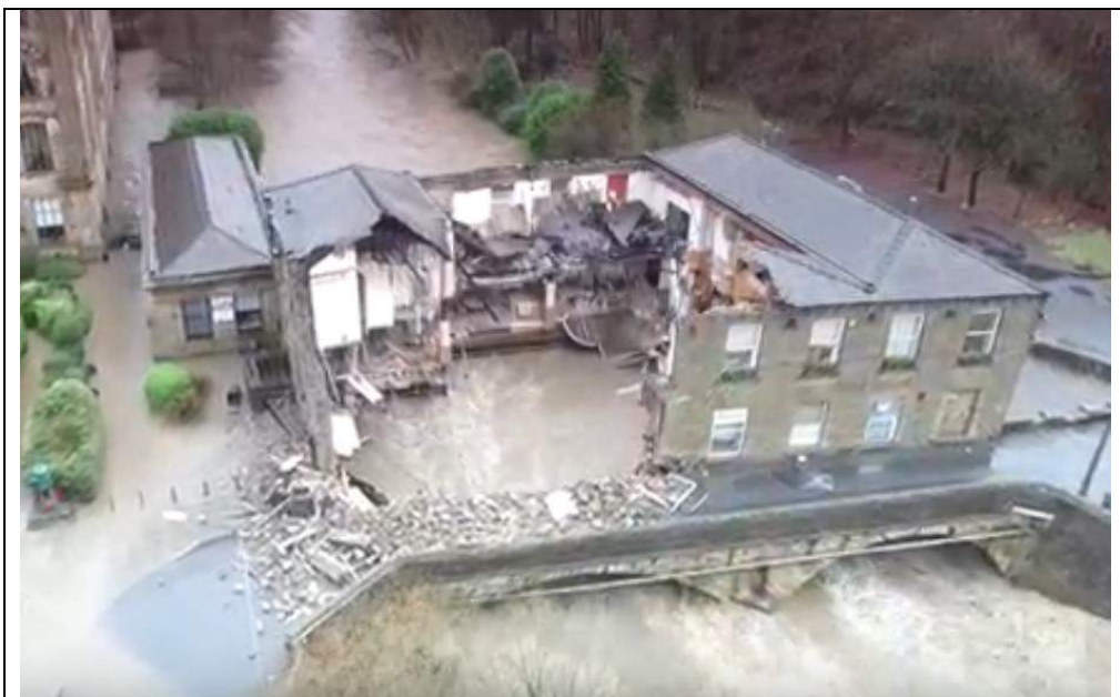
Figure 4: Kay Street Bridge during 2015 flood event
