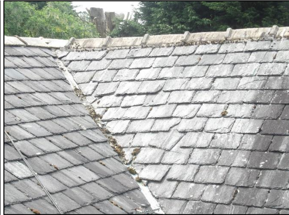
Figure 25: Areas of slipped roof tiles.
