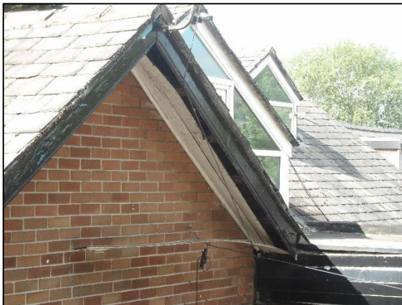
Figure 20: Missing woodwork on the soffits of the building.
