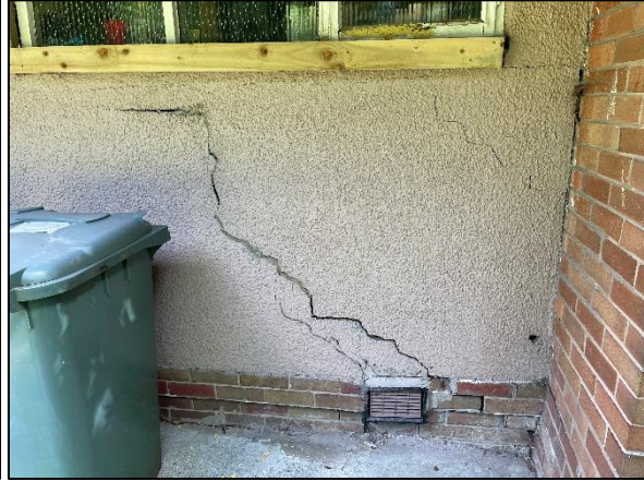
Figure 19: Cracks in the southern elevation.
