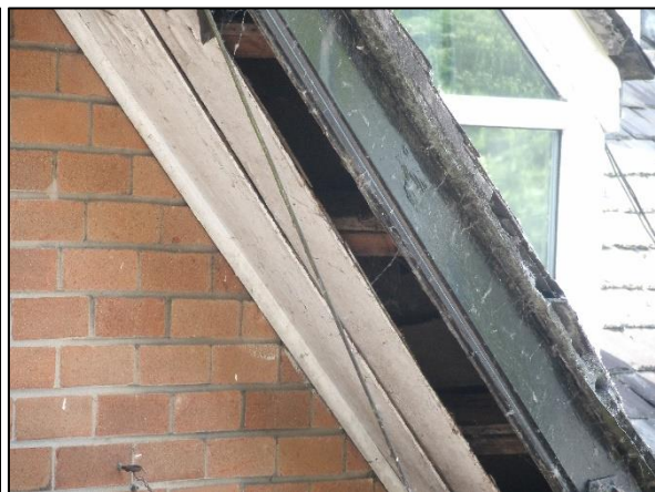
Figure 23: Missing cement in the northern elevation.
