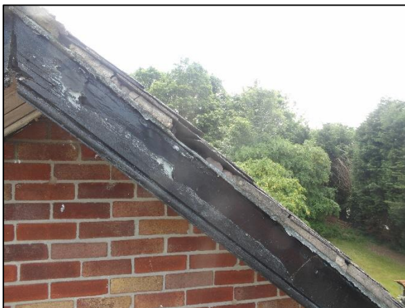
Figure 22: Missing cement in the western elevation.
