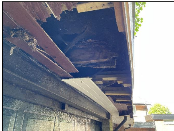
Figure 21: Extensive voids around the garage.
