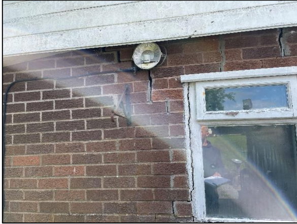
Figure 18: The cracks in the single storey areas of the building.
