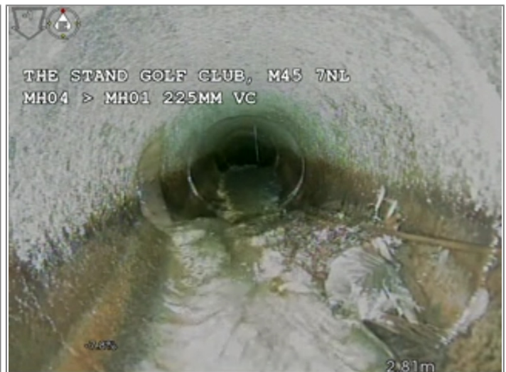
Roots mass 15% cross-sectional area loss at joint
