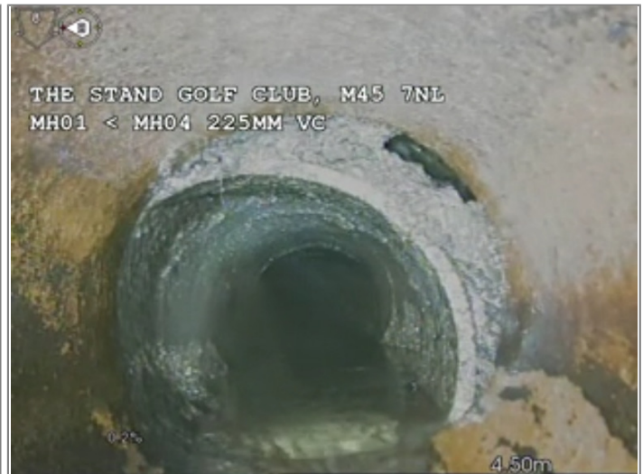
Joint displaced large
