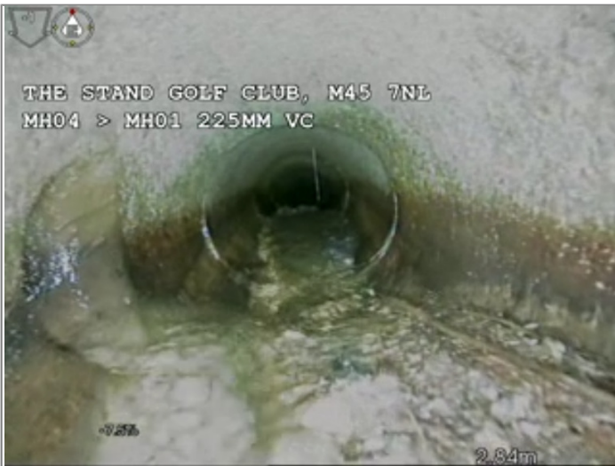
Junction at 09 o'clock, diameter 100mm
