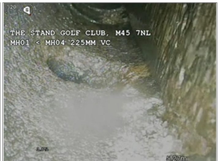
Junction at 09 o'clock, diameter 100mm
