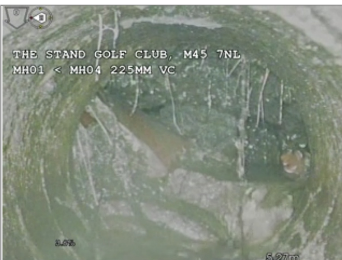
Collapsed drain/sewer 95% - Remark: PLEASE NOTE COLLAPSED DRAIN IS APPROX 3-5M FROM CCTV
