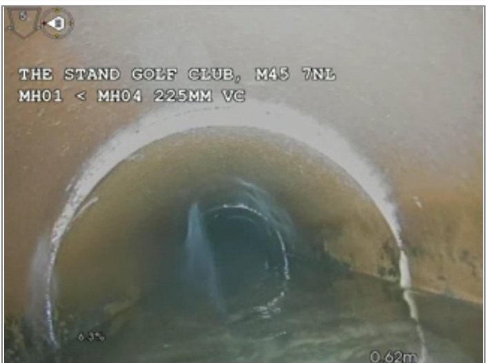
Joint displaced medium
