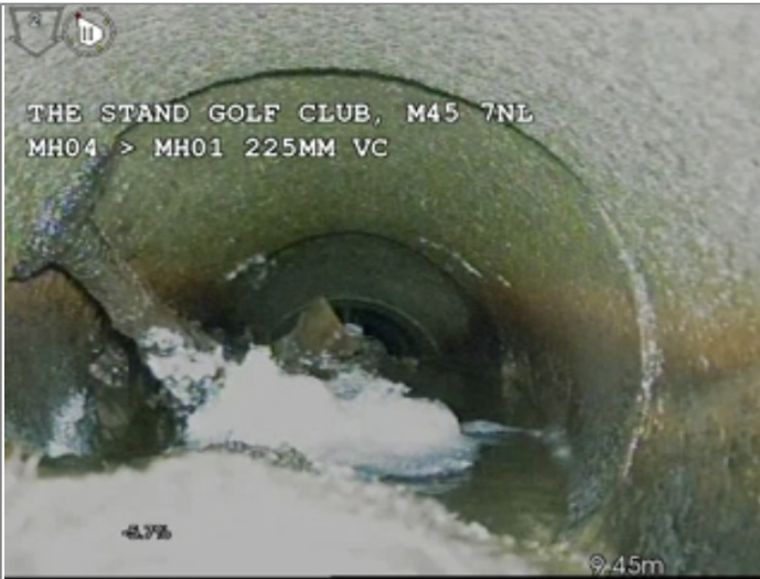
Roots tap at joint
