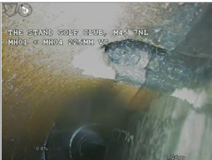
Junction at 03 o'clock, diameter 100mm
