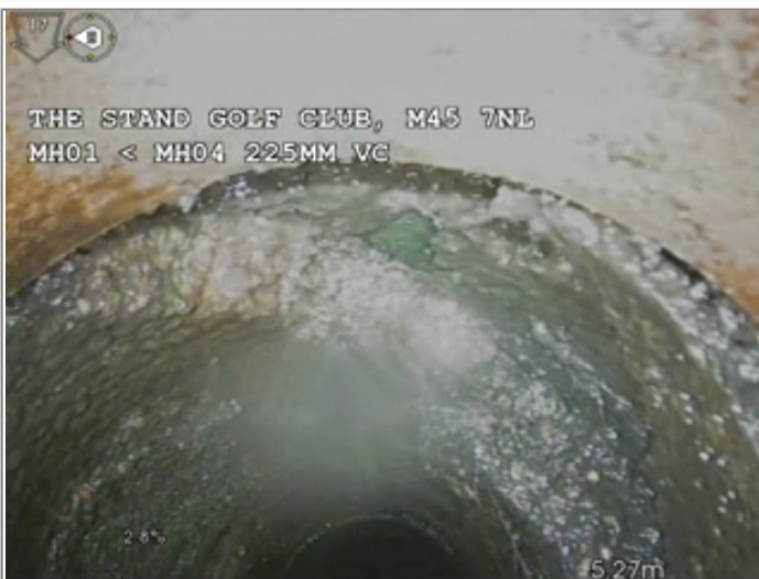
Infiltration running at 12 o'clock at joint
