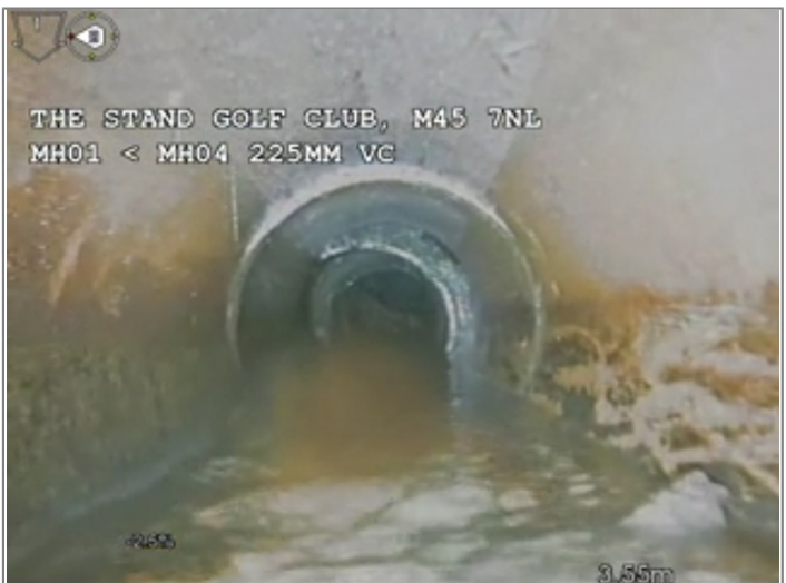
Attached deposits, encrustation from 04 to 08 o'clock 25% cross-sectional area loss, Finished
