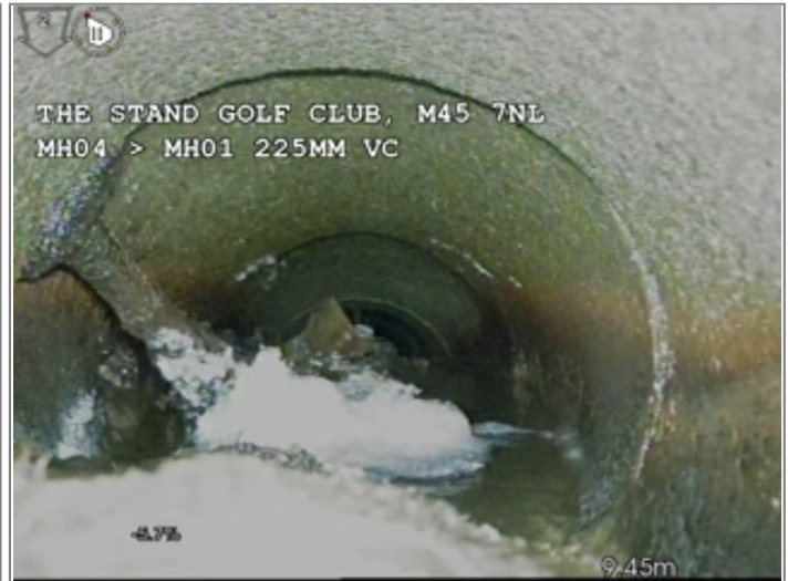
Survey abandoned - Remark: SA DUE TO ROOTS MASS 50% UNABLE TO PASS
