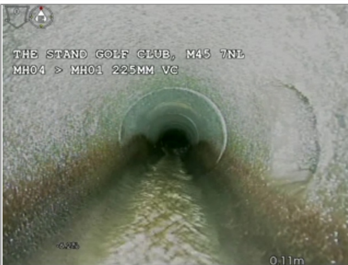
Junction at 03 o'clock, diameter 100mm
