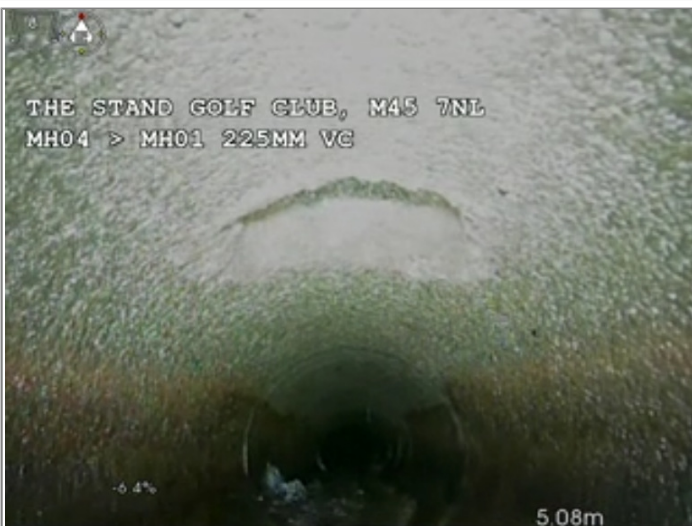
Junction at 12 o'clock, diameter 100mm
