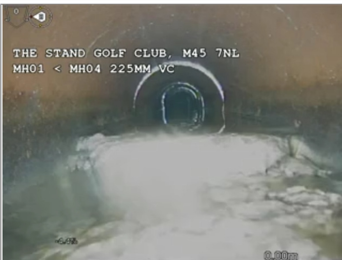
Attached deposits, encrustation from 04 to 08 o'clock 25% cross-sectional area loss, Start
