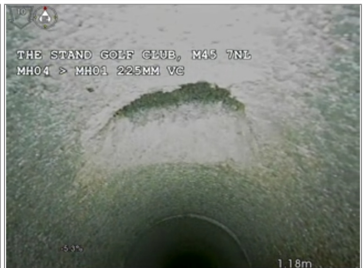
Junction at 12 o'clock, diameter 100mm
