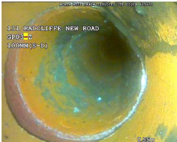
1, 00:00:17, 0.55 m Joint displaced, medium
