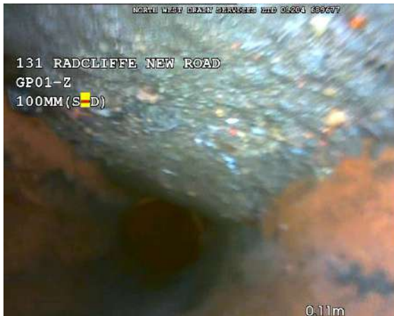
1, 00:00:15, 0.11 m Settled deposits, fine, 20% cross-sectional area loss, start
