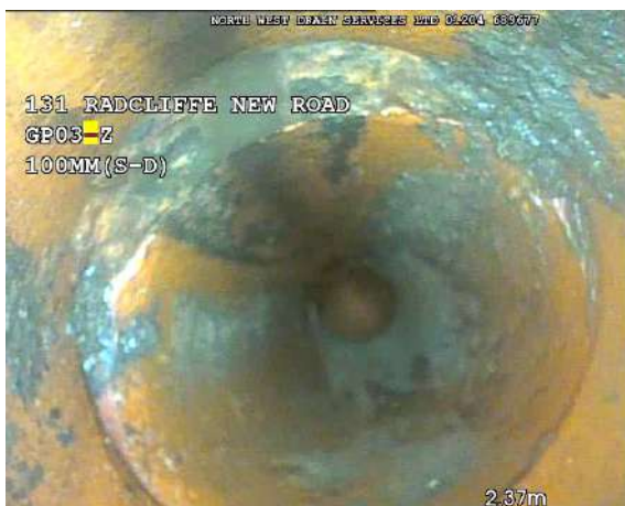
3, 00:00:38, 2.37 m Joint displaced, large
