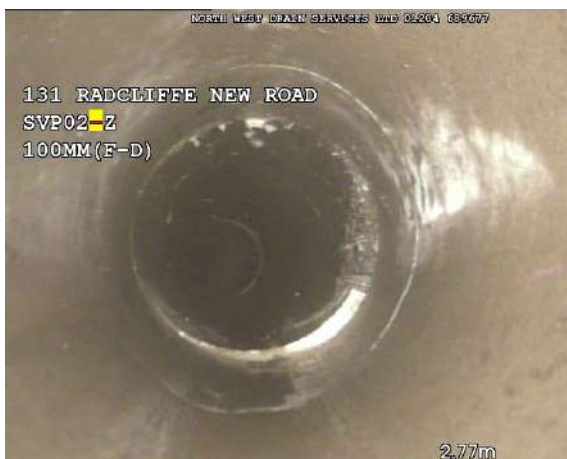
3, 00:00:24, 2.77 m Crack, circumferential from 12 o'clock to 12 o'clock
