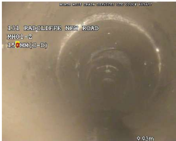
1, 00:00:58, 9.93 m Joint displaced, medium
