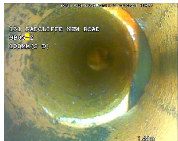
4, 00:00:23, 1.44 m Joint displaced, large
