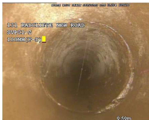
2, 00:00:59, 9.59 m Joint displaced, medium
