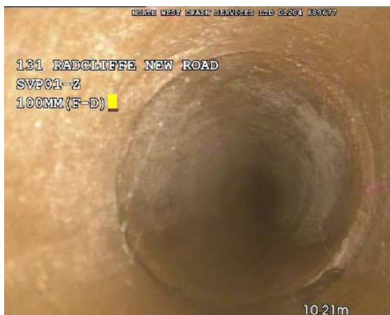
3, 00:01:03, 10.21 m Joint displaced, medium
