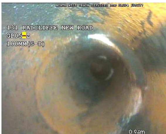
3, 00:00:18, 0.94 m Joint displaced, medium
