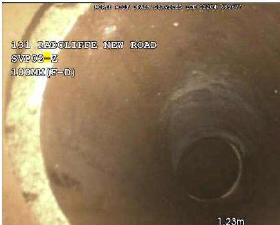
1, 00:00:13, 1.23 m Joint displaced, large
