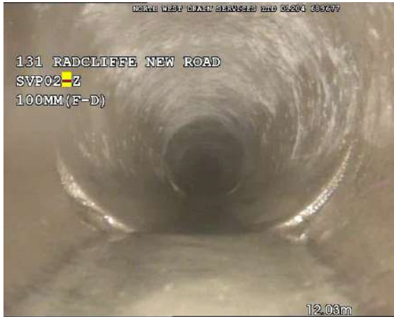
9, 00:01:17, 12.03 m Joint displaced, medium
