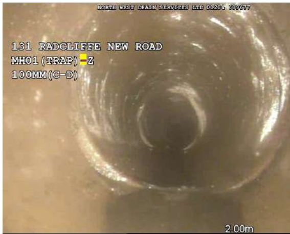
1, 00:00:10, 2.00 m Joint displaced, medium
