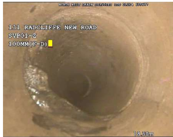
8, 00:02:15, 18.30 m Attached deposits, encrustation at joint from 5 o'clock to 10 o'clock, 20% cross-sectional area loss
