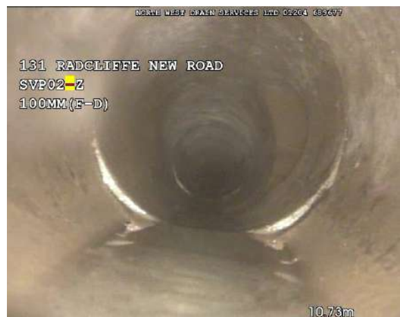
8, 00:01:10, 10.73 m Joint displaced, medium
