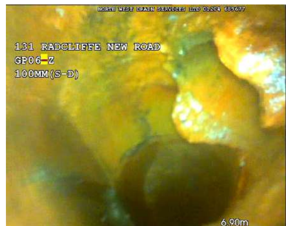
8, 00:01:05, 6.90 m Connection other than junction at 12 o'clock, 100mm dia
