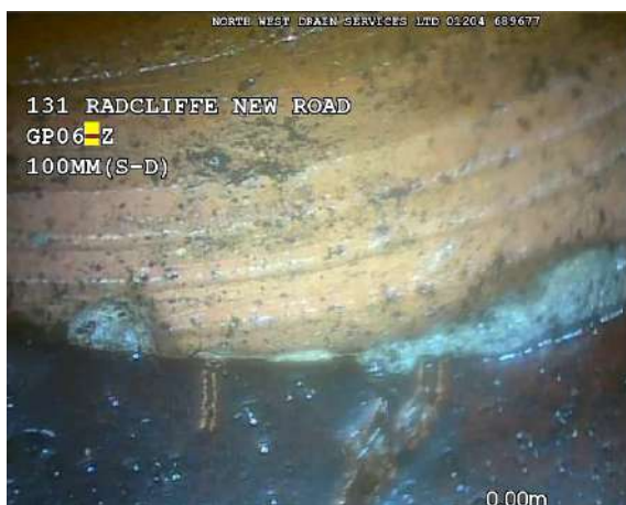
1, 00:00:00, 0.00 m Joint displaced, large
