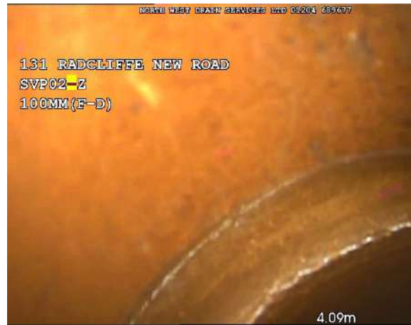
6, 00:00:36, 4.09 m Joint displaced, large
