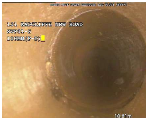
4, 00:01:08, 10.81 m Joint displaced, medium
