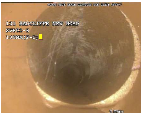
1, 00:00:54, 9.05 m Joint displaced, large
