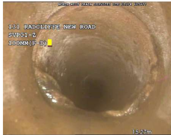
6, 00:01:48, 15.27 m Attached deposits, encrustation at joint from 3 o'clock to 9 o'clock, 15% cross-sectional area loss
