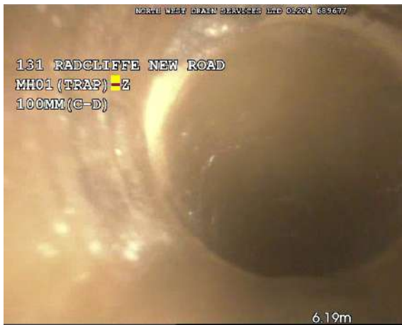
3, 00:00:33, 6.19 m Joint displaced, large
