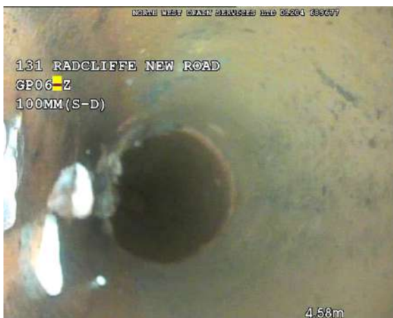
7, 00:00:47, 4.58 m Settled deposits, coarse, 5% cross-sectional area loss
