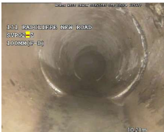
7, 00:01:06, 10.21 m Joint displaced, medium
