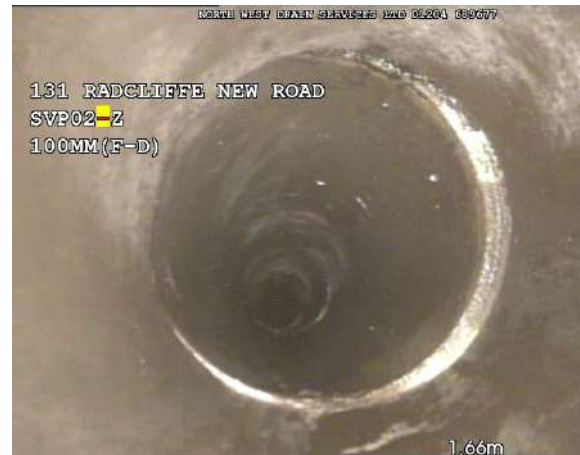
2, 00:00:17, 1.66 m Joint displaced, medium
