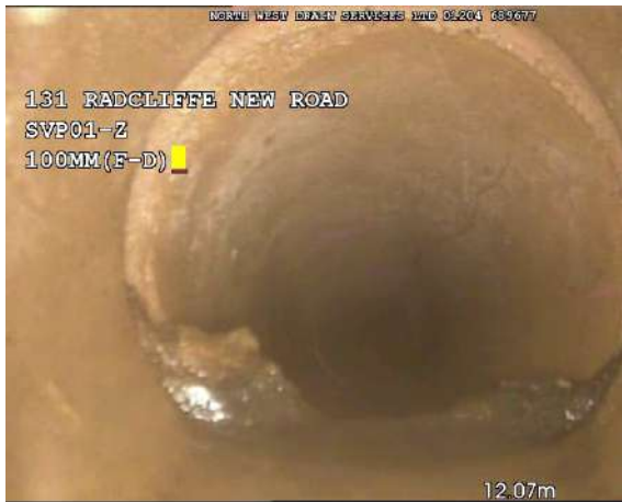
5, 00:01:21, 12.07 m Attached deposits, encrustation at joint from 4 o'clock to 8 o'clock, 15% cross-sectional area loss
