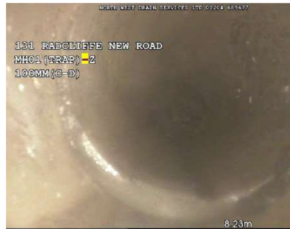
4, 00:00:45, 8.23 m Joint displaced, medium
