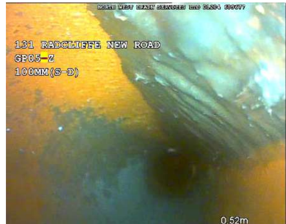
2, 00:00:11, 0.52 m Settled deposits, fine, 10% cross-sectional area loss, start
