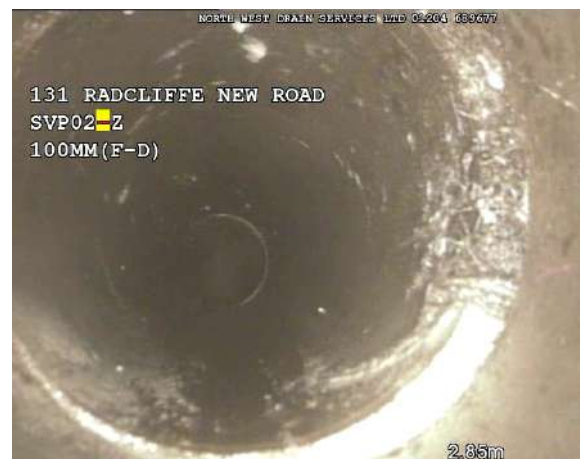
4, 00:00:28, 2.85 m Joint displaced, medium
