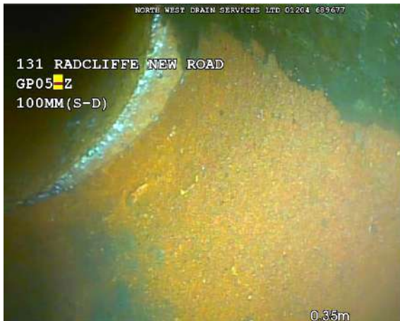
1, 00:00:07, 0.35 m Joint displaced, medium
