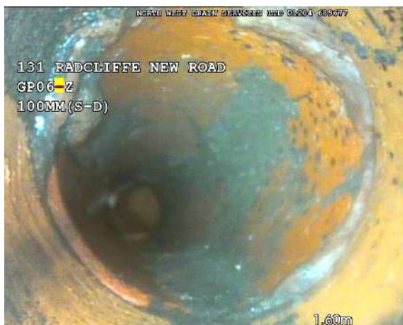
3, 00:00:20, 1.60 m Attached deposits, encrustation at joint from 12 o'clock to 12 o'clock, 10% cross-sectional area loss
