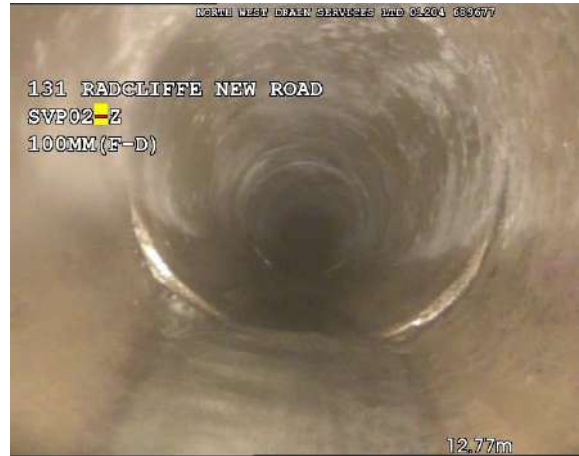
10, 00:01:20, 12.77 m Joint displaced, medium
