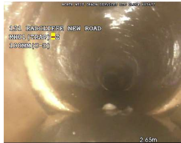
2, 00:00:14, 2.65 m Joint displaced, large
