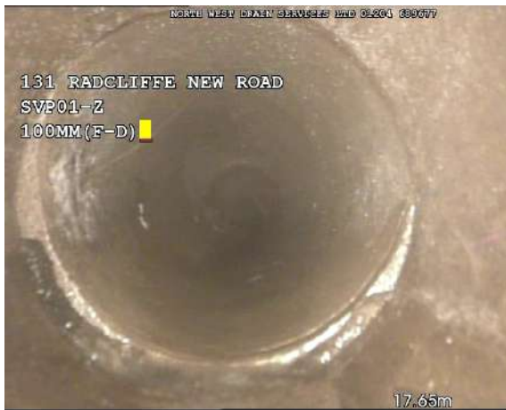
7, 00:02:09, 17.65 m Joint displaced, large
