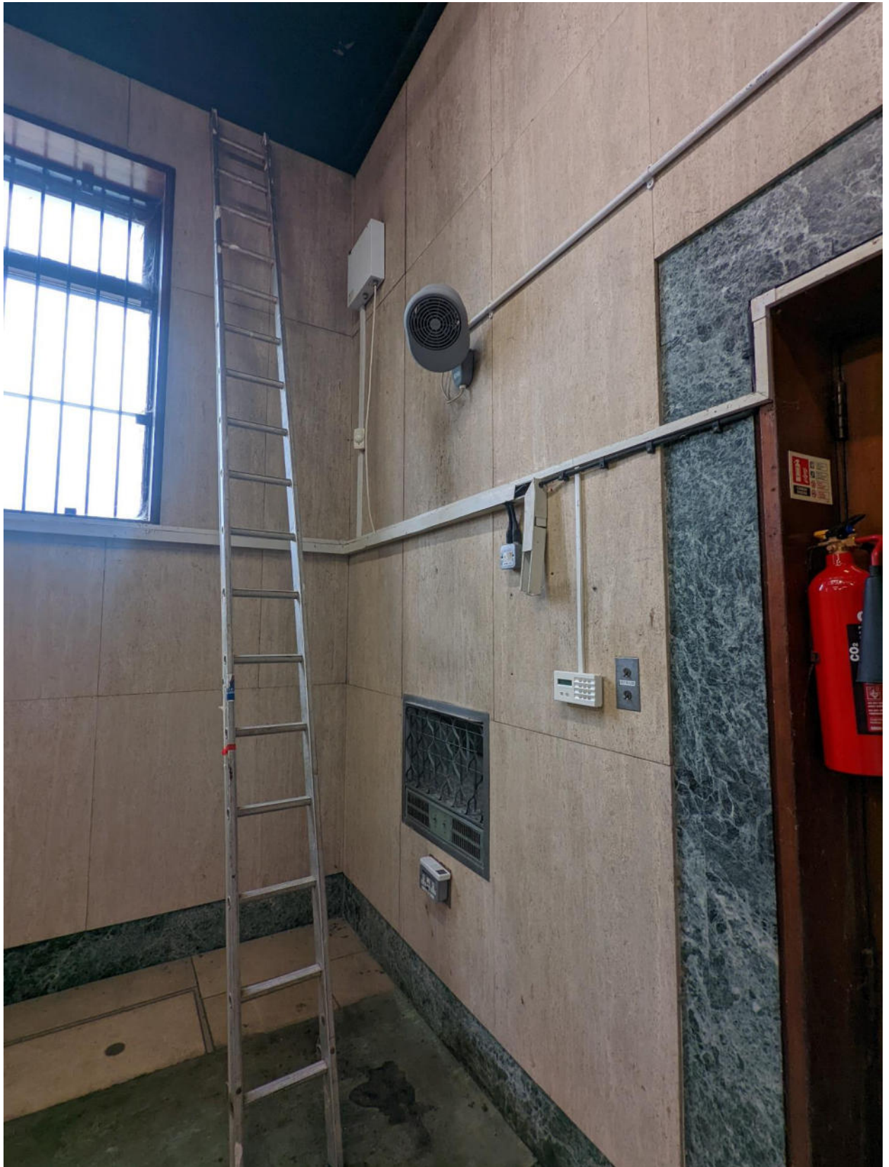
Plate 28: View of internal heating system and window security bars of Heaton Park Reservoir Pumping Station (4).
