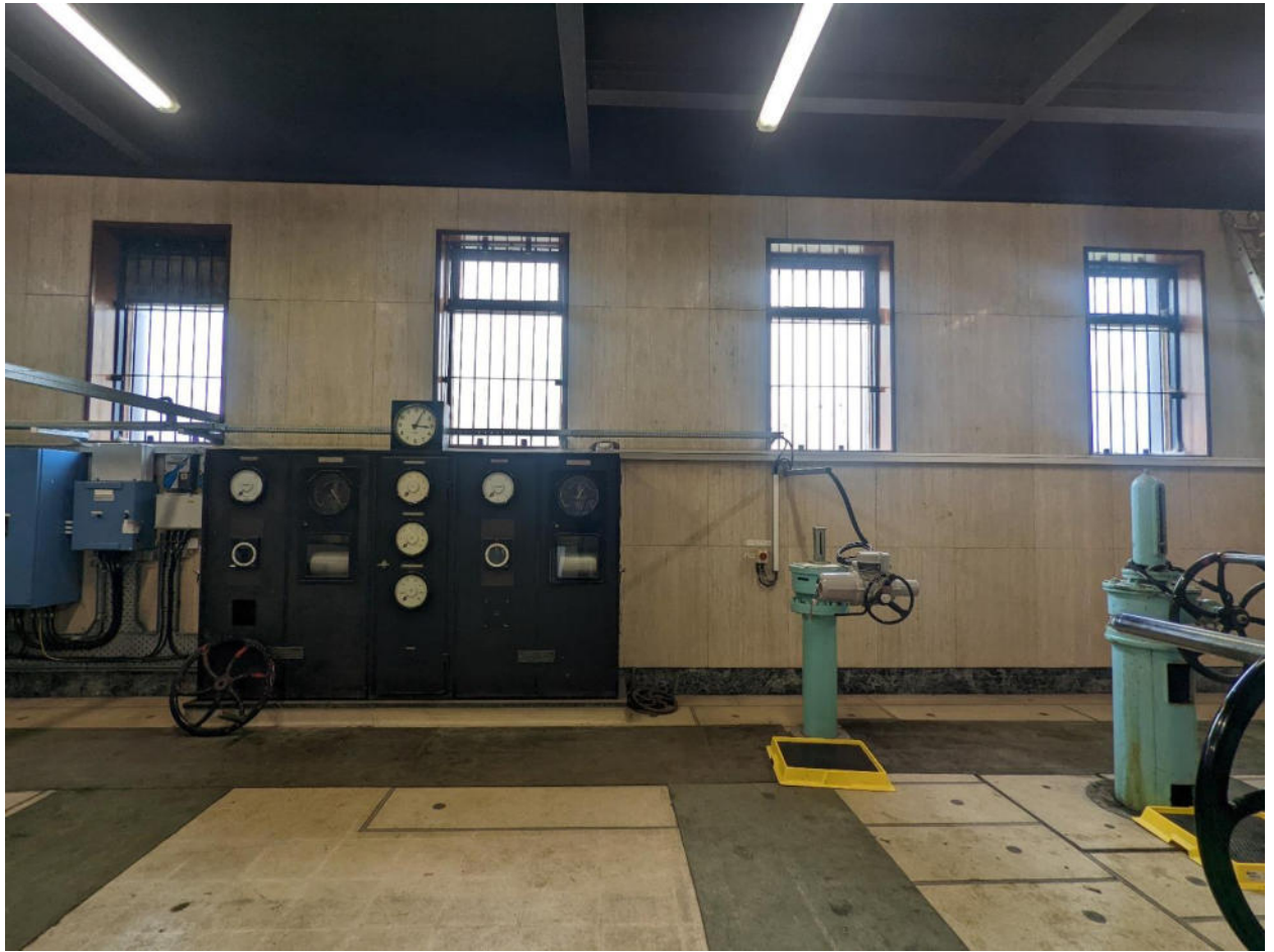
Plate 29: Interior view of windows on south-east elevation and interior controls of Heaton Park Reservoir Pumping Station (4).
