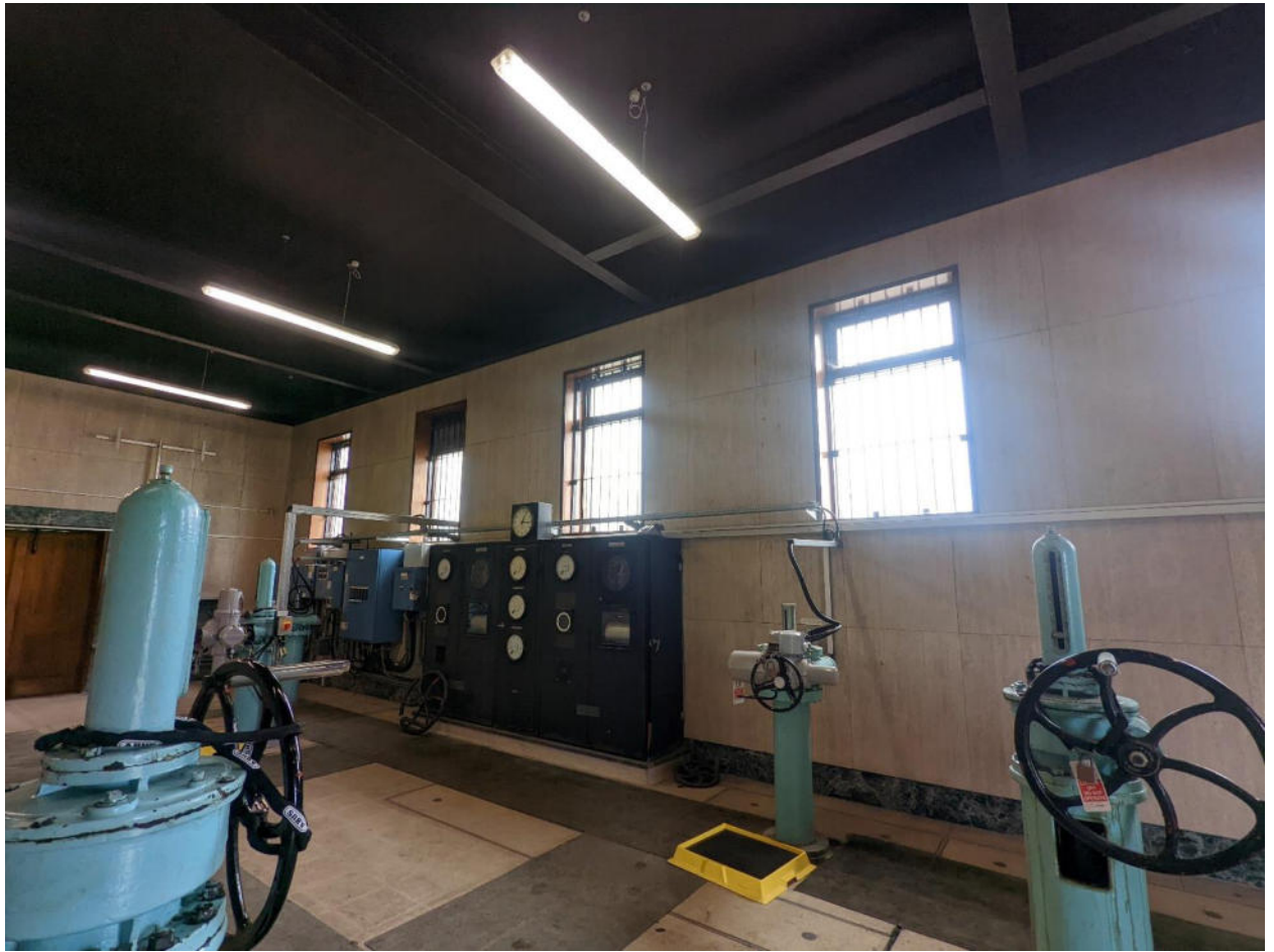
Plate 33: View of interior lighting, windows and security bars and controls of Heaton Park Reservoir Pumping Station (4).
