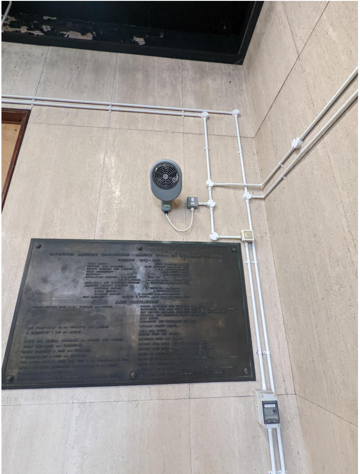
Plate 31: View of internal heating system of Heaton Park Reservoir Pumping Station (4).
