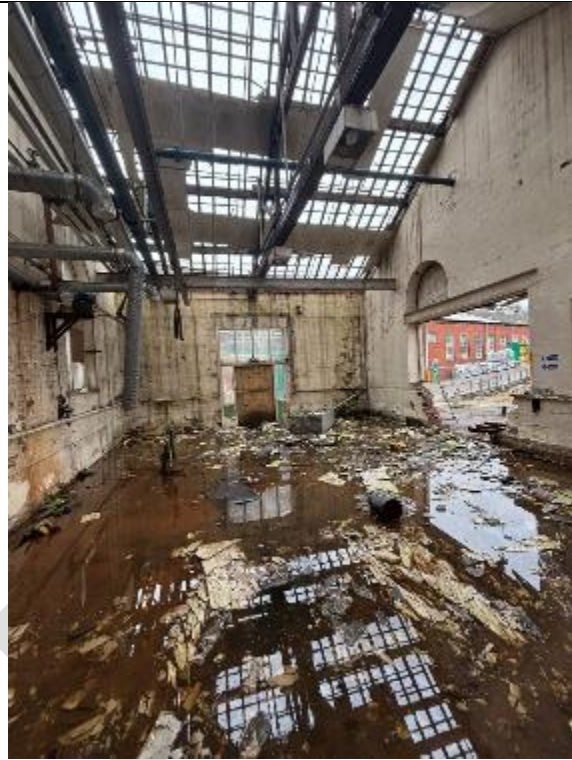
Photograph 14: View of flooded interior of the structure.
