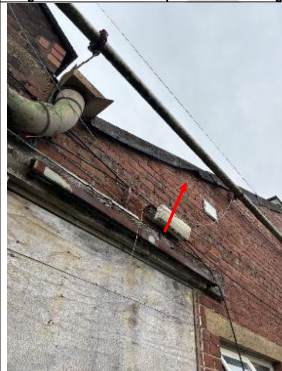
Photograph 3: View of the raised lead flashing along the southern elevation (PRF1).
