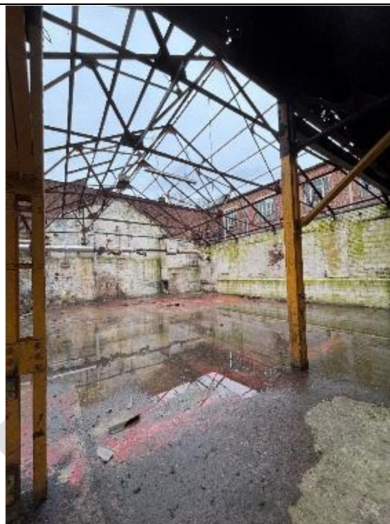
Photograph 10: View of the entire roof missing within the northwestern section.
