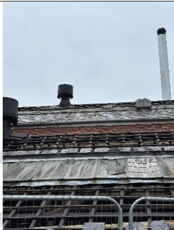
Photograph 2: View of the southwestern elevation. Large areas of the roof exposed and missing.
