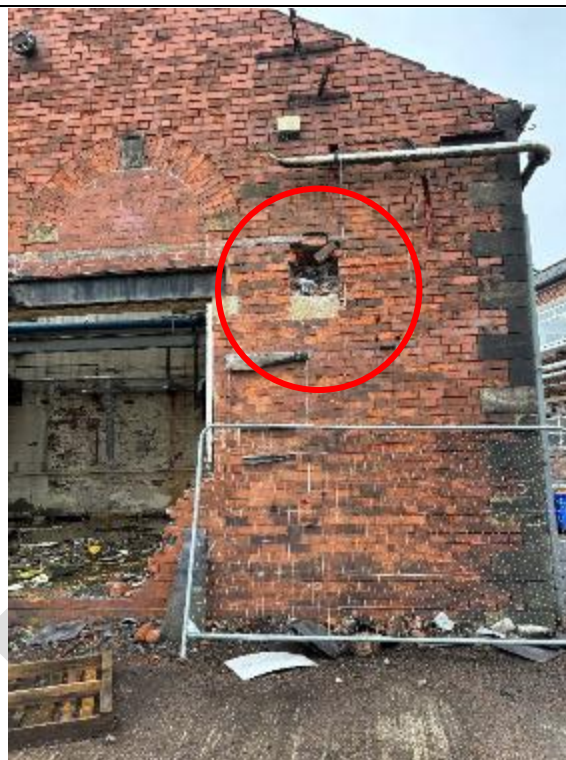
Photograph 6: View of large holes in the damaged wall along the southern elevation (PRF2).
