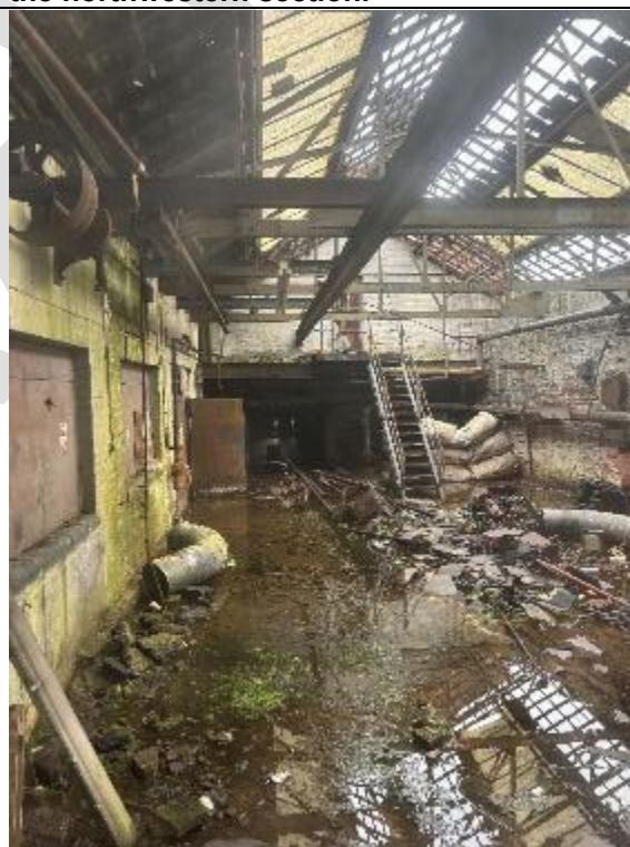
Photograph 12: View of the internal area of the western section of the building. Interior was flooded and damp throughout.
