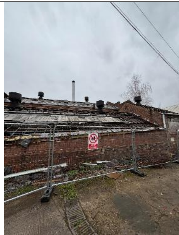
Photograph 1: View of the southwestern elevation. Large areas of the roof exposed and missing.
