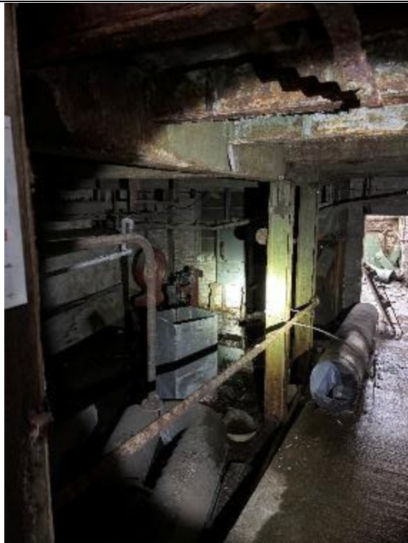
Photograph 13: View of the cellar which was damp throughout.
