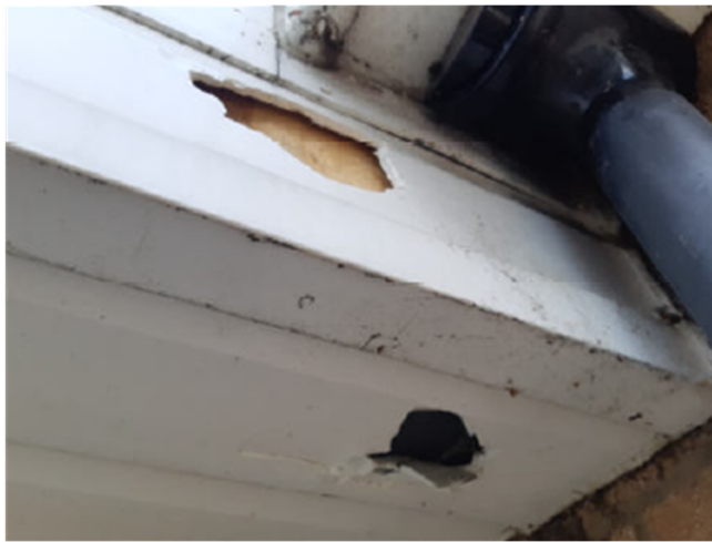
Photograph 3: B1 - Holes in cladding.
