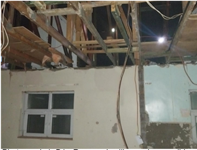
Photograph 1: B1 - Removed ceiling and accessible loft cavity. Light can be seen coming in through holes in the cladding.
