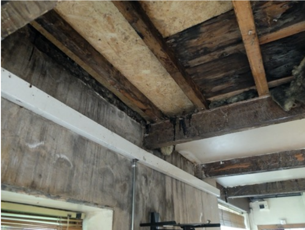
Photo, collapsed ceiling under flat roof section
