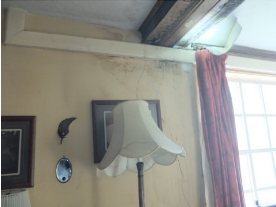
Photo, cracking under beams
