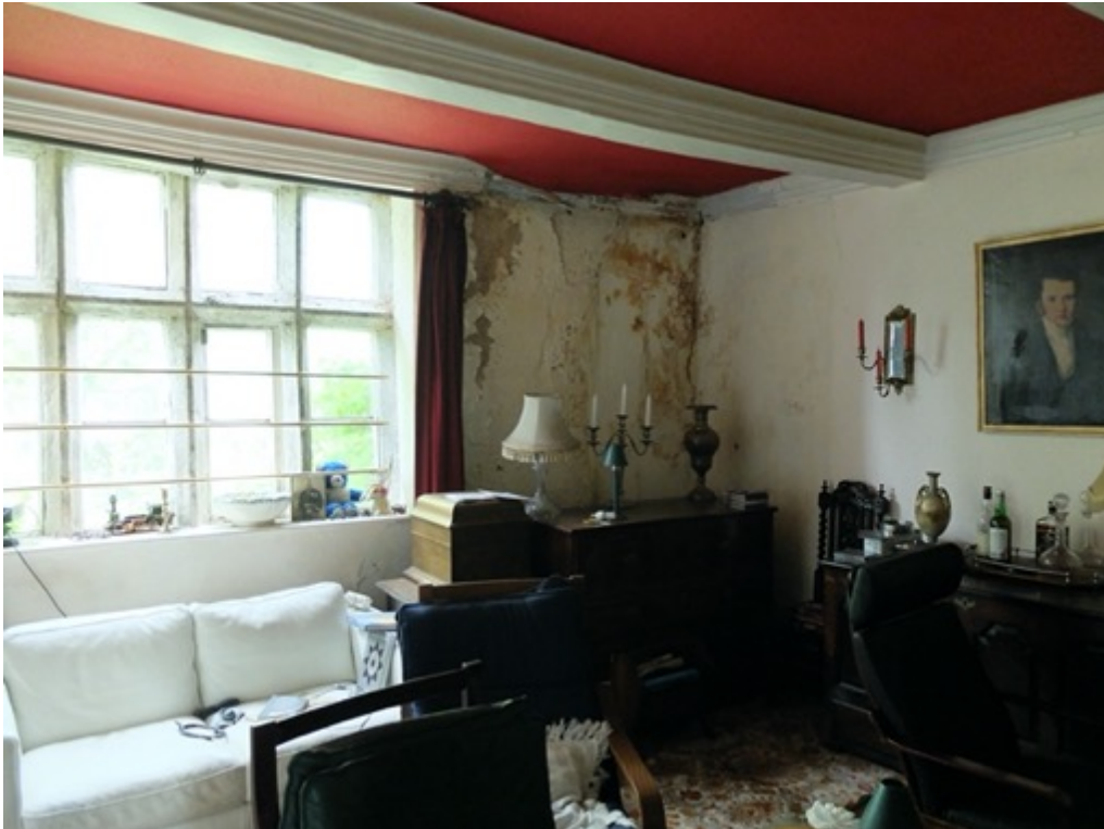
Photo, lounge with leaks to front corner
