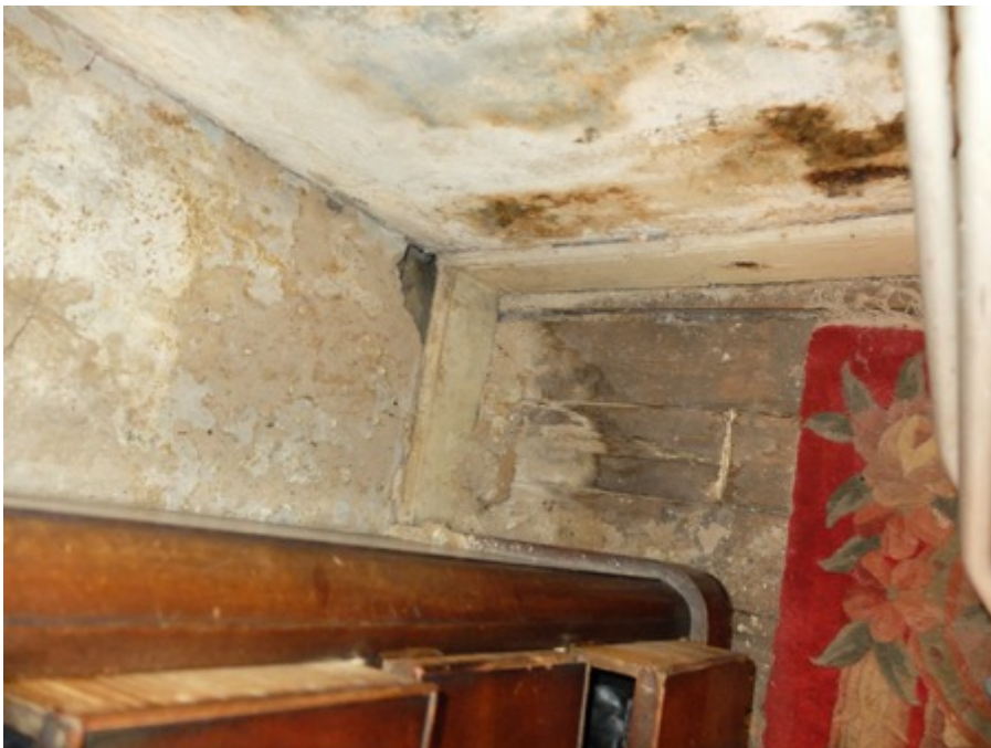
Photo, dampness to floors
