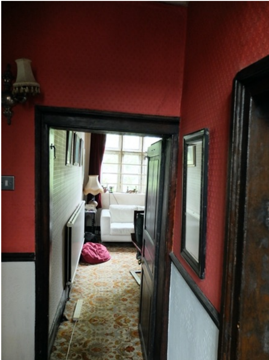
Photo, door casing head out of plumb
