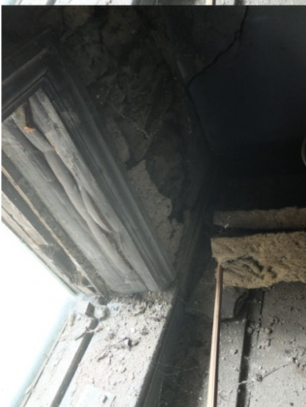
Photo, dry rot in window
