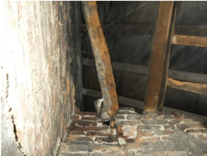
Photo, old oak ridge requires securing
