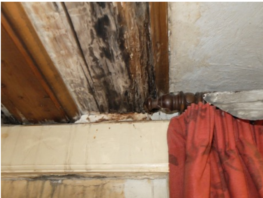
Photo, decay to beams supporting external wall
