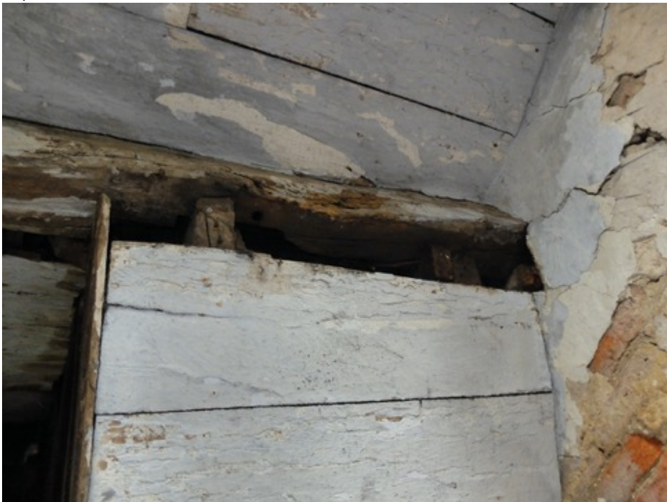
Photo, decay to stair timbers
