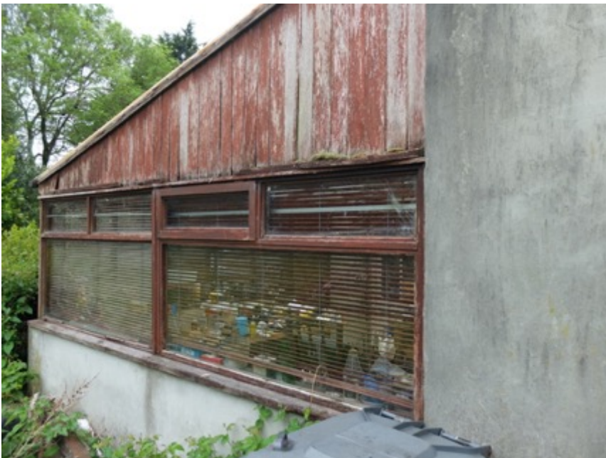
Photo, timber decay to window and matchboard
