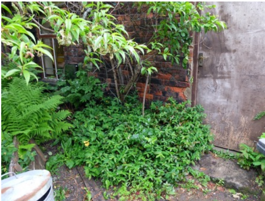
Photo, frost damaged brickwork
