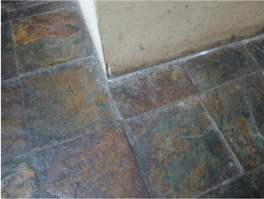
Photo, plaster down to ground level
