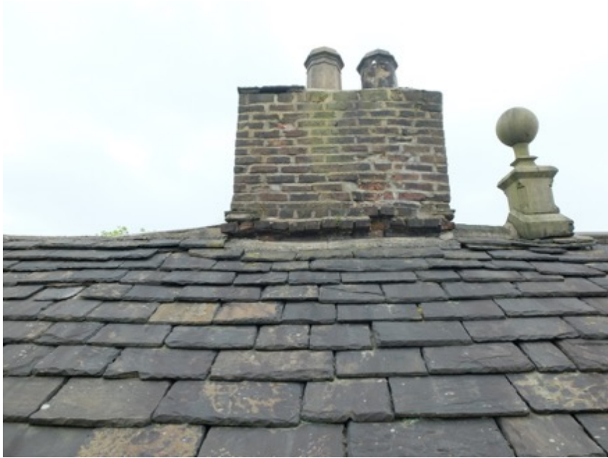
Photo, sulphate attack left chimney
