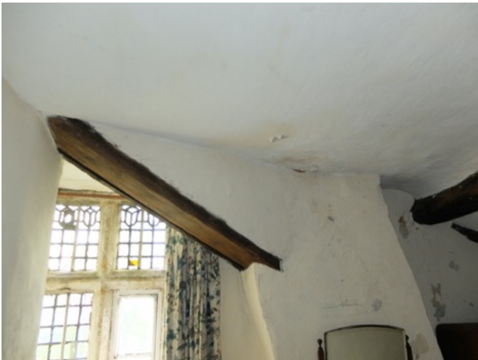
Photo, beam supporting flue and leaks around chimney
