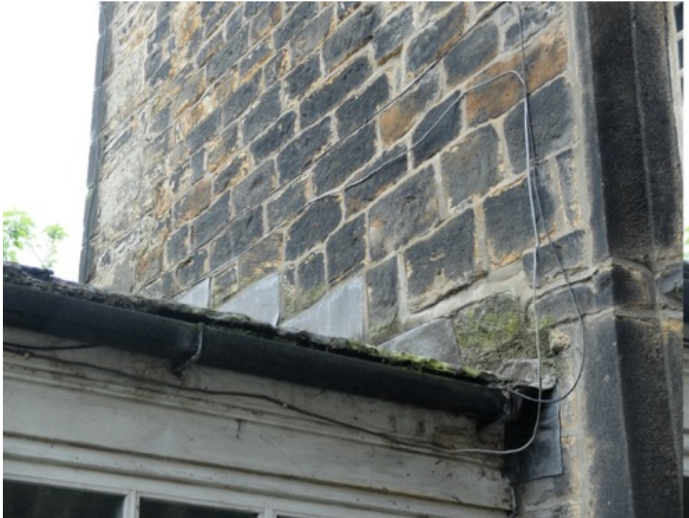
Photo, stepped cracking over roof
