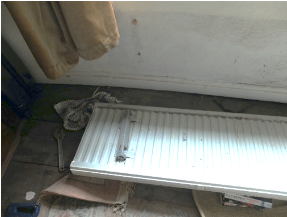
Photo, radiator fallen off wall, gap between floor and skirting
