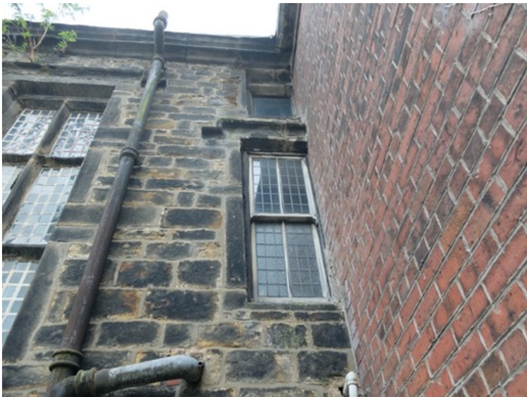
Photo, overflowing of gutters
