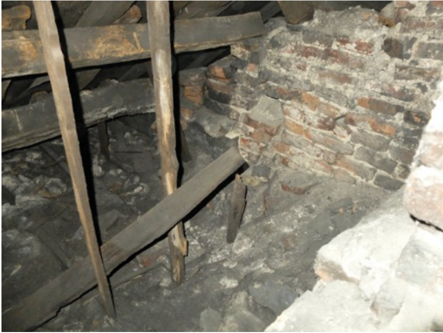
Photo, debris on ceiling and poorly packed purlins on spine wall.
