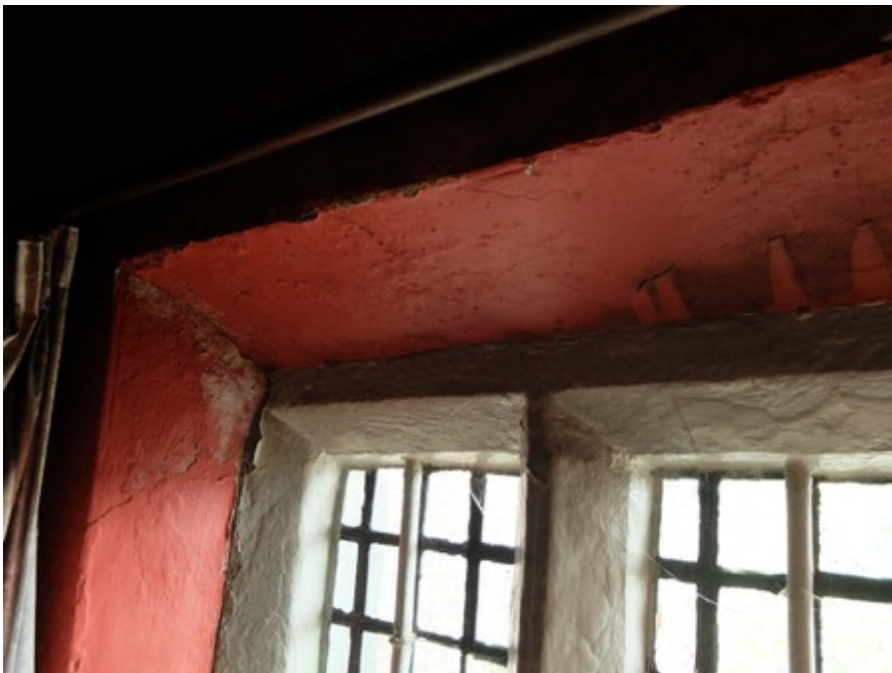
Photo, ingress around top of window
