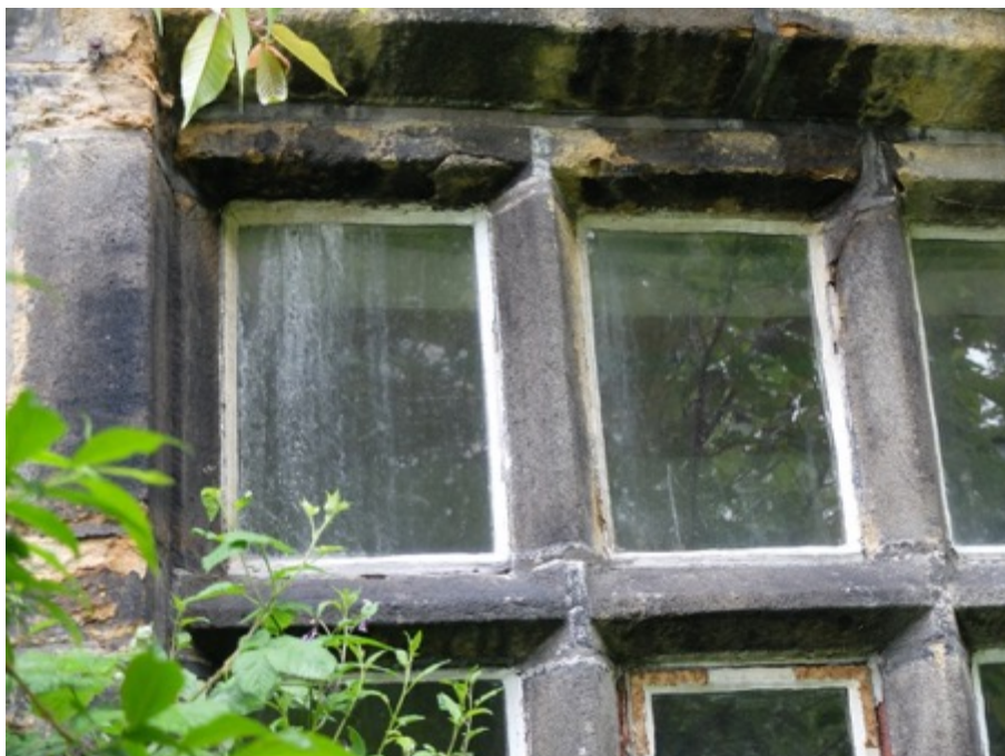
Photo, cracking of stone mullions
