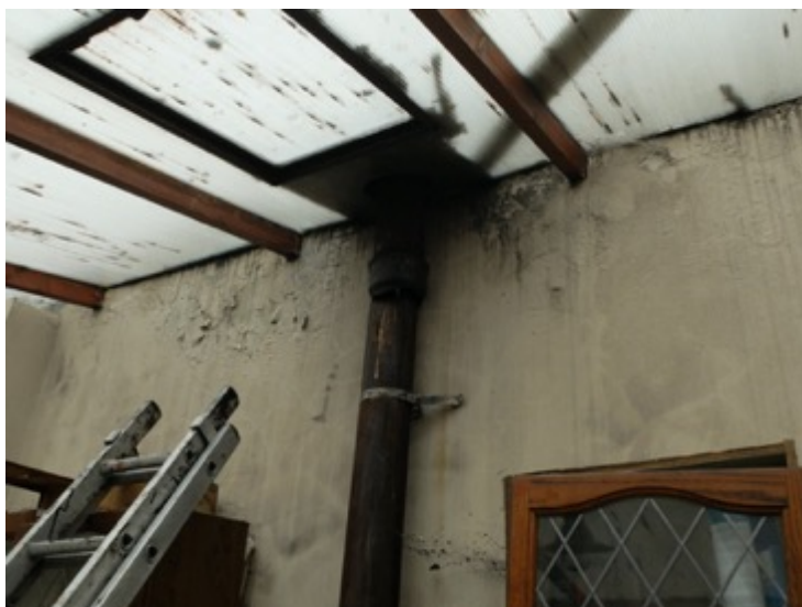
Photo, leaks from ceiling
