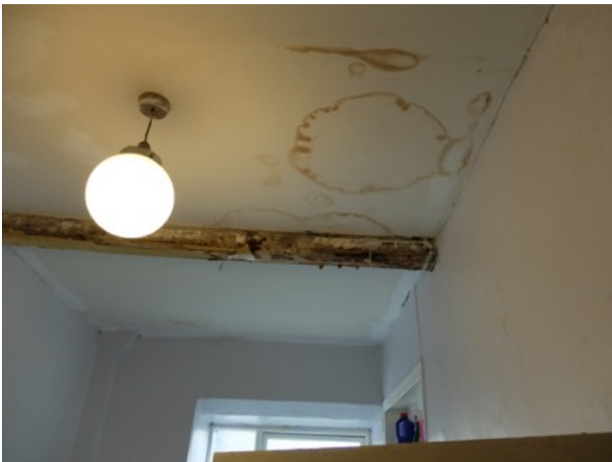
Photo, leaks to ceilings
