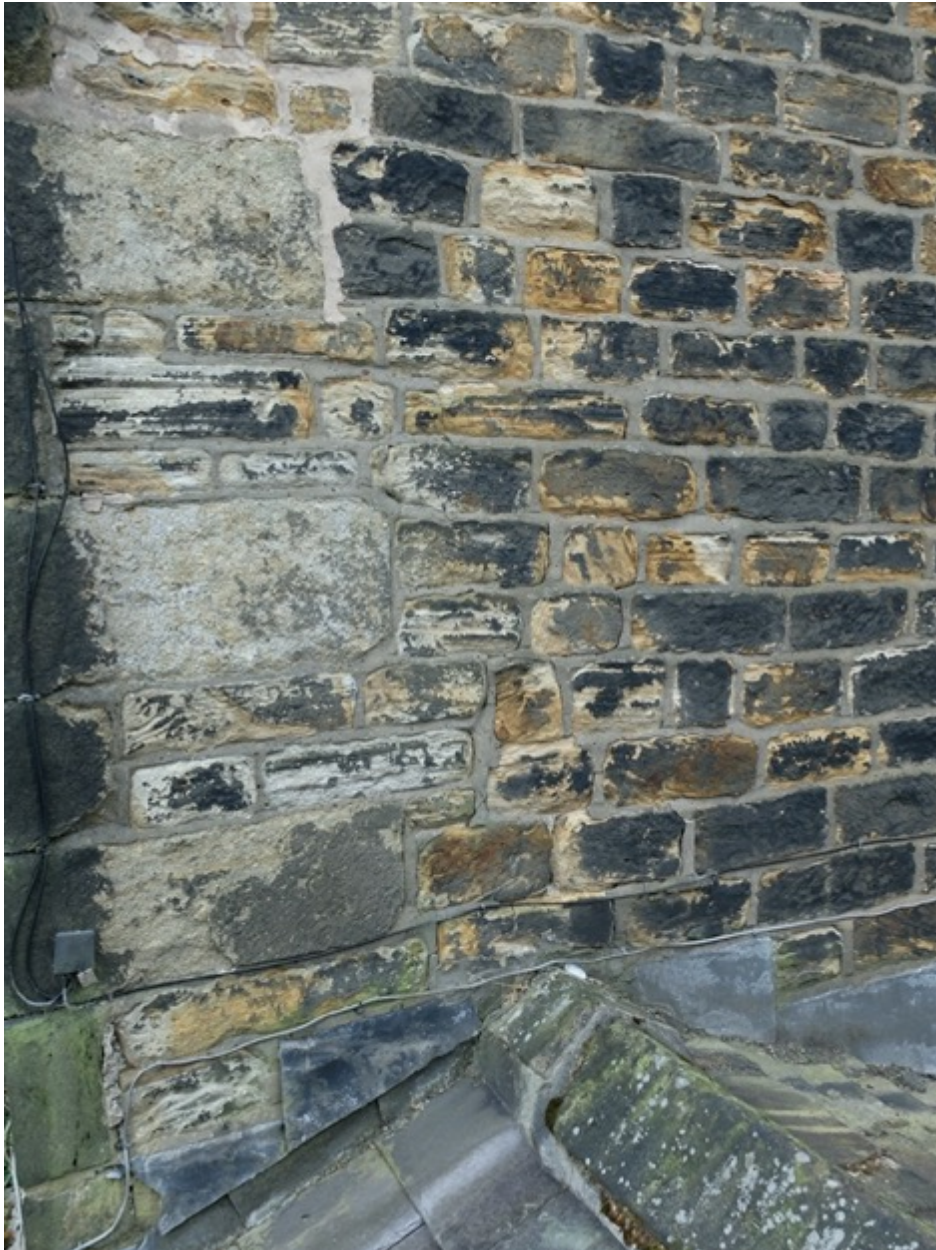
Photo, stepped cracking over dining room
