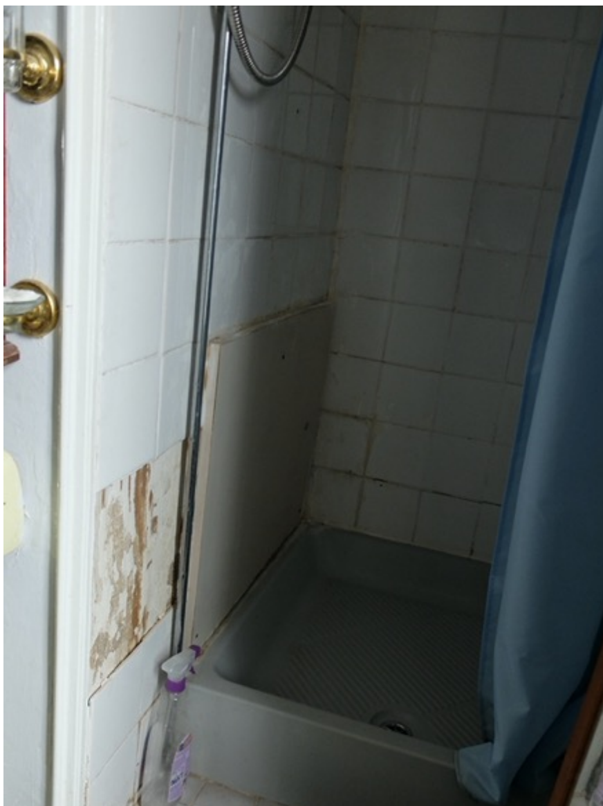
Photo, missing tiles to shower
