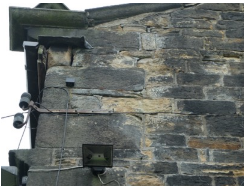
Photo, cracking and frost damage to front kneeler
