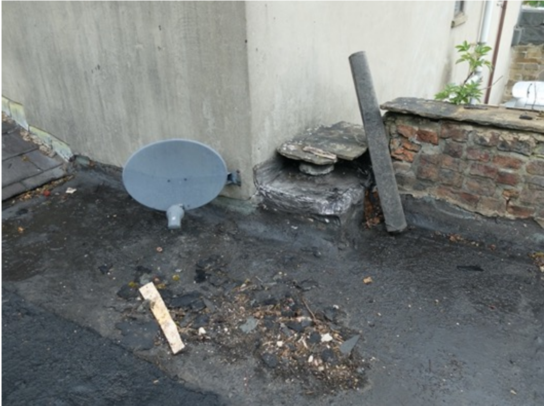
Photo, weathering around cooker extract to roof
