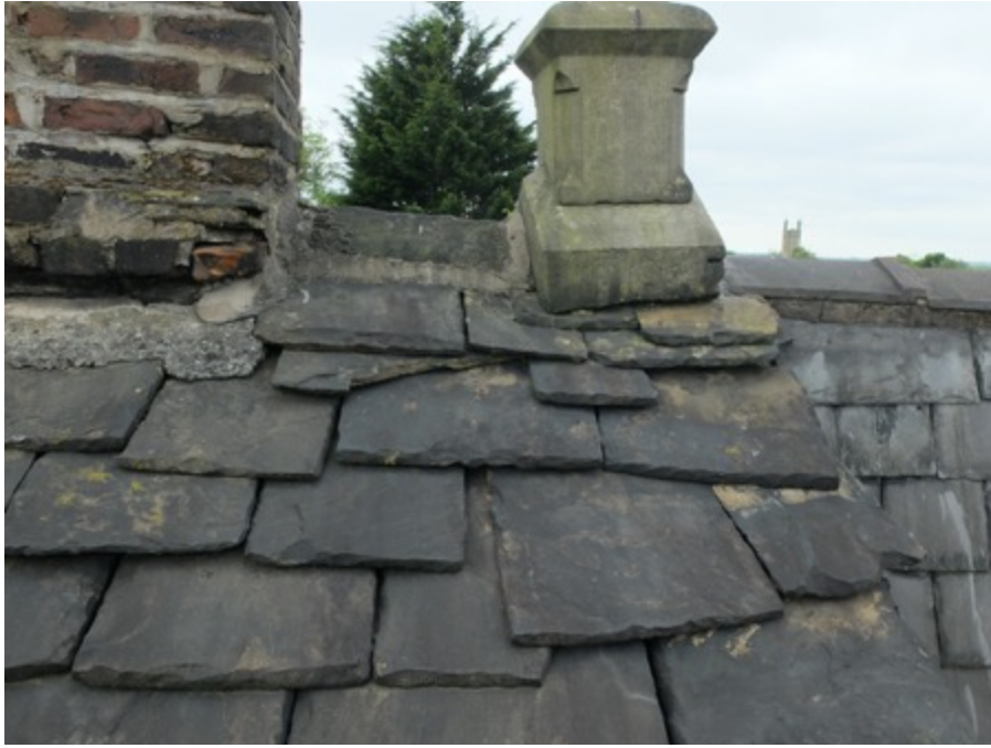
Photo, slipped tiles to rear
