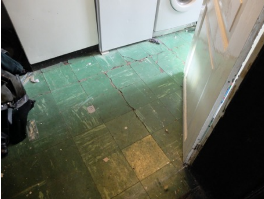
Photo, cracking to floors
