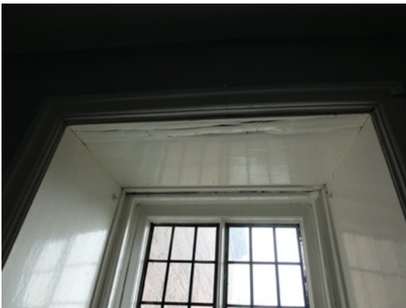
Photo, dry rot to window linings
