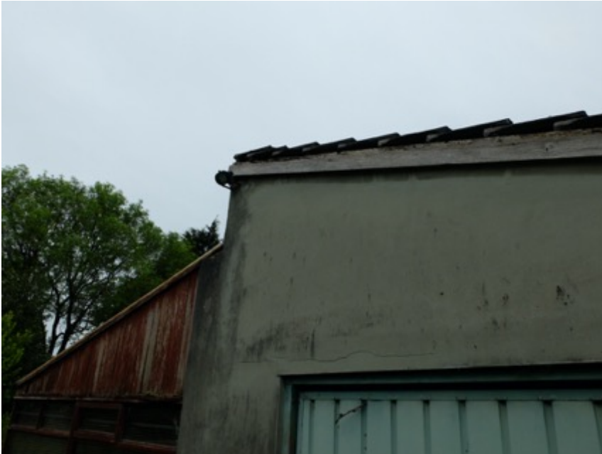
Photo, cracking over garage
