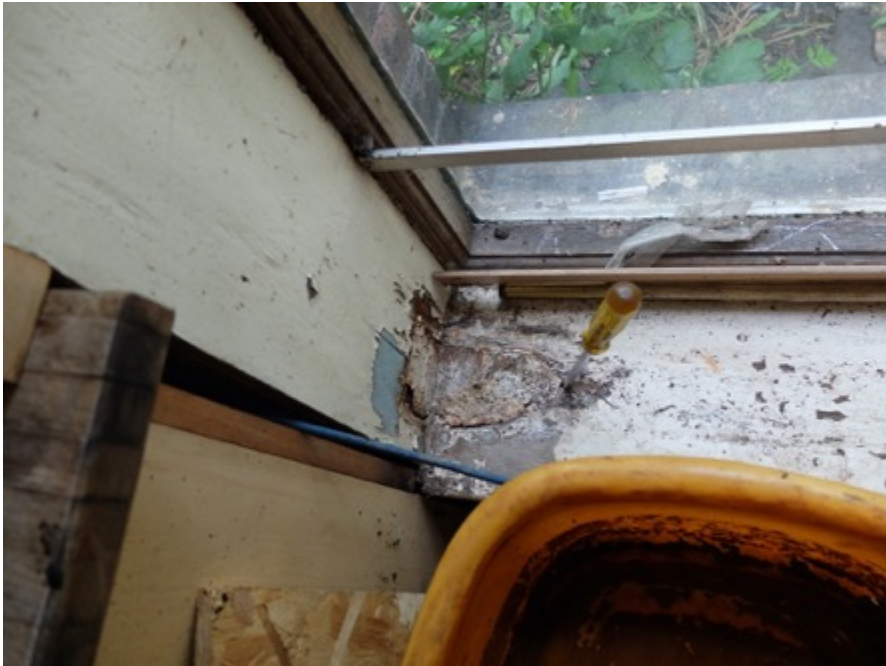
Photo, decay to window board
