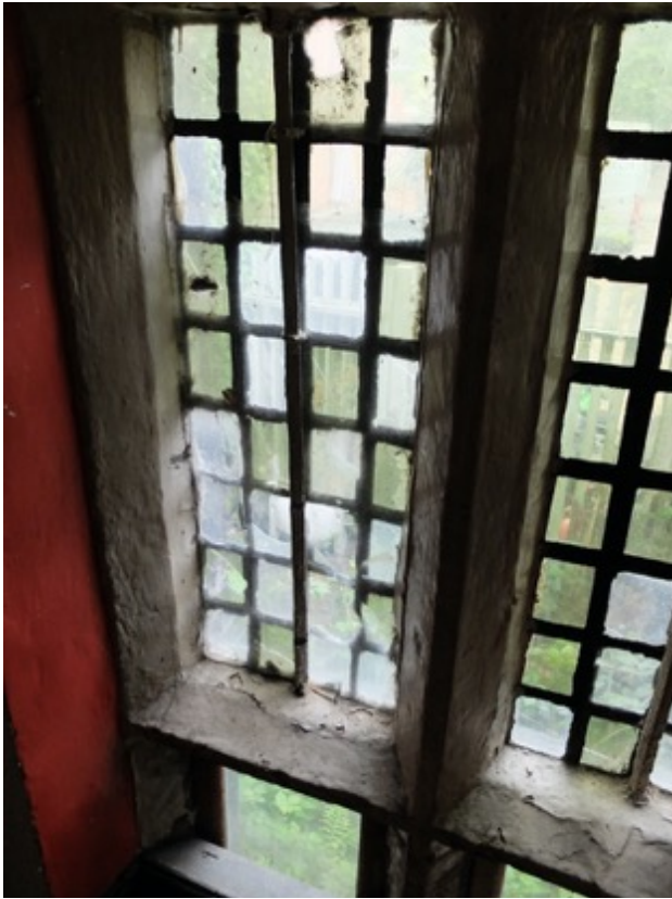
Photo, mullioned window poor condition
