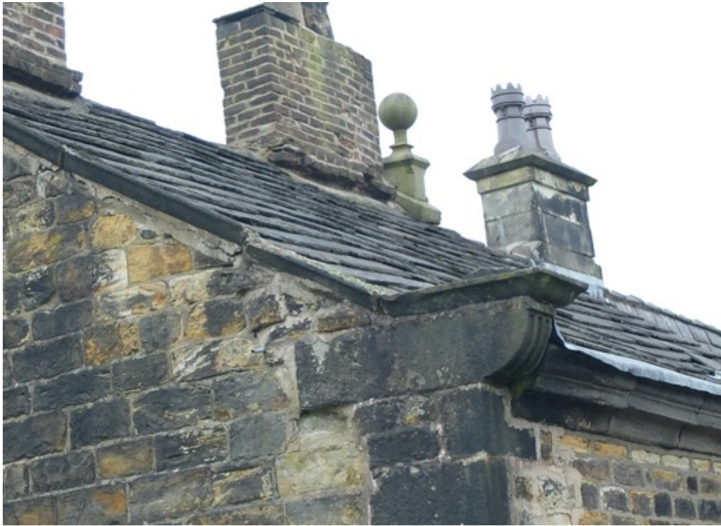
Photo, cracking around rear kneeler
