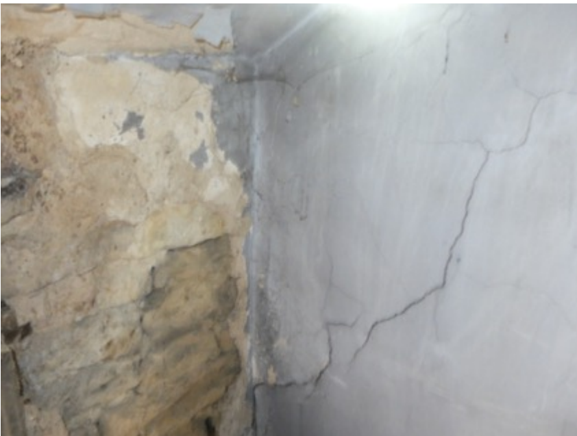
Photo, cracking where spine wall meets with rear external wall
