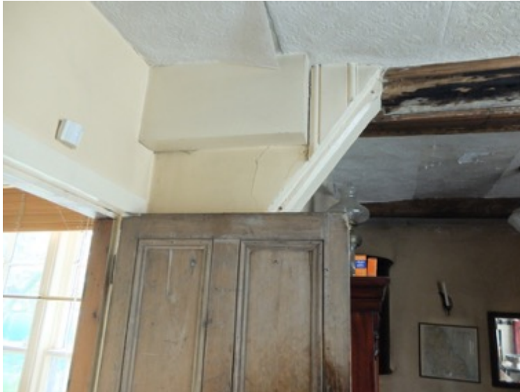
Photo, cracking and brace to other side of beam
