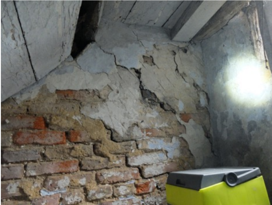
Photo, cracking to brickwork further investigation required
