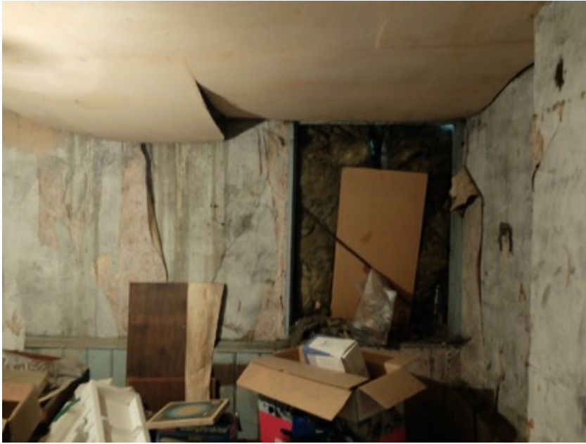
Photo, poor condition of room and blocked window
