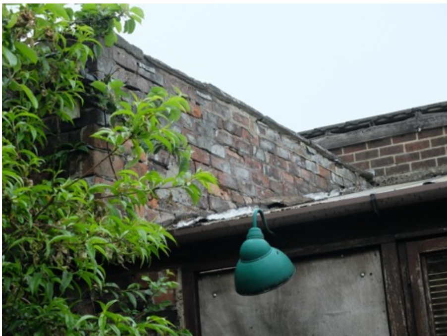
Photo, Frost damage and poor brickwork to high level wall
