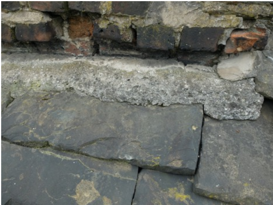
Photo, failed mortar parging
