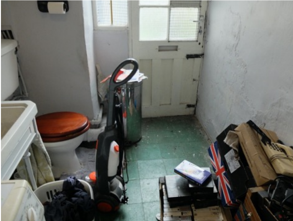
Photo, deterioration of wall plaster right wall
