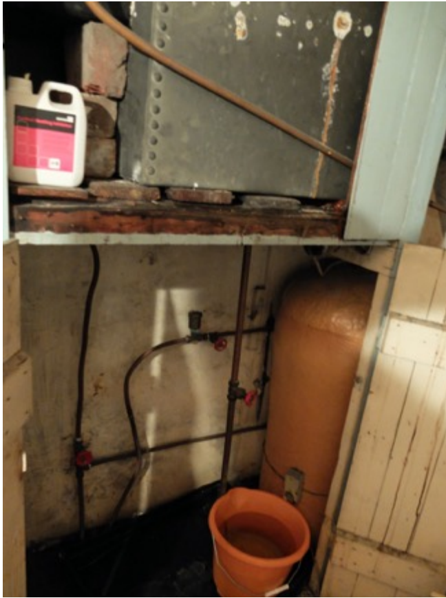
Photo, hot water cylinder
