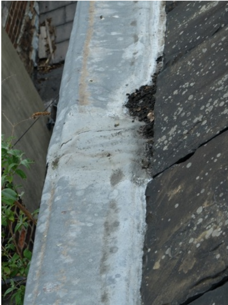
Photo, ingress at joint in rear gutter
