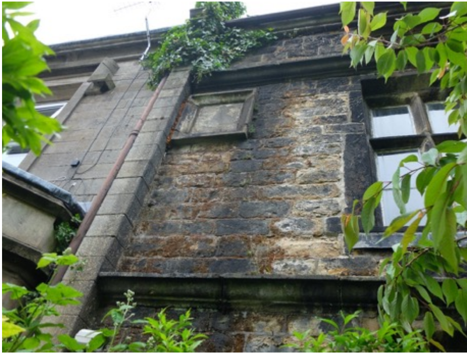
Photo, water percolating down from front gutter
