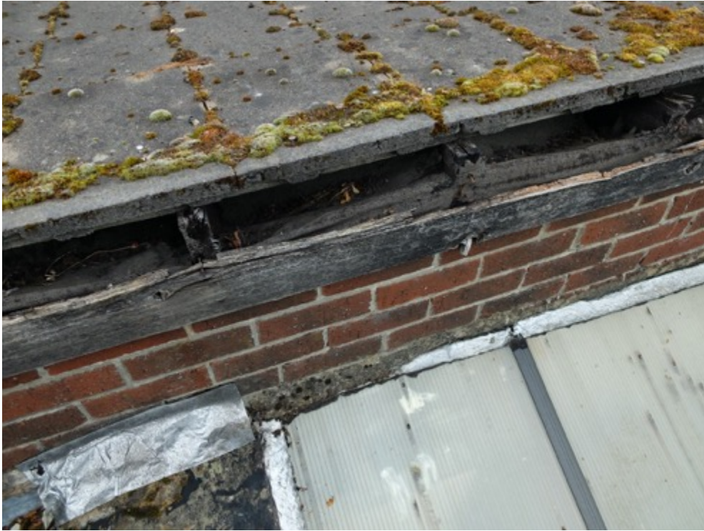
Photo, decay to eaves timbers
