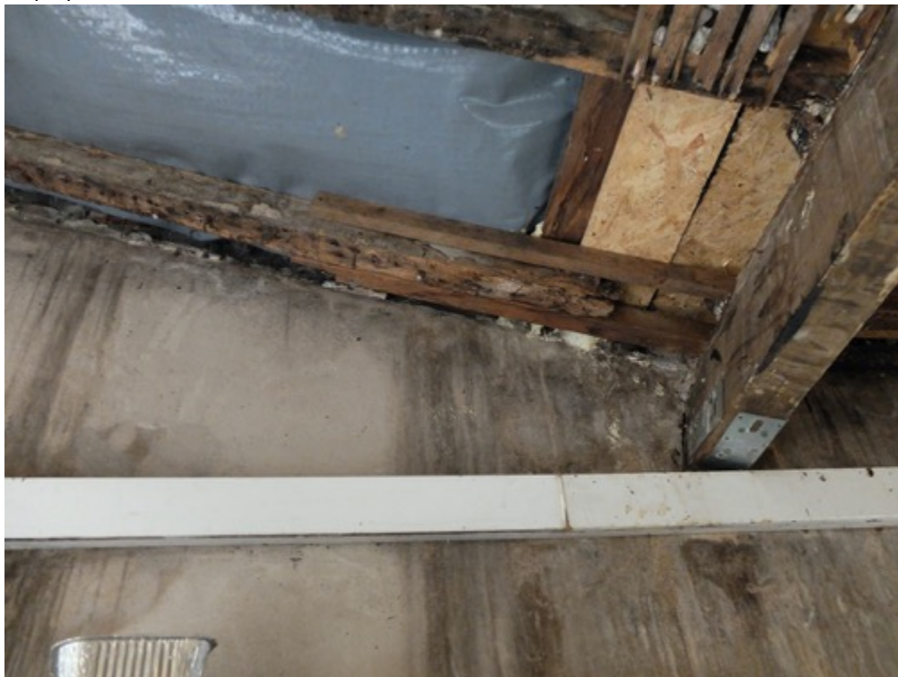
Photo, collapsed ceiling in kitchen under east section
