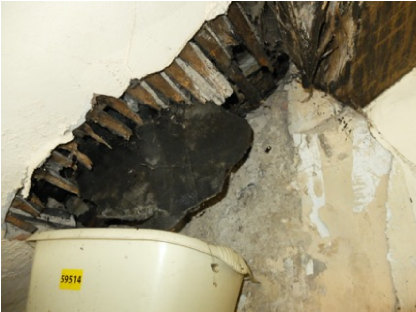
Photo, leaks to ceiling
