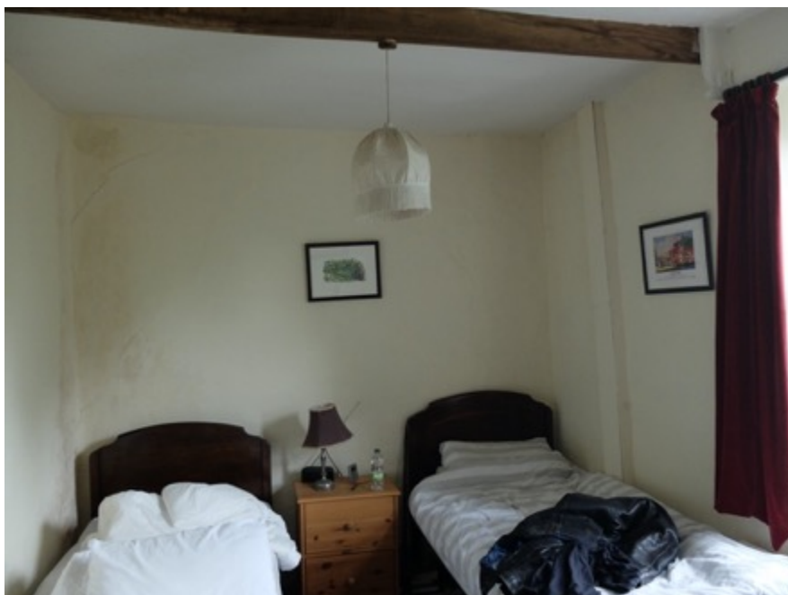
Photo, cracking to rear elevation wall
