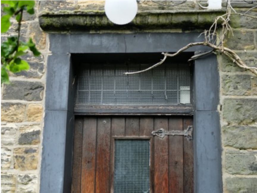
Photo, stuck on lead tape and crack to lintel
