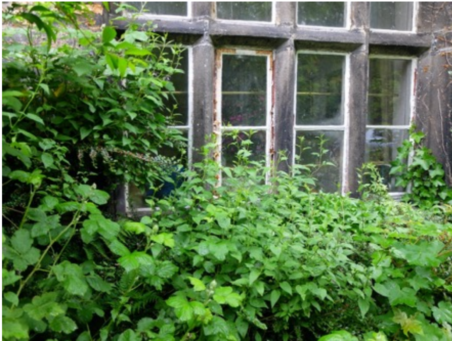
Photo, overgrown at base of walls
