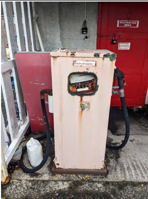
Figure 3 – View north showing a suspected disused diesel pump, with a likely underground storage tank in the north eastern site section
