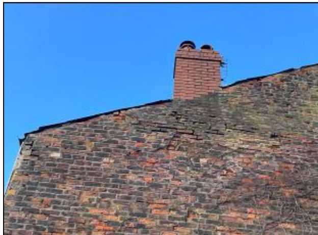
Plate 3 Gaps around verges at southeast gable
