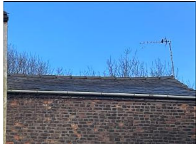
Plate 4 Gaps exist under ridge tiles and fascia board
