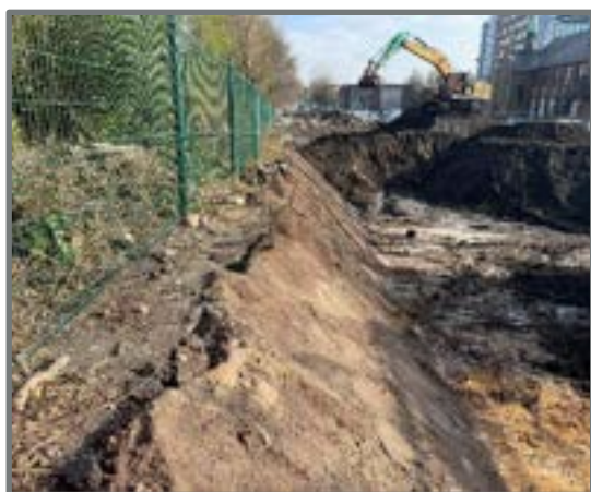
Battered sides of excavation
