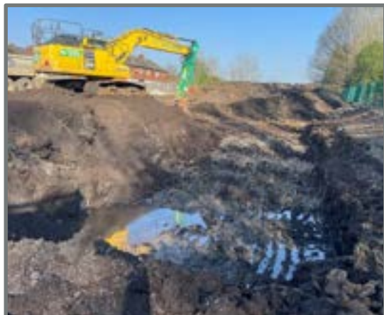
Soft spot in base of excavation
