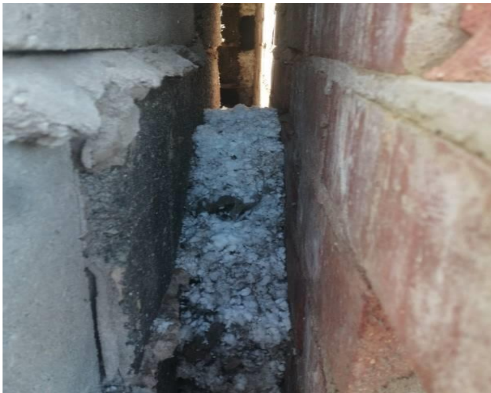
Plate 4- Droppings within the exposed cavity wall at 119 Cornwall Drive
