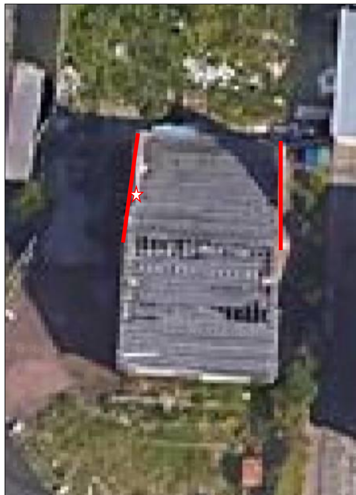
Figure 4: Exposed cavity walls and destroyed roost location denoted with ☆
