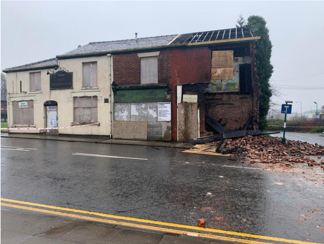
P1 The collapsed structure
