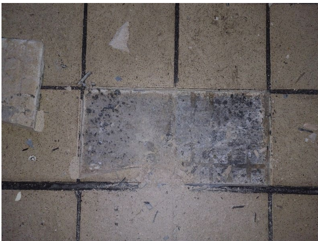
Sample No: 22/12/B/13/MAC8 G.02 Rear of shop Floor below ceramic tiles Residual bitumen adhesive containing: Chrysotile
