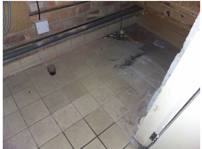
Sample No: Refer to Sample 22/12/B/13/MAC8 G.03 Understairs cupboard Floor below ceramic tiles Residual bitumen adhesive containing: Chrysotile
