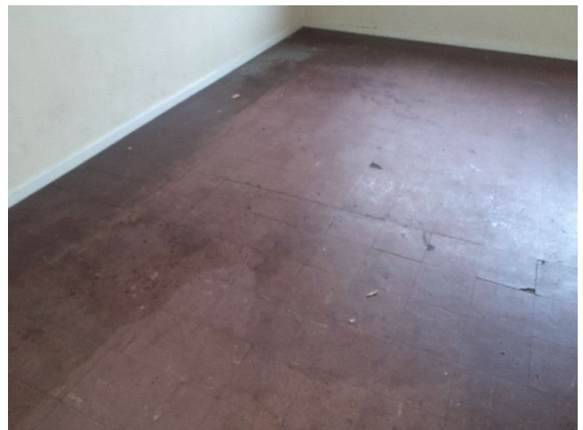
Sample No: 22/12/B/13/MAC11 1.01 Staff room Floor Vinyl floor tiles and bitumen adhesive containing: Chrysotile (In both tile and bitumen)
