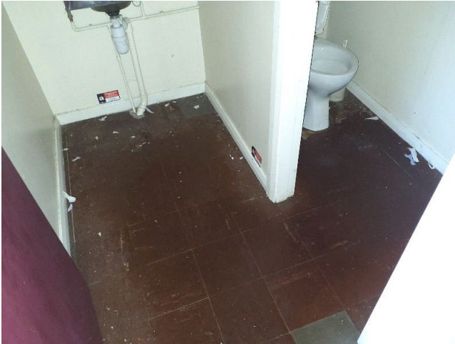
Sample No: Refer to Sample 22/12/B/13/MAC11 1.02 Toilets Floor Vinyl floor tiles and bitumen adhesive containing: Chrysotile (In both tile and bitumen)
