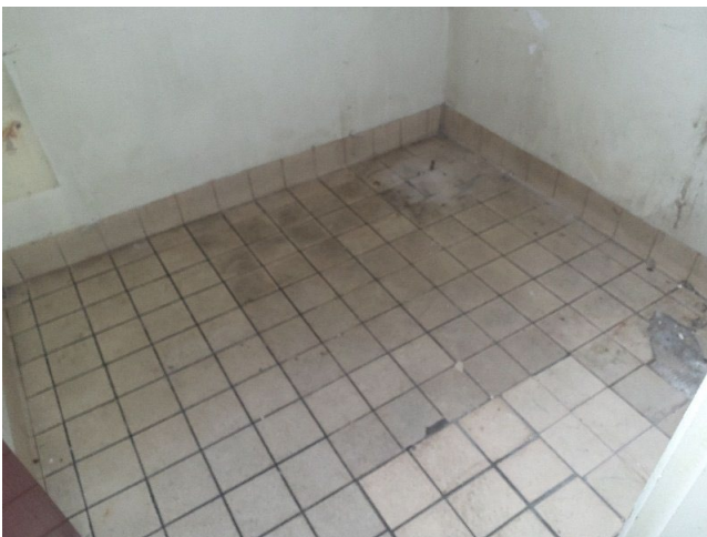
Sample No: Refer to Sample 22/12/B/13/MAC8 G.04 Cloakroom Floor below ceramic tiles Residual bitumen adhesive containing: Chrysotile
