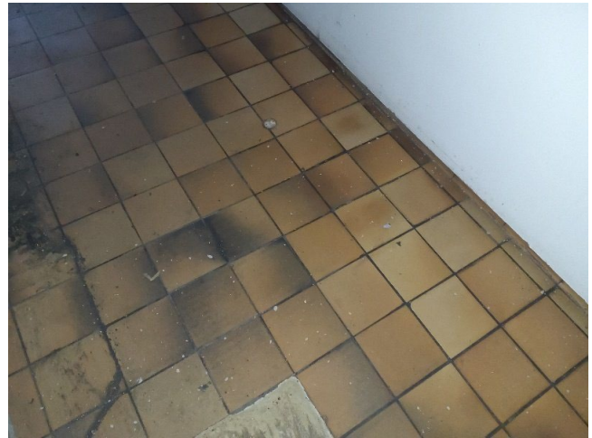
Sample No: Refer to Sample 22/12/B/13/MAC8 G.01 Front of shop Floor below ceramic tiles Residual bitumen adhesive containing: Chrysotile
