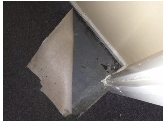
Sample No: 22/12/B/12/SAW2 1.01 Landing Floor Vinyl floor tiles with bitumen adhesive containing: Chrysotile (In both tile and bitumen)
