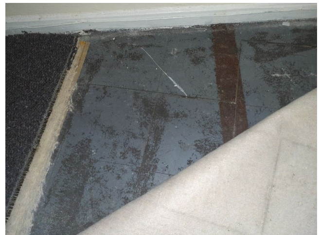
Sample No: Refer to Sample 22/12/B/12/SAW2 1.04 Office Floor Vinyl floor tiles with bitumen adhesive containing: Chrysotile (In both tile and bitumen)
