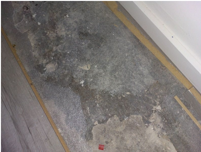
Sample No: Refer to Sample 22/12/B/12/SAW1 G.02 Rear Shop area Floor beneath screed Bitumen residuals containing: Chrysotile
