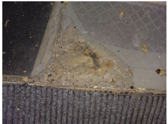
Sample No: 22/12/B/12/SAW1 G.01 Shop area Floor beneath screed Bitumen residuals containing: Chrysotile
