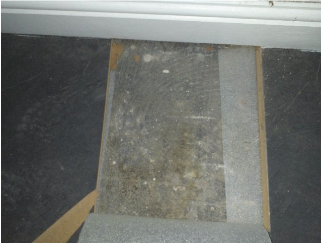
Sample No: Refer to Sample 22/12/B/12/SAW7 1.05 Sunbed room Floor Bitumen residuals containing: Chrysotile
