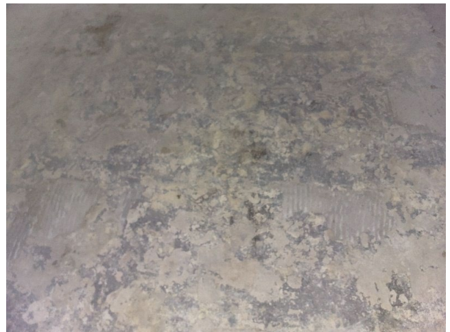
Sample No: 22/12/B/12/SAW6 G.01 Shop area Floor beneath screed Bitumen residuals containing: Chrysotile
