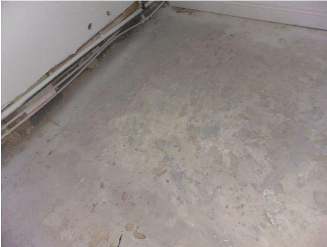
Sample No: Refer to Sample 22/12/B/12/SAW6 G.02 Office Floor beneath screed Bitumen residuals containing: Chrysotile
