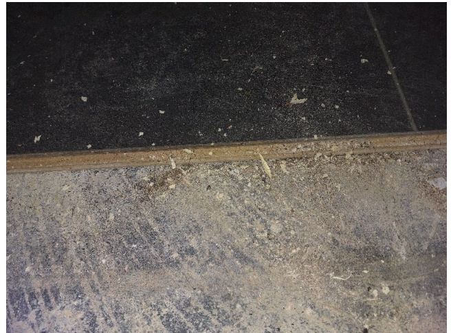
Sample No: Refer to Sample 22/12/B/12/SAW7 1.02 Tanning room Floor Bitumen residuals containing: Chrysotile
