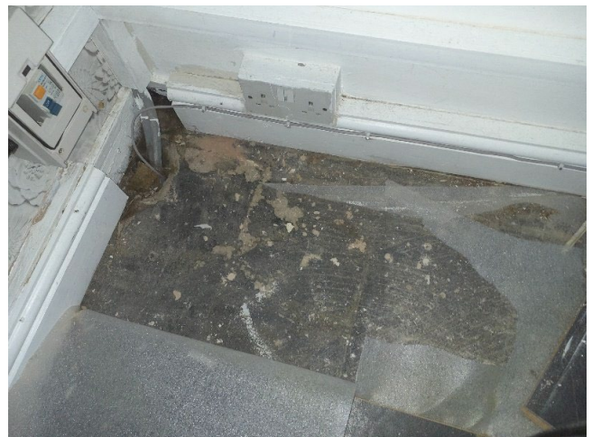
Sample No: Refer to Sample 22/12/B/12/SAW7 1.04 Sunbed room Floor Bitumen residuals containing: Chrysotile
