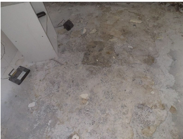
Sample No: Refer to Sample 22/12/B/12/SAW6 G.05 Office Floor beneath screed Bitumen residuals containing: Chrysotile
