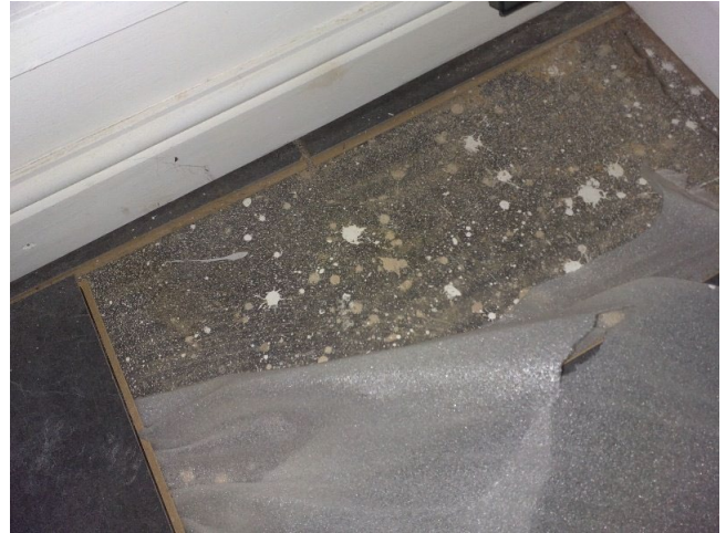
Sample No: Refer to Sample 22/12/B/12/SAW7 1.06 Office Floor Bitumen residuals containing: Chrysotile
