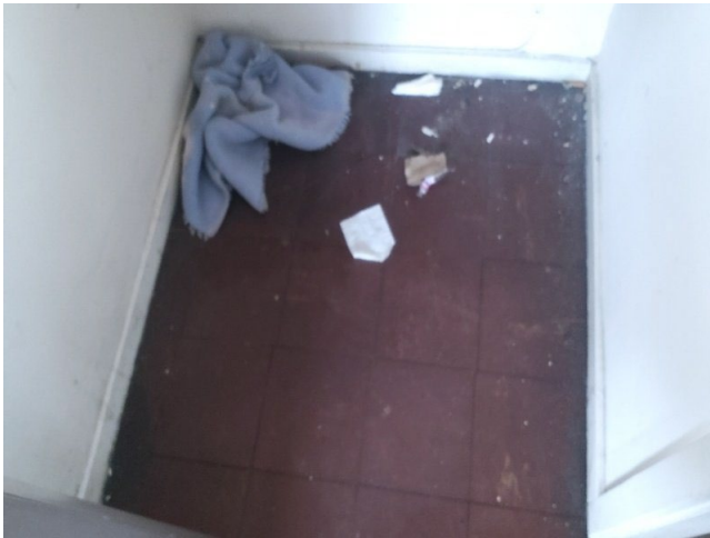
Sample No: Refer to Sample 22/12/B/12/MBK7 2.02 Gents toilet lobby Floor
