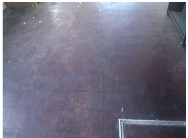
Sample No: 22/12/B/12/MBK4 1.02 Open plan storage space Floor Vinyl Floor Tiles containing: Chrysotile (In tile only)
