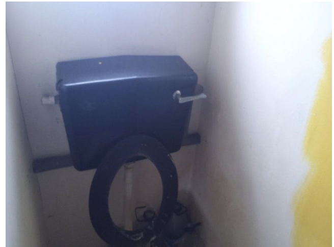
Sample No: 22/12/B/12/MBK8 2.03 Gents toilet Toilet Cistern
