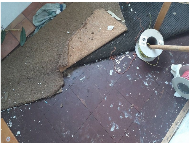
Sample No: Refer to Sample 22/12/B/12/MBK4 1.04 Store Floor Vinyl Floor Tiles containing: Chrysotile (In tile only)
