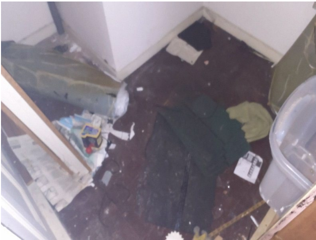
Sample No: Refer to Sample 22/12/B/12/MBK4 1.03 Store Floor Vinyl Floor Tiles containing: Chrysotile (In tile only)
