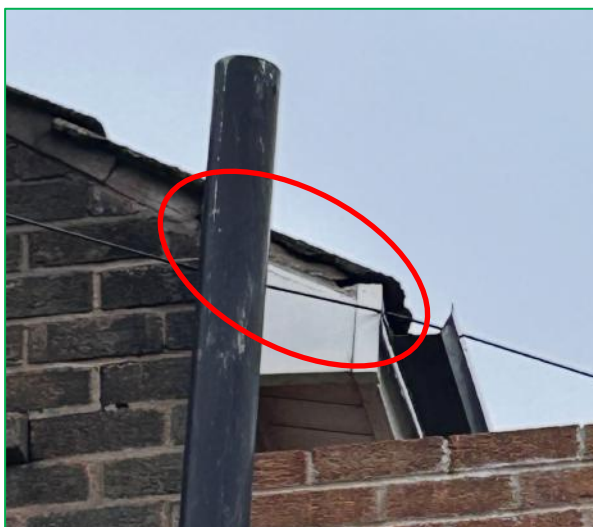
Showing crevices under the tiles on the south elevation of the house
