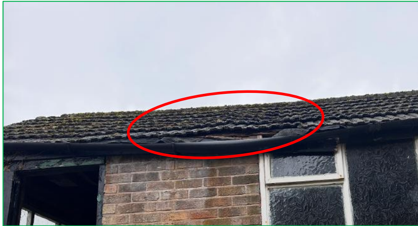
Showing damage to the shed roof providing potential access for bats between the tiles and the lining
