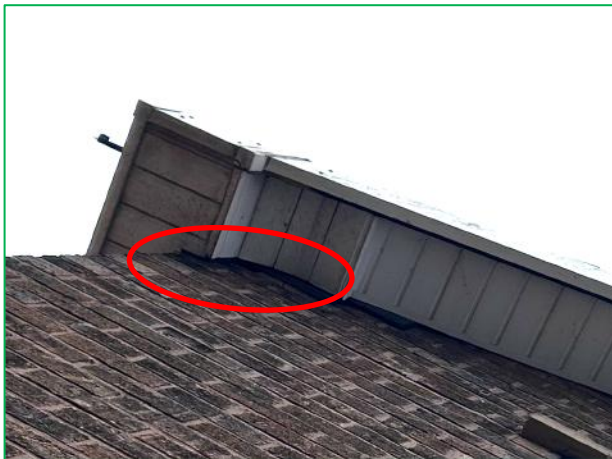
Showing a small gap under the soffit of the house on the north elevation.
