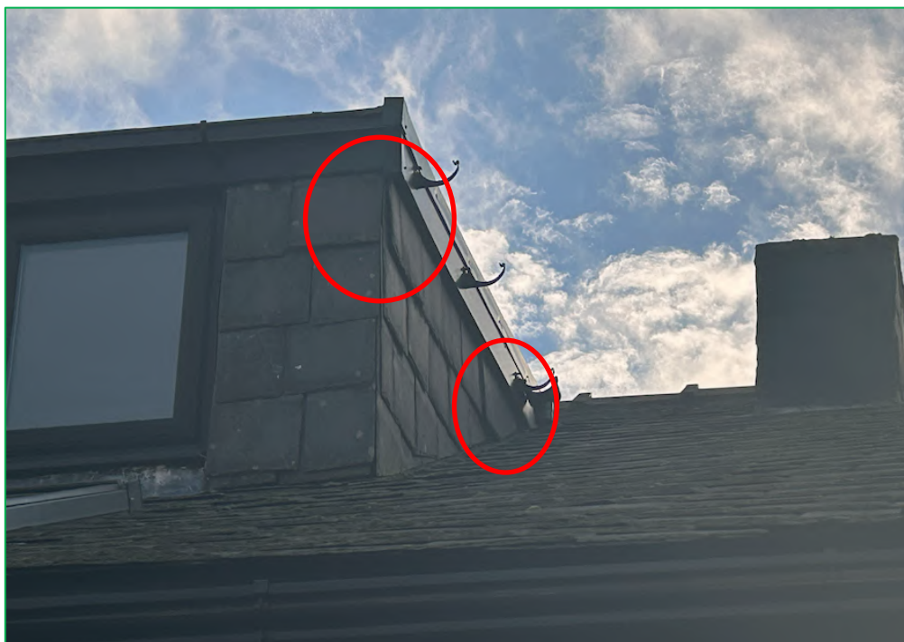
Showing gaps under lifted slates on the rear of the building
