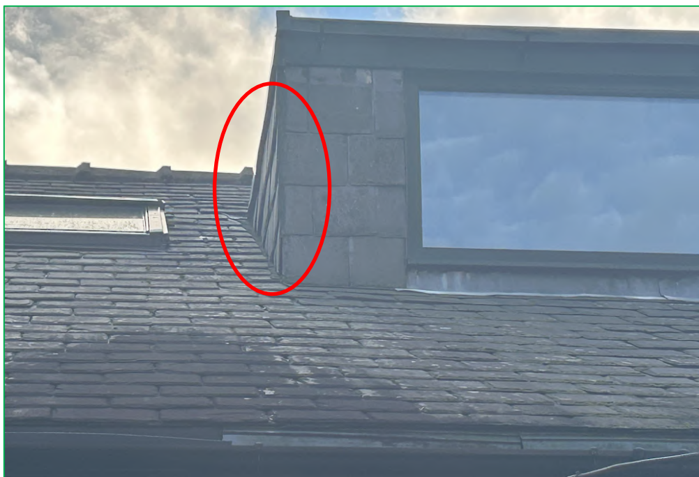
Showing gaps under lifted slates on the rear of the building
