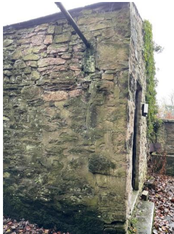
(25) Poor quality rubble walling
