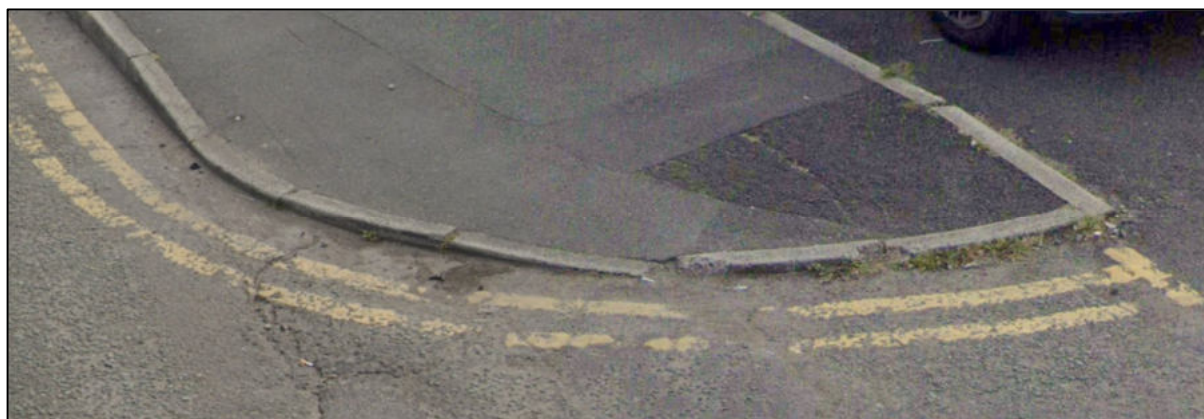
115m – Kerbs in poor condition. Worn double yellow lines.
