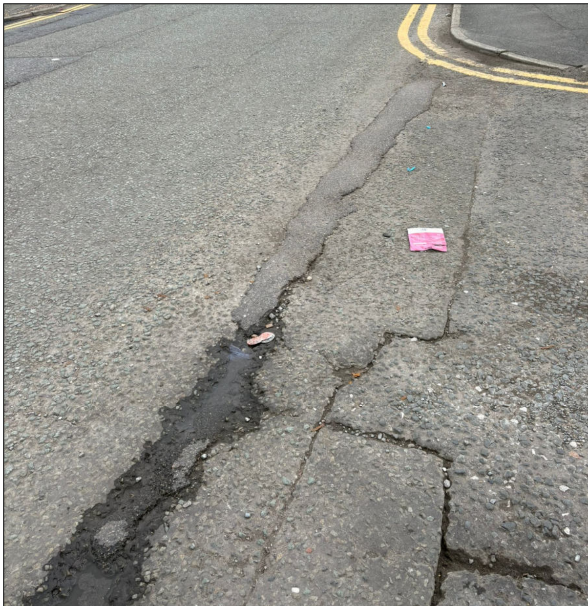
110m – Poor carriageway reinstatement at the access
