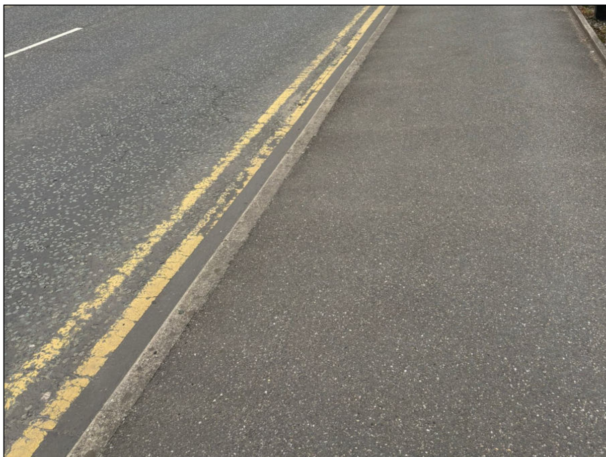
21m – Cracked carriageway and worn double yellow lines
