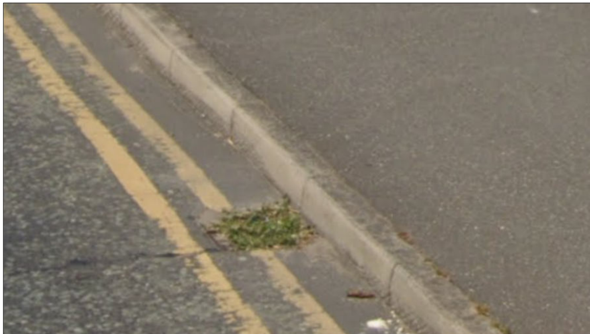
18m – Gulley blocked in carriageway
