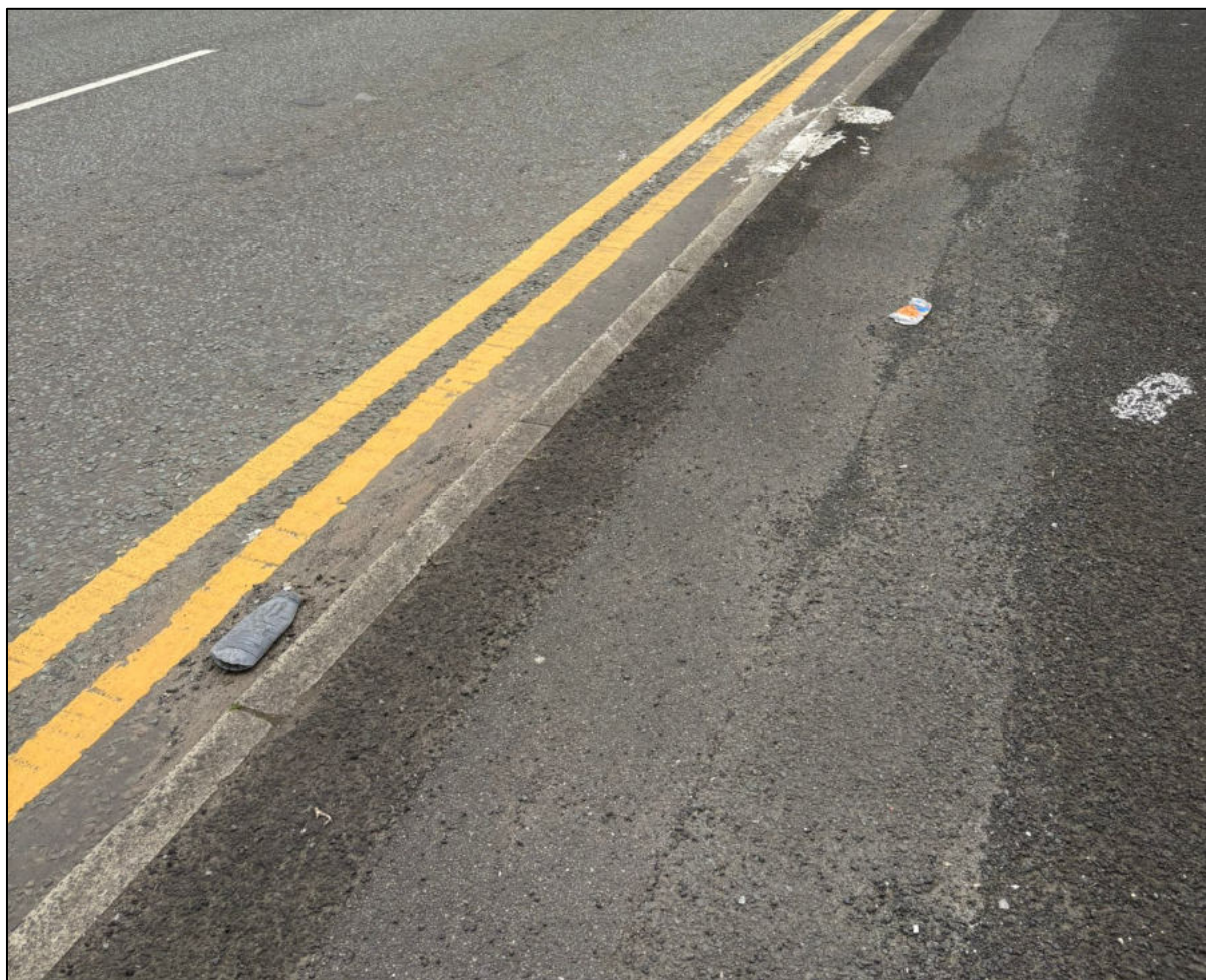
59m – Footway condition worn
