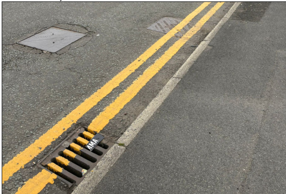
122m – Failed utility cover
