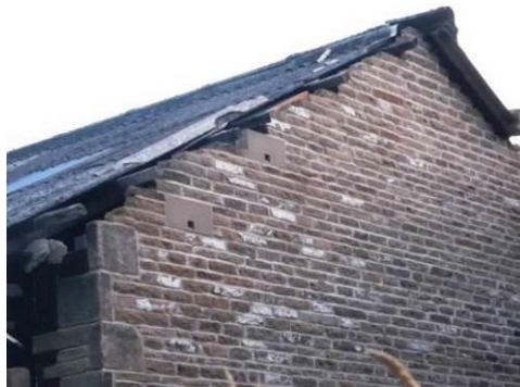
Example of Forticrete boxes in situ
