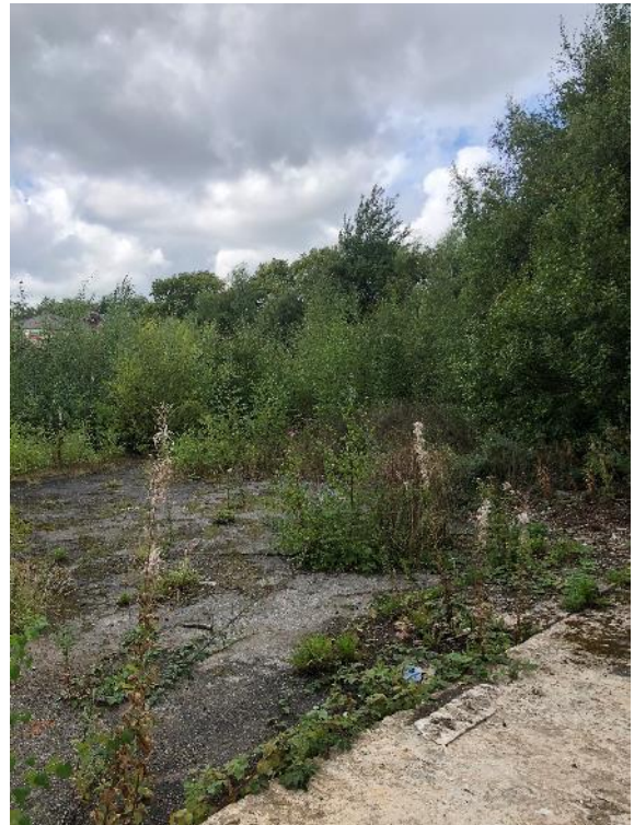
Photograph 3: TN1 scattered scrub growing through cracks in the concrete.
