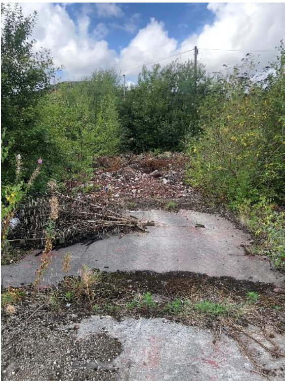
Photograph 2: TN1 area of buddleia and willow scrub forming in cracks in the concrete.
