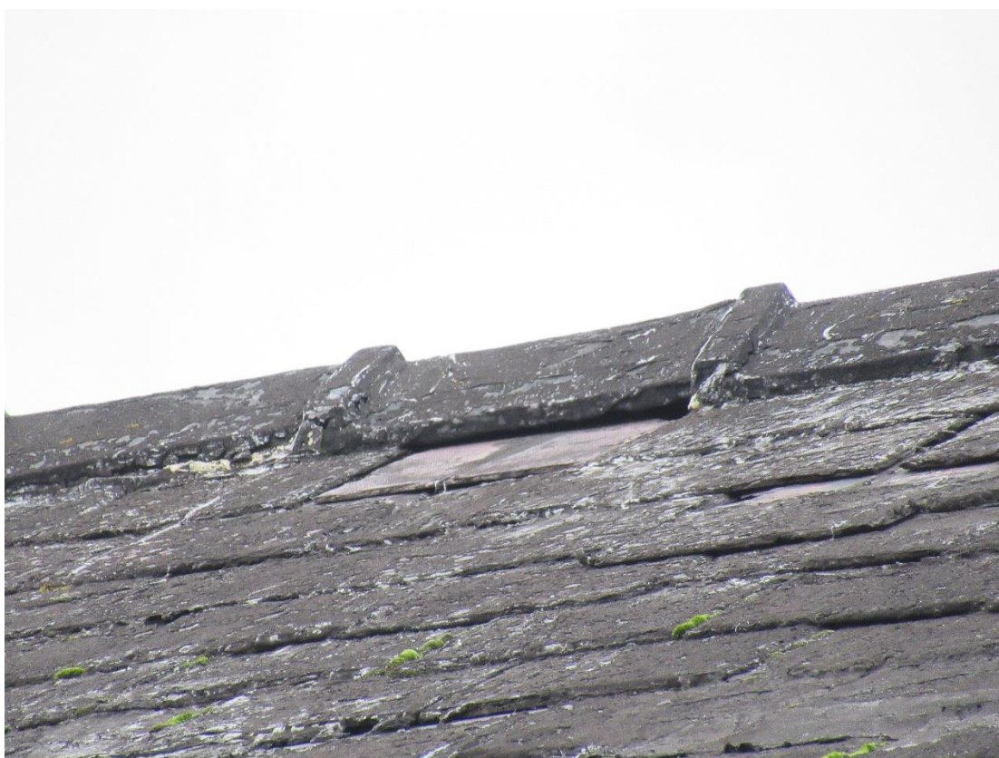
Photograph 10 – Example of gap under a ridge tile on the south-eastern aspect.
