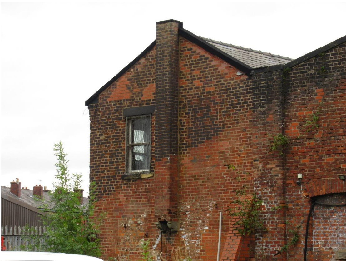
Photograph 14 – Damaged chimney on the north-western aspect.
