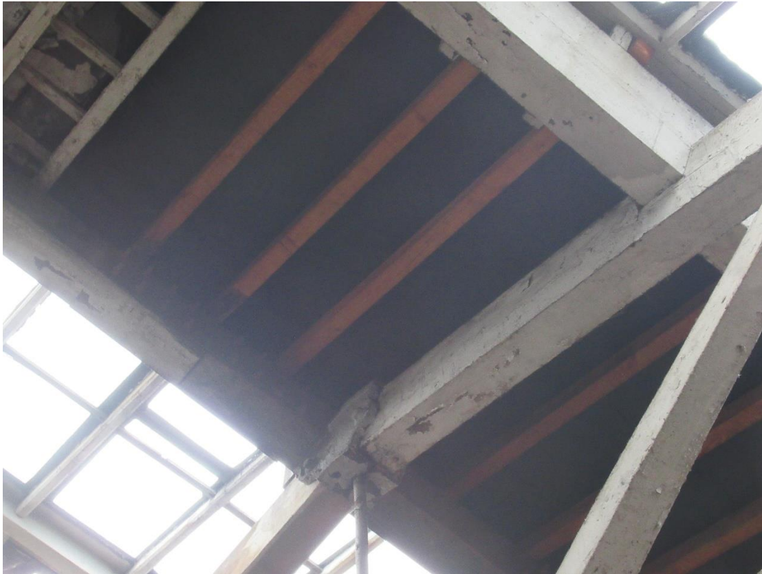
Photograph 17 – Small section of bitumen felt roof lining in the north-western section.
