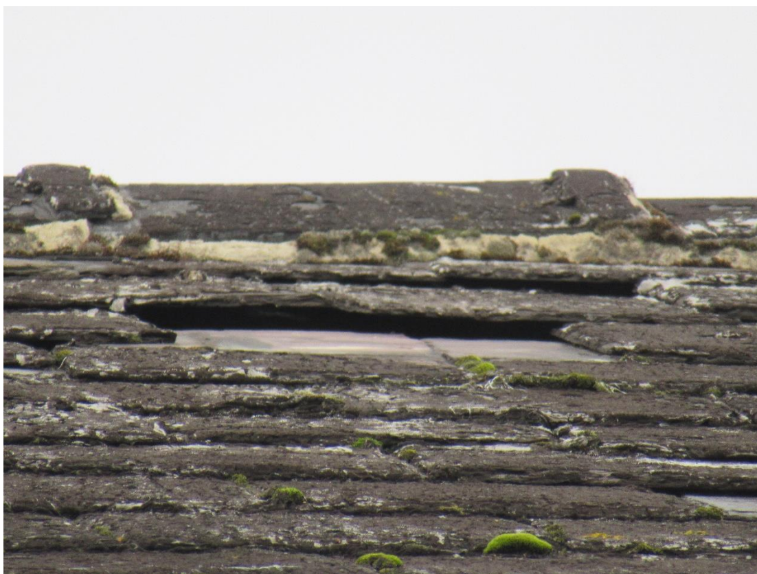
Photograph 9 – Example of gap from missing roof tile on the south-eastern aspect.
