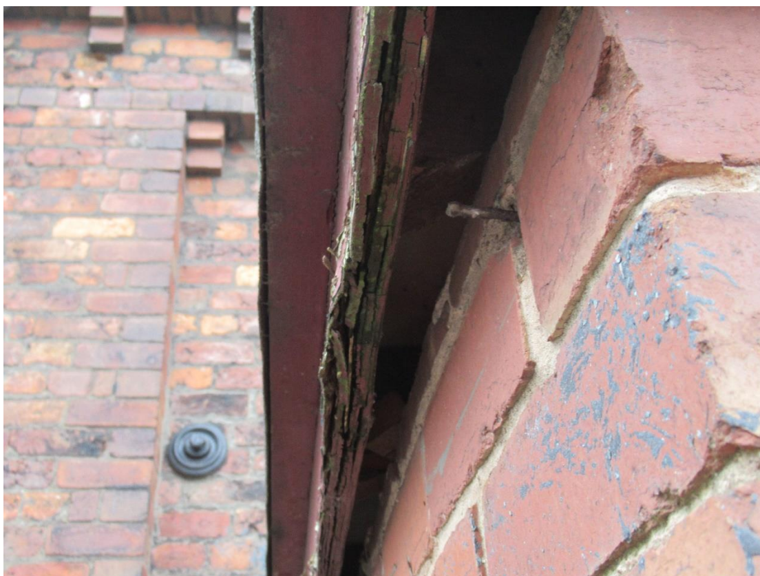
Photograph 11 – Gap behind the wooden bargeboard on the single storey extension.
