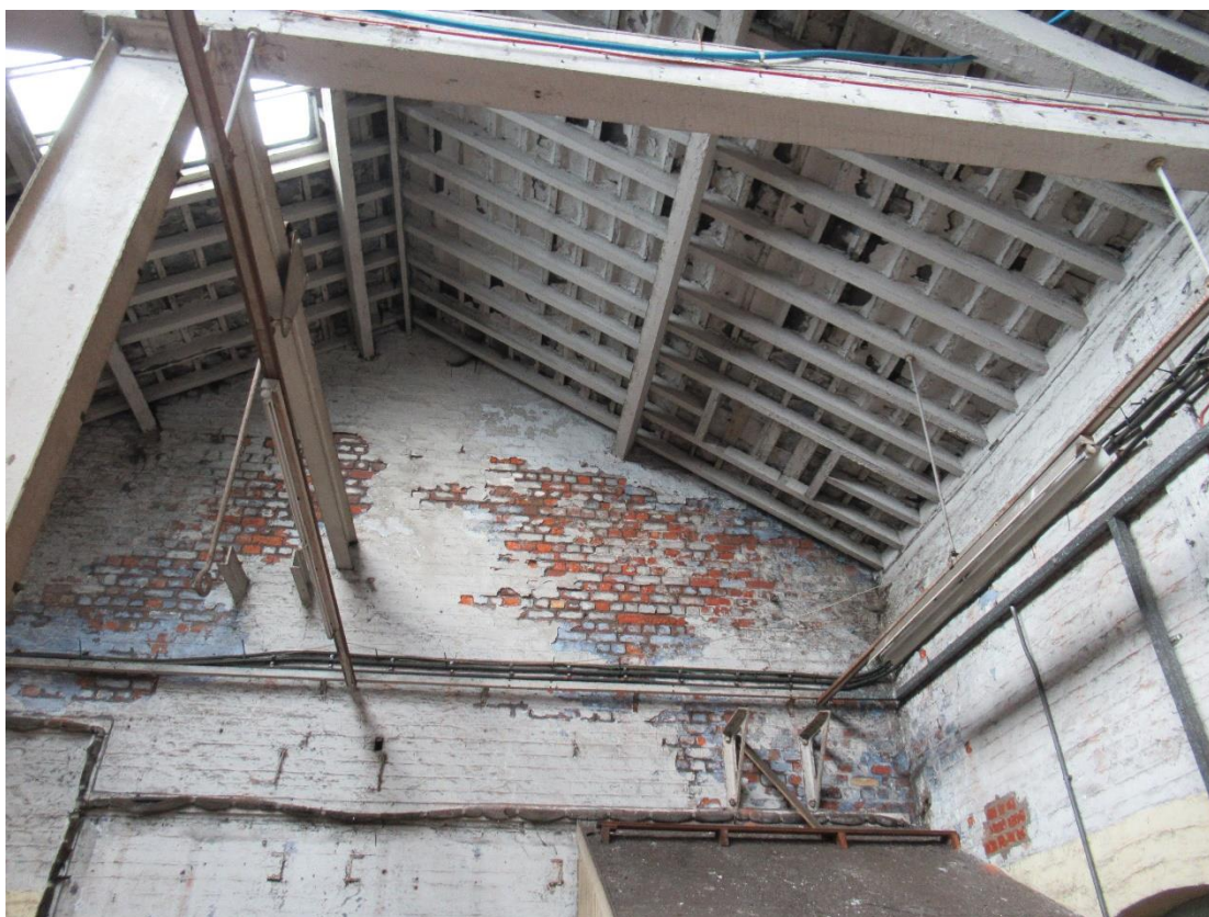
Photograph 15 – Inside of the building, showing no loft void and unlined roof.
