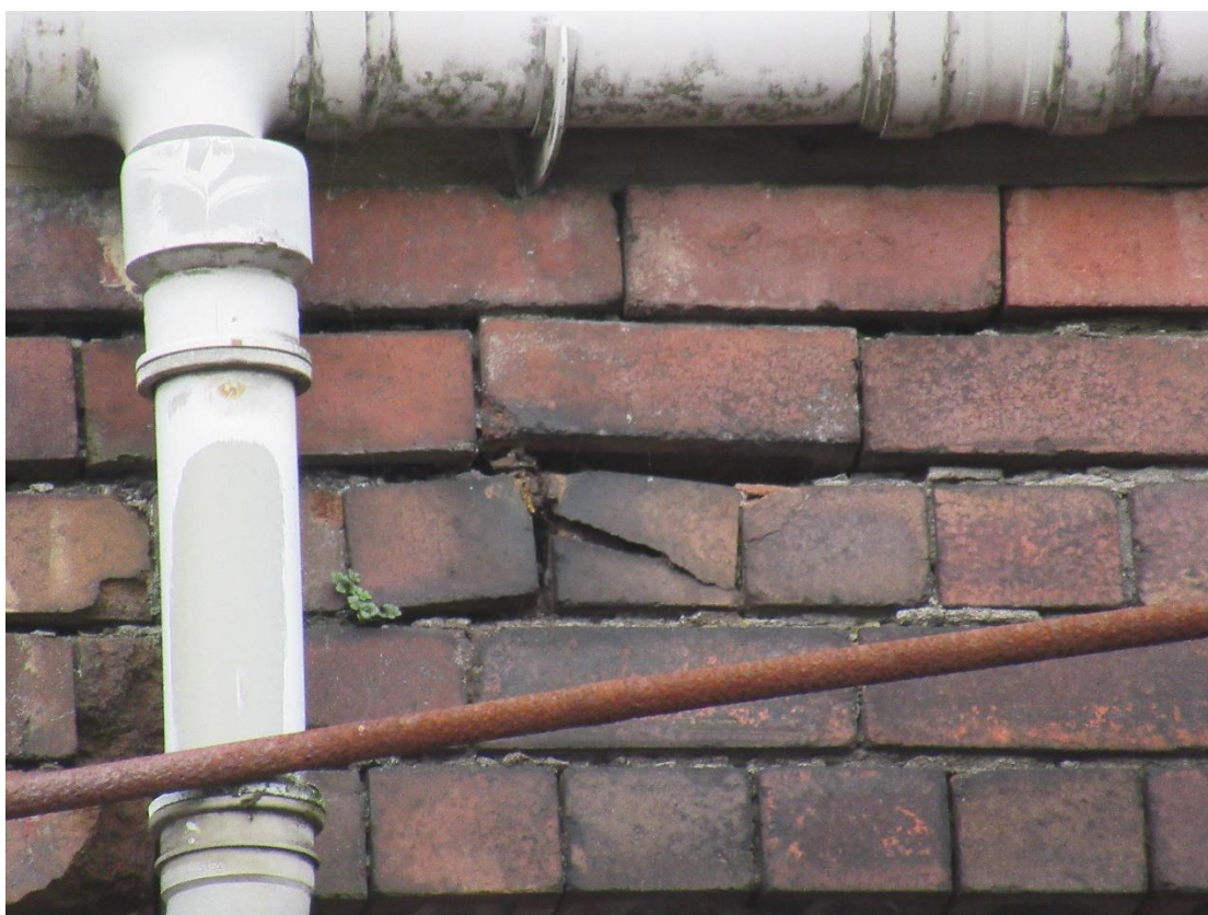
Photograph 12 – Example of gaps within the brickwork on the south-eastern aspect.
