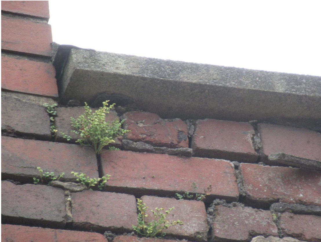
Photograph 13 – Example of gap under a coping stone on the north-western aspect.
