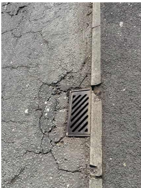
(37) Cracking to kerbs on northbound footway and carriageway and footway deterioration at kerb edge. Carriageway cracks on northbound side and significant subsidence surrounding gully.
