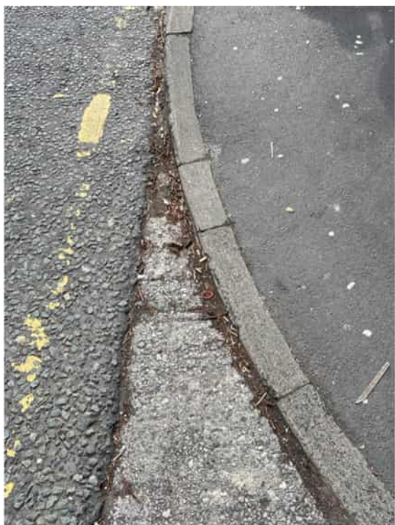
(11) Carriageway surface deterioration at TfGM access track junction. Minor cracks in kerbing. Line markings worn.
