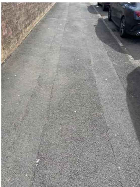
(41) Minor deterioration around trench scars on southbound footway surface.
