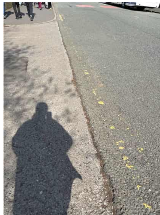
(16) Carriageway surface deterioration at interface between TfGM access track junction and Market Street on northbound side. Line markings worn.
