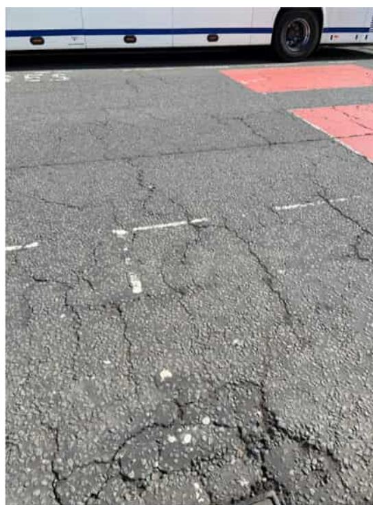
(38) Significant carriageway cracks on northbound side and line markings worn.
