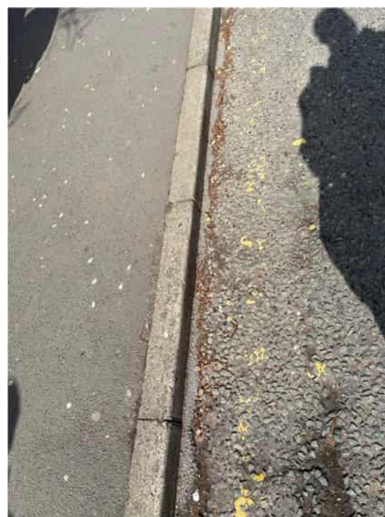
(8) Minor cracks on kerbs on northbound footway and minor carriageway and footway deterioration at kerb edge. Line markings worn.
