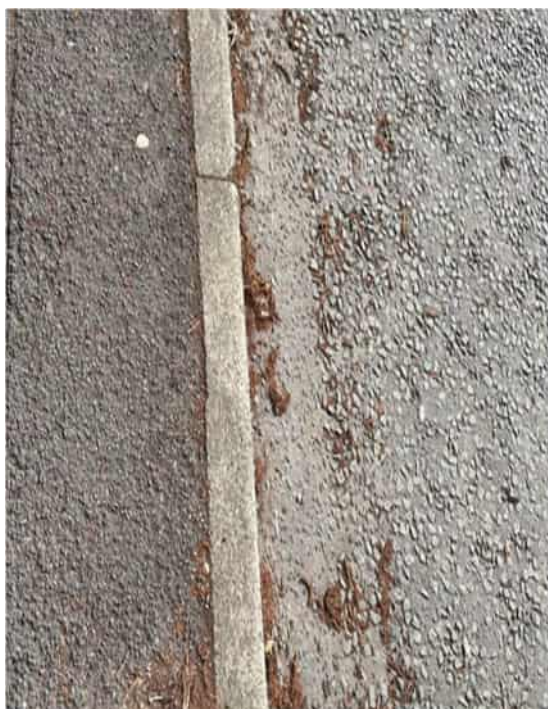
(75) Cracking to kerbs on southbound footway and carriageway and footway deterioration at kerb edge.
