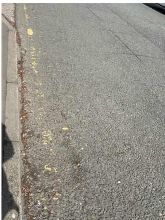
(7) Minor surface deterioration on northbound side carriageway. Line markings worn
