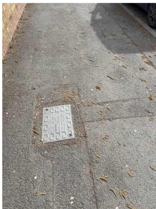
(62) Minor deterioration around trench scars on southbound footway surface.
