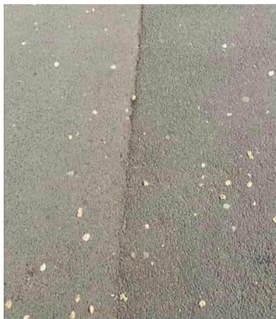
(4) Minor deterioration at resurfacing edge in northbound footway surface
