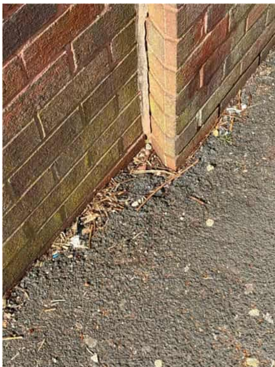
(1) Surface breakage along wall edge on northbound footway
