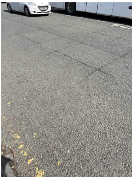
(15) Minor carriageway surface deterioration on northbound side. Line markings worn.
