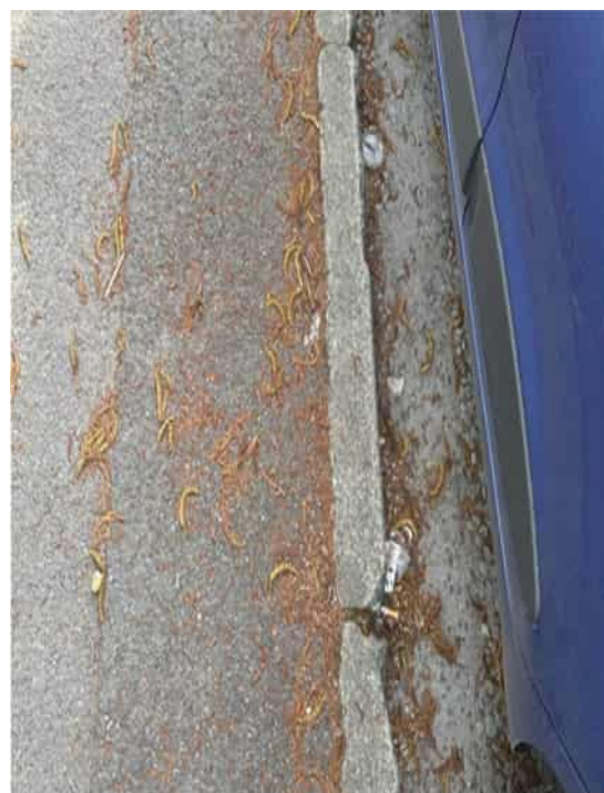
(68) Cracking and chipping to kerbs on southbound footway and carriageway and footway deterioration at kerb edge.
