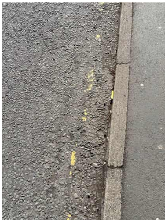
(27) Minor cracks on kerbs on northbound footway and minor carriageway and footway deterioration at kerb edge and along carriageway. Line markings worn.
