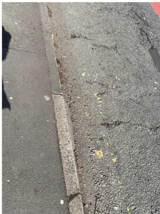
(33) Minor cracks on kerbs on northbound footway and minor carriageway and footway deterioration at kerb edge. Carriageway cracking. Line markings worn.
