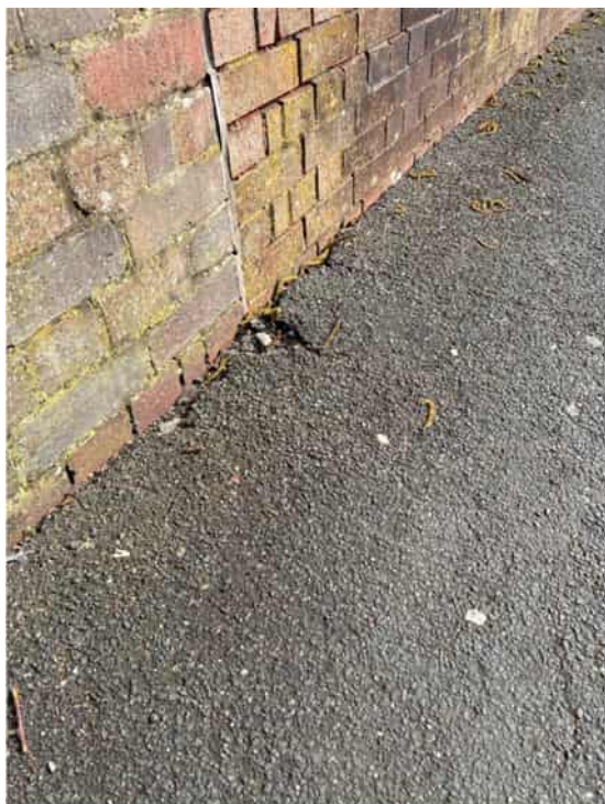
(61) Surface breakage along wall edge on southbound footway.
