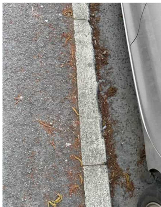
(72) Cracking and chipping to kerbs on southbound footway and carriageway and footway deterioration at kerb edge.
