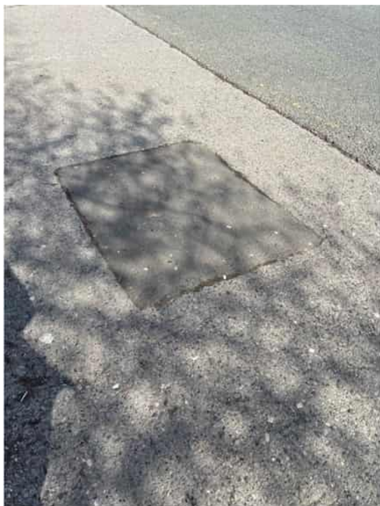
(17) Carriageway surface deterioration at interface between TfGM access track junction and Market Street on northbound side. Line markings worn.
