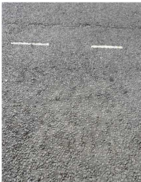
(76) Minor surface deterioration on carriageway on southbound side.
