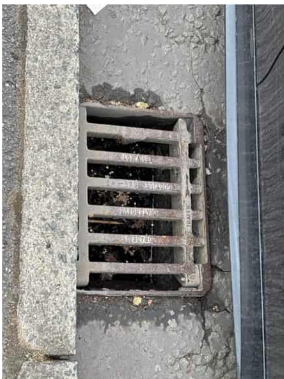
(45) Partially blocked gully on southbound side of carriageway. Minor cracking on surfacing around gully. Minor cracking to kerbs.
