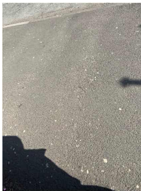
(34) Minor surface deterioration in northbound footway
