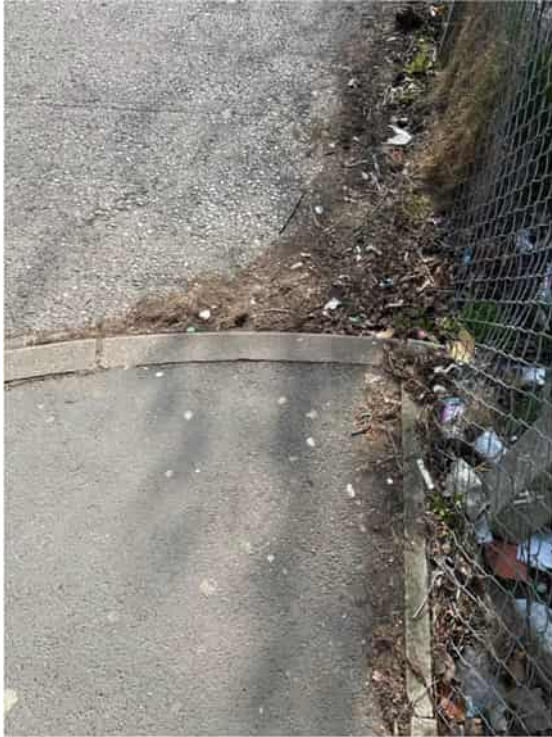
(21) Minor cracks on kerbs on northbound footway at TfGM access track junction and minor carriageway and footway deterioration at kerb edge. Build up of mud and debris.
