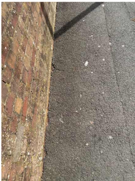
(53) Surface breakage along wall edge on southbound footway.
