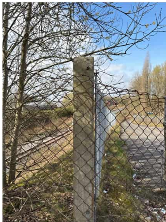
(18) Fencing loose from fence post at TfGM access track entrance
