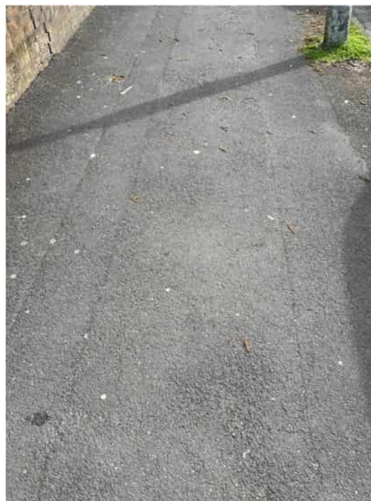
(56) Minor deterioration to southbound footway surface.
