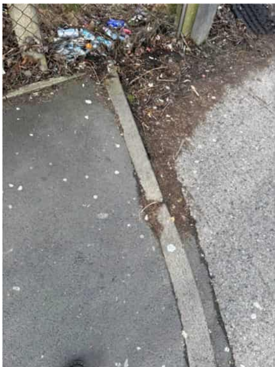
(13) Minor cracks on kerbs on northbound footway at TfGM access track junction and minor carriageway and footway deterioration at kerb edge. Build-up of mud and debris.
