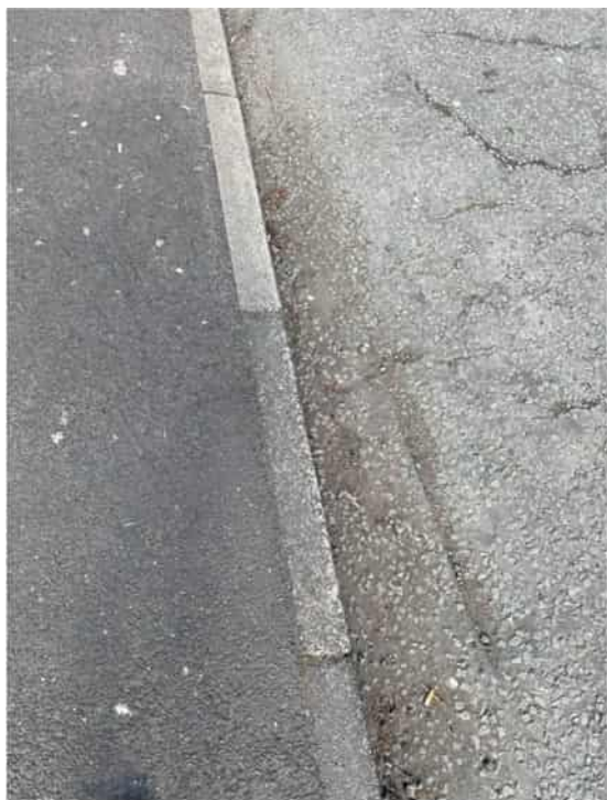
(39) Minor cracks on kerbs on northbound footway and minor carriageway and footway deterioration at kerb edge. Carriageway cracking
