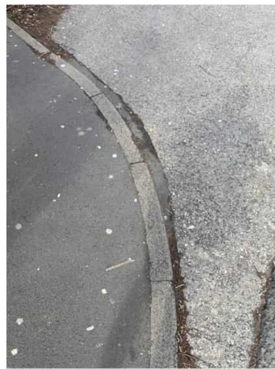
(12) Minor cracks on kerbs on northbound footway at TfGM access track junction and minor carriageway and footway deterioration at kerb edge
