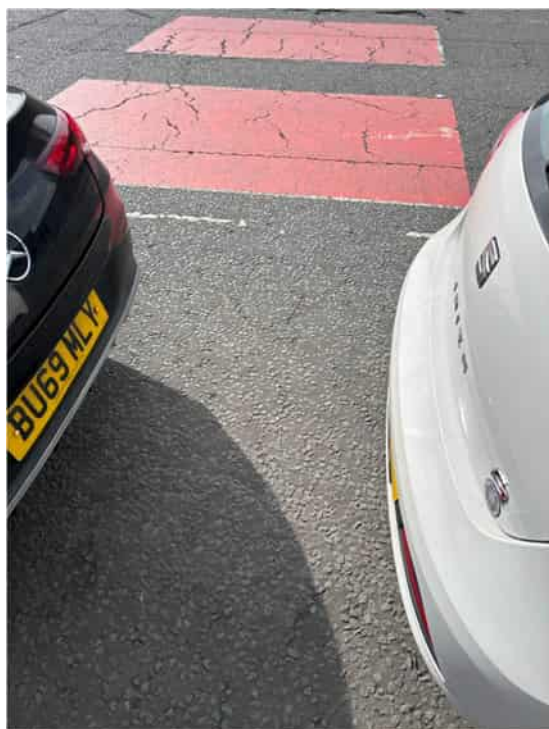
(43) Surface deterioration on northbound side carriageway. Line markings worn.
