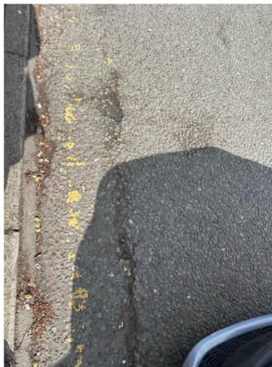
(6) Northbound side carriageway deterioration. Line markings worn
