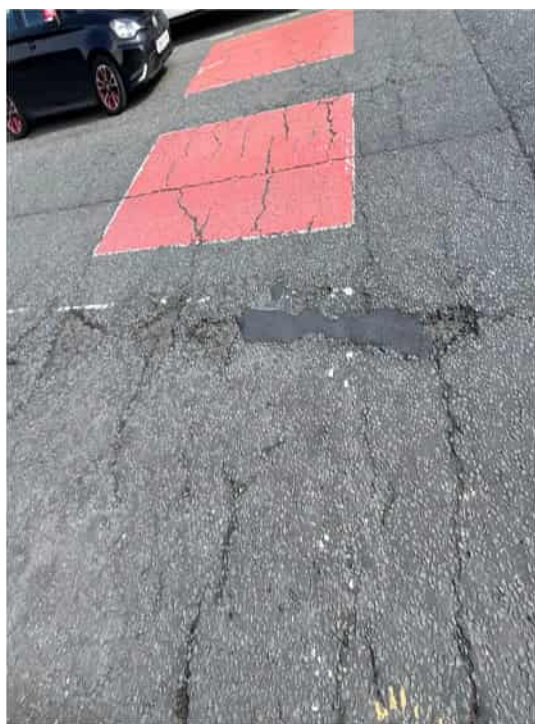
(31) Surface deterioration on northbound side carriageway. Minor potholes. Road markings fading.
