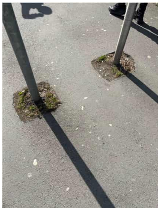
(28) Footway surface missing at post base on northbound footway, weed growth and slight footway deterioration surrounding edge of missing surface.
