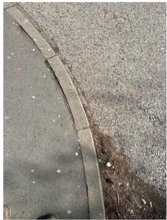
(22) Minor cracks on kerbs on northbound footway at TfGM access track junction and minor carriageway and footway deterioration at kerb edge. Build up of mud and debris.
