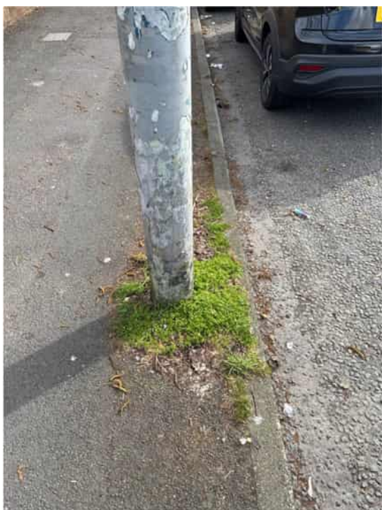
(57) Lamppost coating peeling and deteriorating. Weed growth and surface deterioration around lamppost base.
