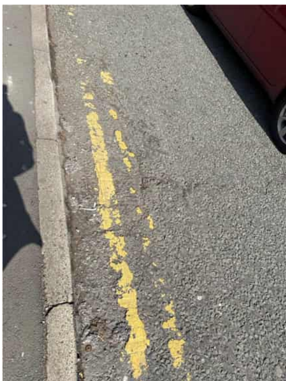
(25) Minor cracks on kerbs on northbound footway and minor carriageway and footway deterioration at kerb edge and along carriageway. Line markings worn.
