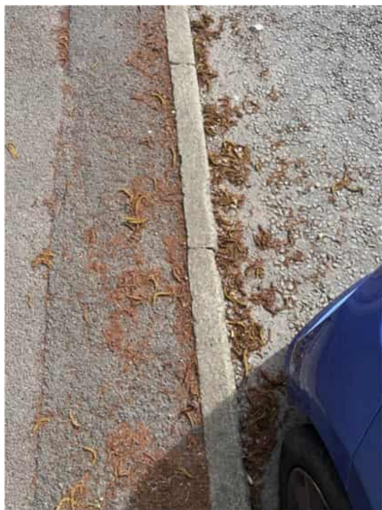
(69) Cracking and chipping to kerbs on southbound footway and carriageway and footway deterioration at kerb edge.
