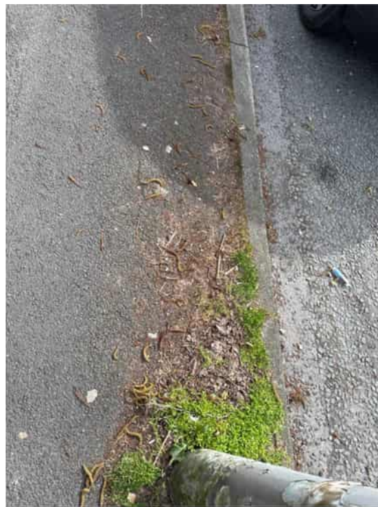
(58) Lamppost coating peeling and deteriorating. Weed growth and surface deterioration around lamppost base. Weed growth on footway edge. Build up of debris.
