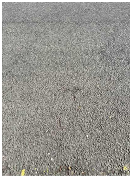
(14) Minor carriageway surface deterioration on northbound side
