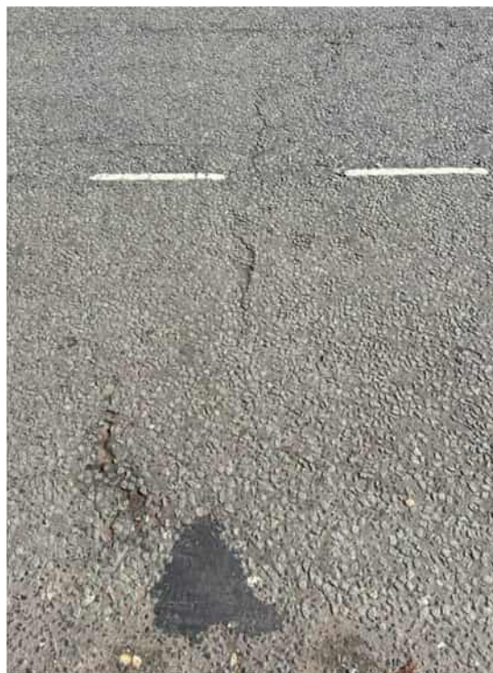
(2) Carriageway surface deterioration on northbound side
