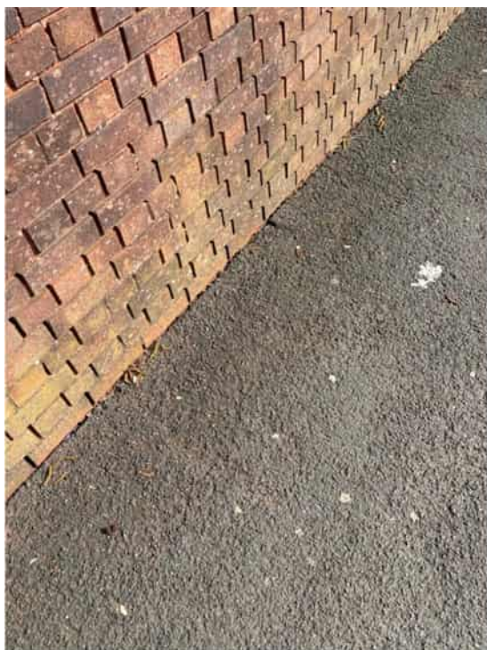
(73) Surface breakage along wall edge on southbound footway and minor deterioration to footway surface.
