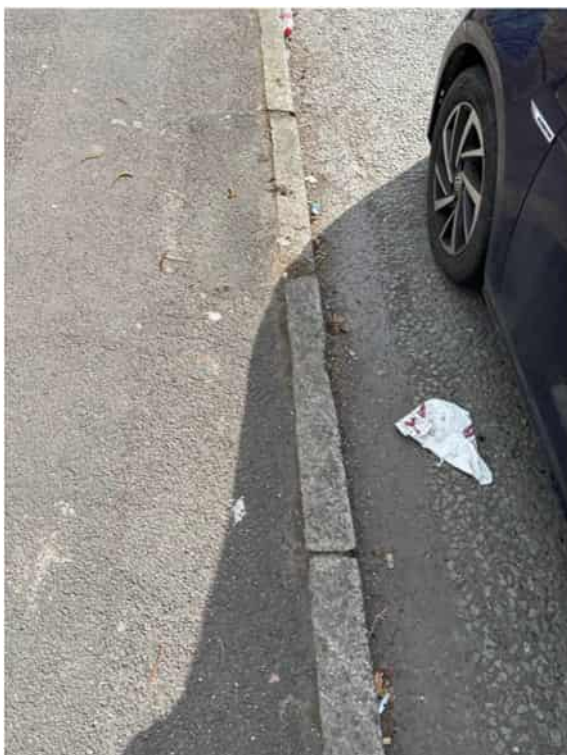
(49) Cracking to kerbs on southbound footway and carriageway and footway deterioration at kerb edge.
