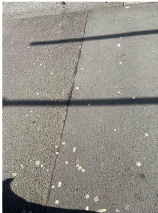
(32) Minor deterioration at resurfacing edge in northbound footway surface
