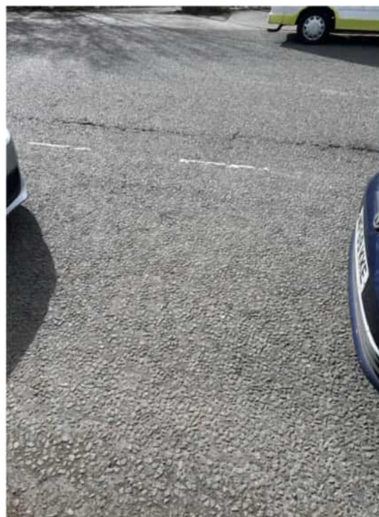
(50) Surface deterioration on northbound side carriageway. Line markings worn
