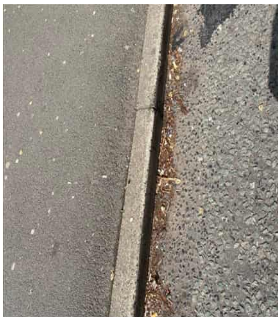
(3) Cracked kerbs along northbound footway
