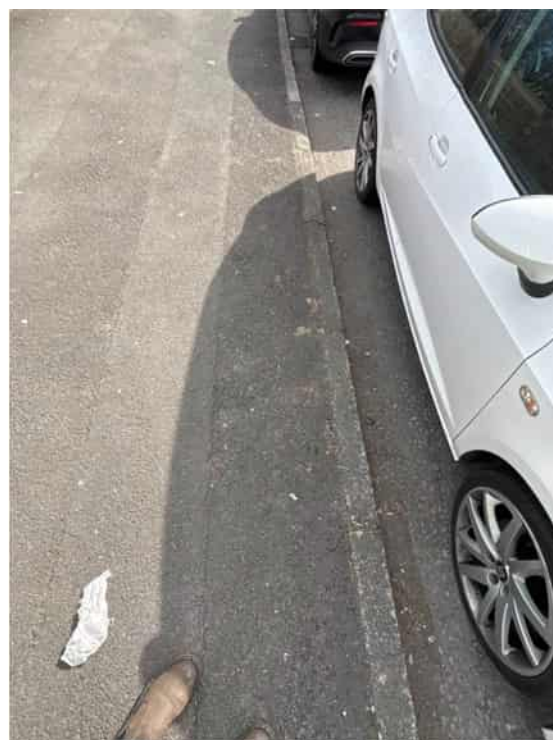
(42) Cracking to kerbs on southbound footway and carriageway and footway deterioration at kerb edge.
