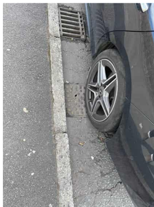
(44) Cracking to kerbs on southbound footway and carriageway and footway deterioration at kerb edge. Subsidence around utilities cover and cracking on carriageway.
