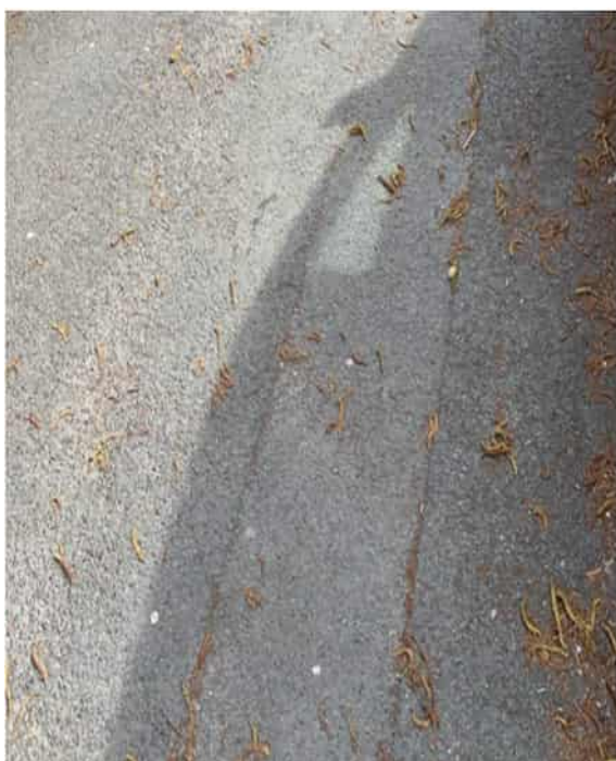
(67) Minor deterioration along footway and around trench scars on southbound footway surface.
