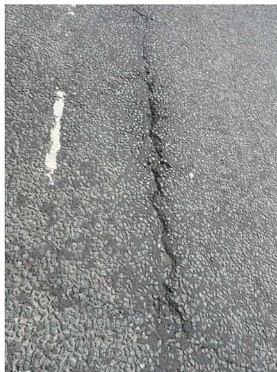
(54) Cracking in carriageway surface on southbound side. Line markings worn.
