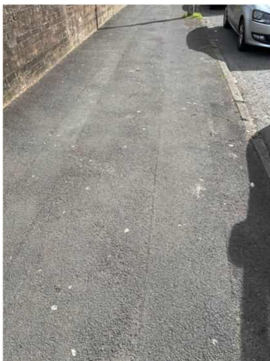
(47) Minor deterioration around trench scars on south bound footway surface
