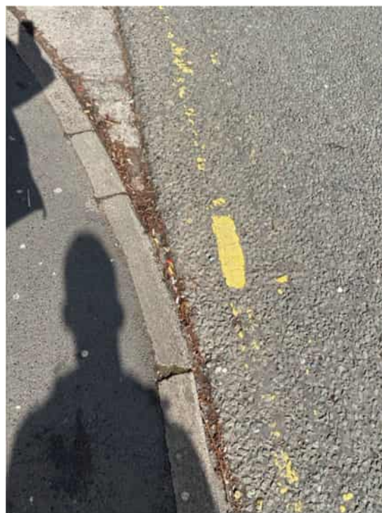
(10) Minor cracks on kerbs on northbound footway at TfGM access track junction and minor carriageway and footway deterioration at kerb edge. Line markings worn.
