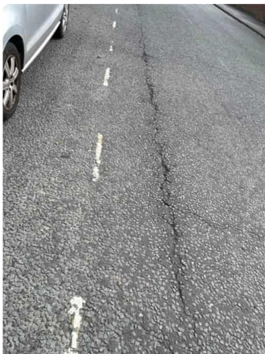
(55) Cracking in carriageway surface on southbound side. Line markings worn.
