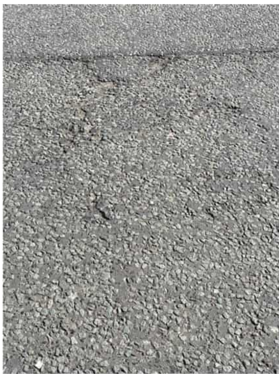
(29) Minor surface deterioration on northbound side carriageway
