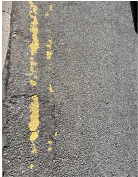
(24) Surface deterioration on northbound carriageway. Line markings worn.
