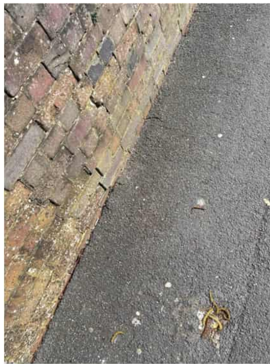
(60) Surface breakage along wall edge on southbound footway.
