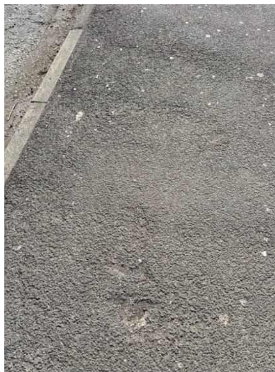
(36) Surface deterioration on northbound footway surface
