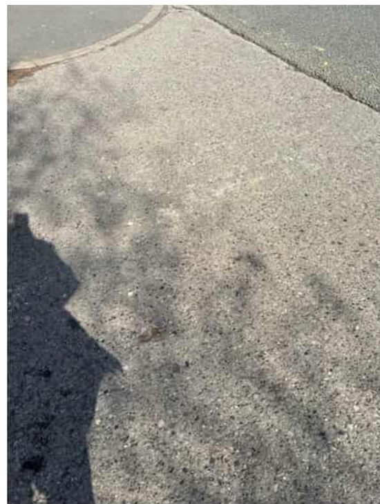
(20) Carriageway surface deterioration at interface between TfGM access track junction and Market Street on northbound side. Line markings worn.
