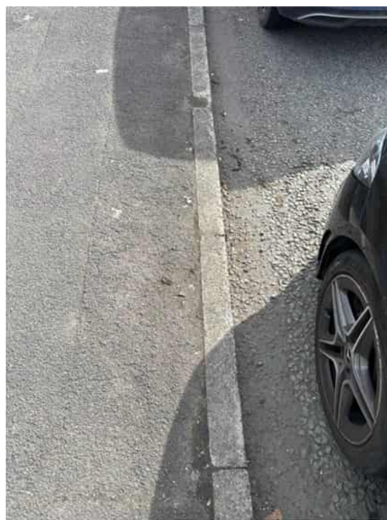
(46) Cracking to kerbs on southbound footway and carriageway and footway deterioration at kerb edge.
