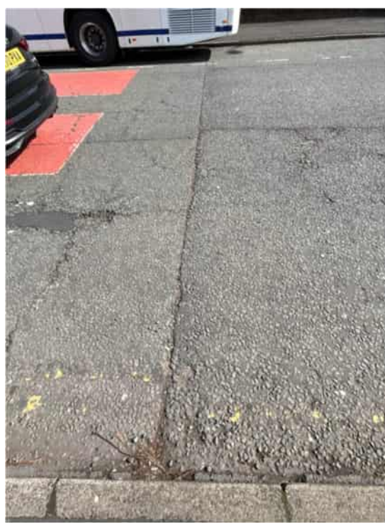
(30) Surface deterioration on northbound side carriageway. Line markings worn.
