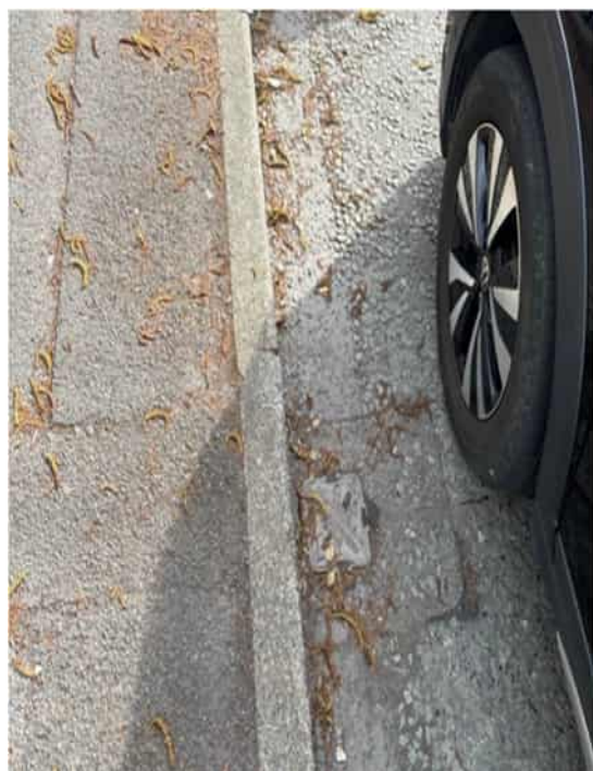
(64) Cracking to kerbs on southbound footway and carriageway and footway deterioration at kerb edge.
