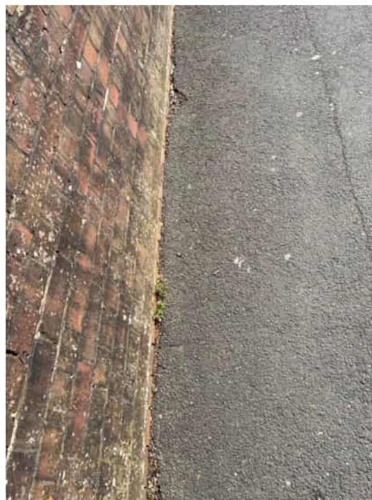
(48) Surface breakage along wall edge on southbound footway
