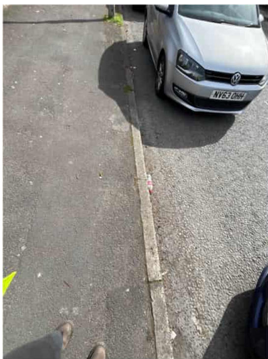
(51) Cracking to kerbs on southbound footway and carriageway and footway deterioration at kerb edge.
