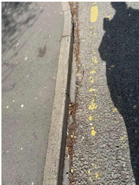
(9) Minor cracks on kerbs on northbound footway and minor carriageway and footway deterioration at kerb edge. Line markings worn.
