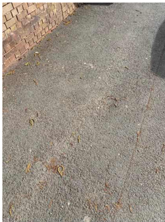
(70) Minor deterioration to southbound footway surface.
