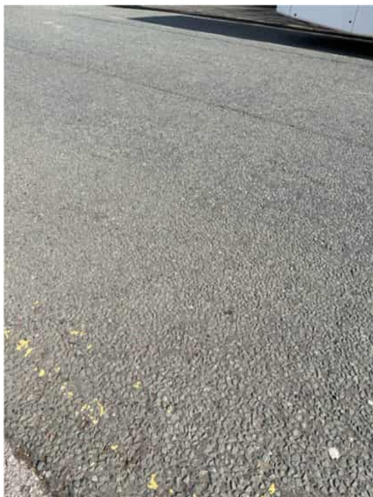
(19) Minor surface deterioration on carriageway. Line markings worn.
