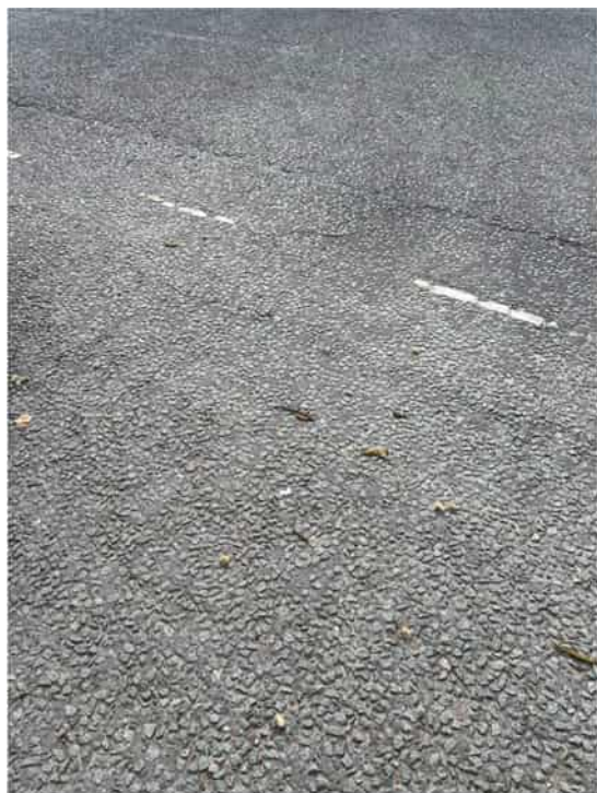
(59) Surface deterioration on northbound side carriageway. Line markings worn
