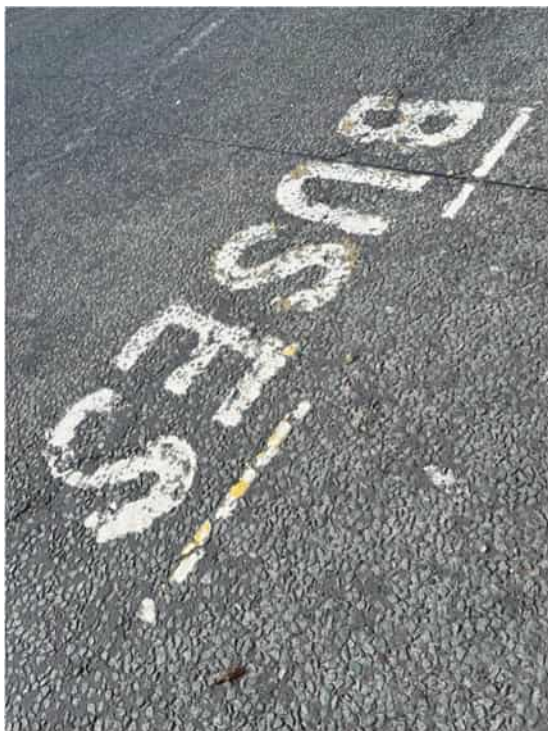
(65) Minor carriageway deterioration on southbound side and line markings worn.
