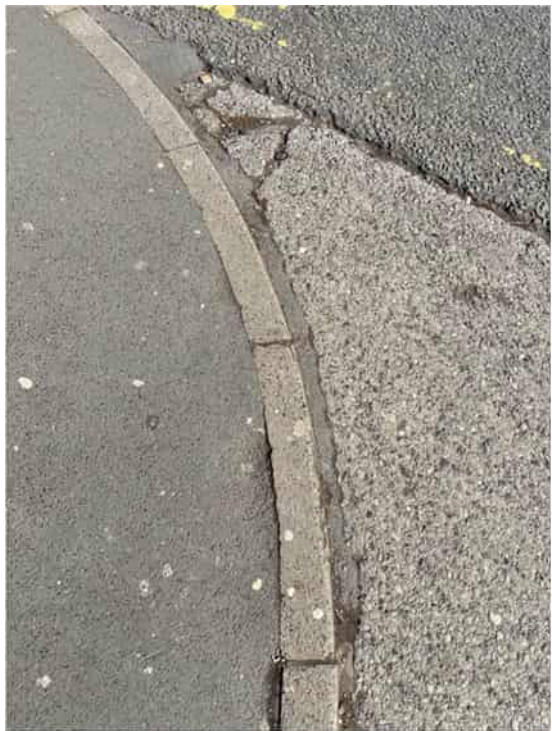
(23) Minor cracks on kerbs on northbound footway at TfGM access track junction and minor carriageway and footway deterioration at kerb edge. Line markings worn.
