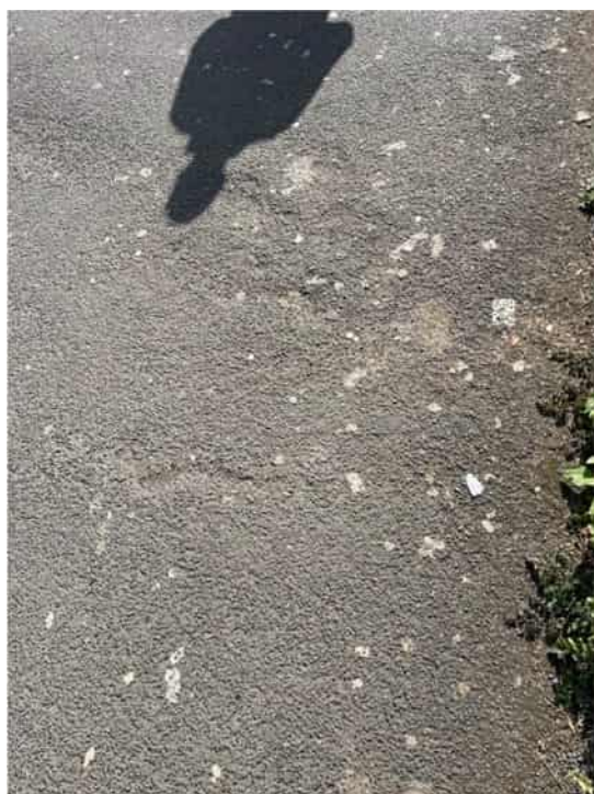
(35) Surface deterioration on northbound footway surface
