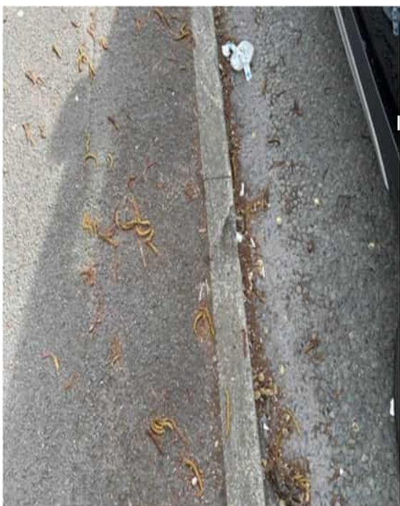
(63) Cracking to kerbs on southbound footway and carriageway and footway deterioration at kerb edge.
