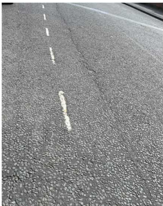
(71) Minor cracking in carriageway surface on southbound side. Line markings slightly worn.
