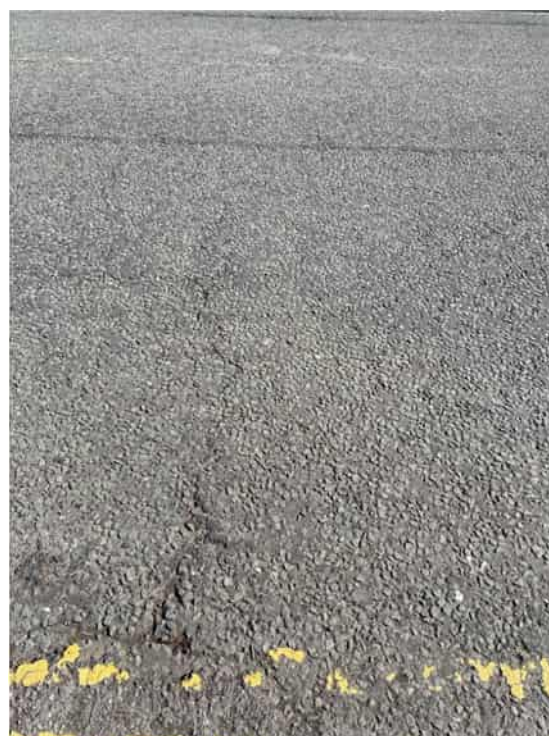
(26) Minor surface deterioration on northbound side carriageway. Line markings worn.
