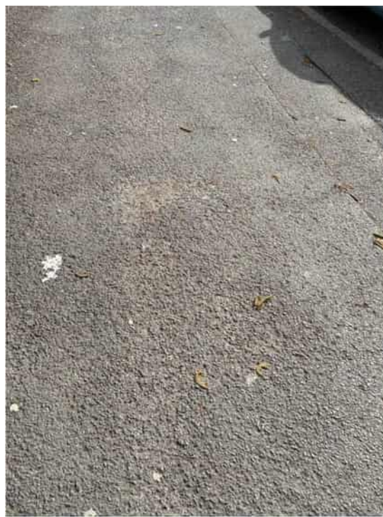
(74) Minor deterioration to footway surface.
