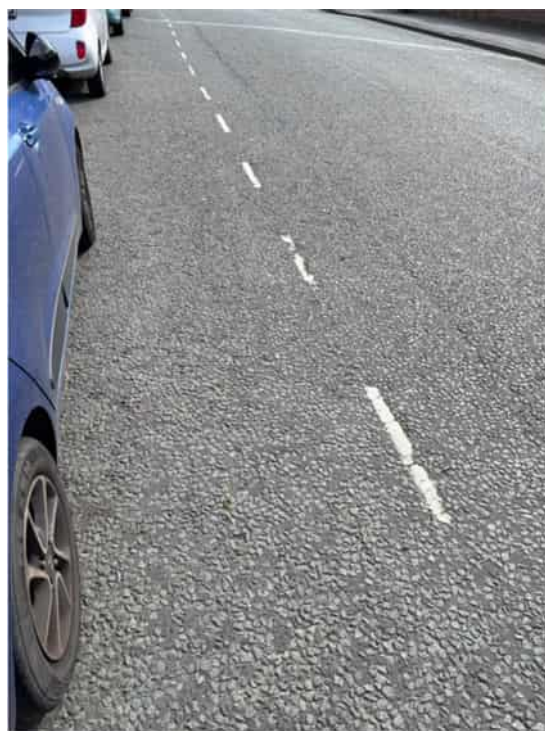
(66) Minor carriageway deterioration on southbound side and line markings worn.
