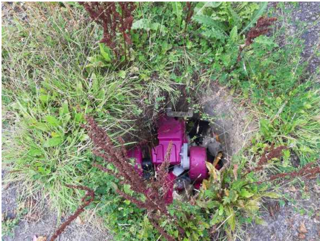
Plate 6 Detail of removed manhole cover and fly tipped material
