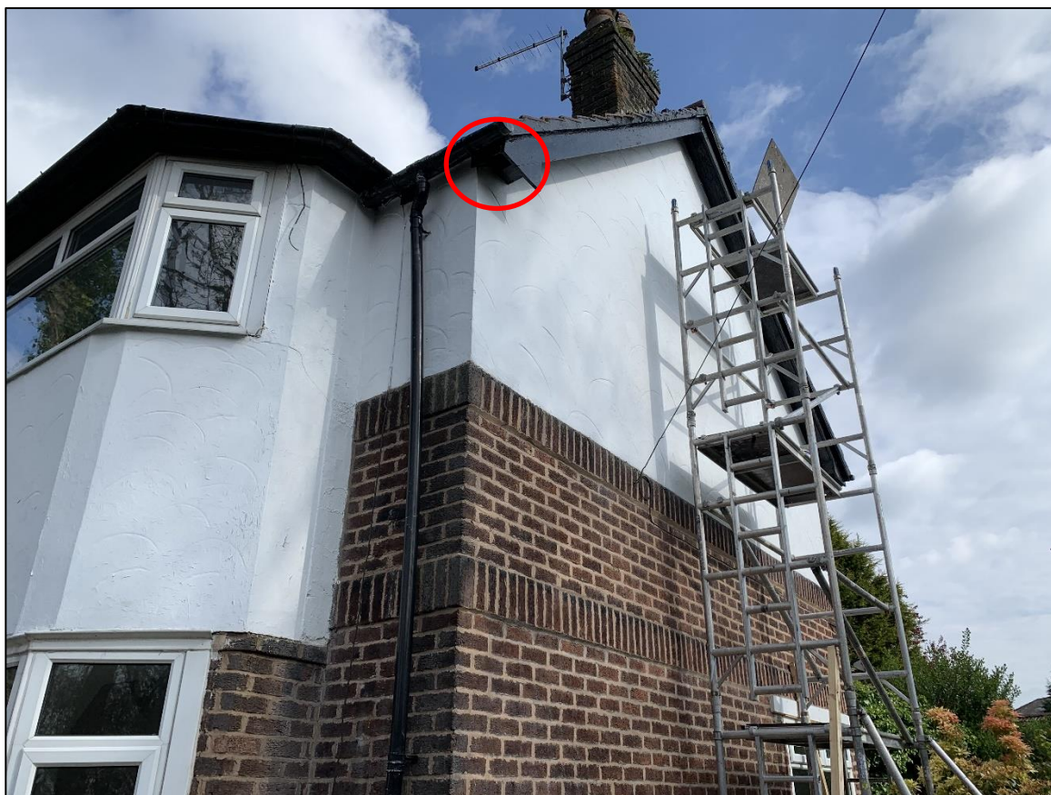
Plate 5 – Gap behind the barge board / soffit on the south-eastern elevation
