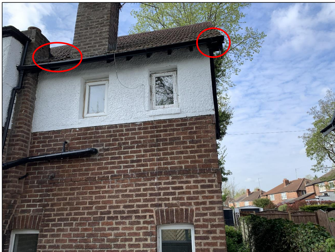
Plate 4 – Entry points on the north-eastern elevation, with a lifted tile to the left and an open barge board / soffit to the right
