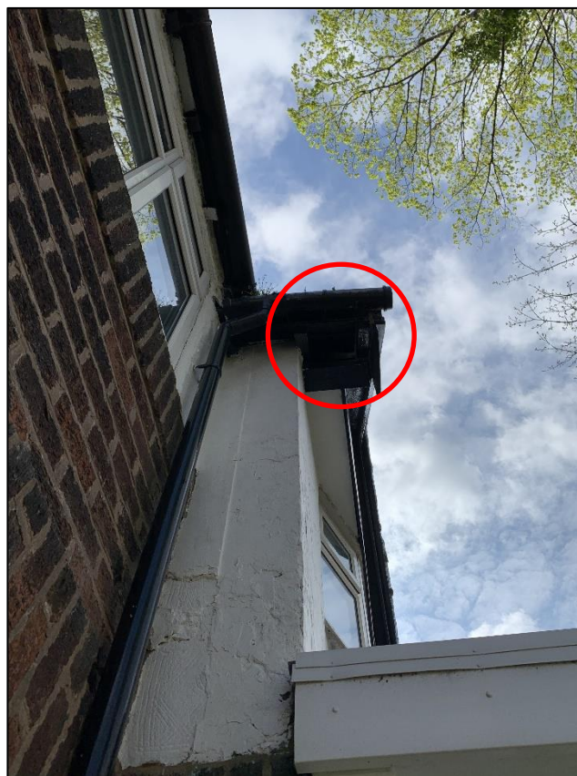
Plate 7 – Gap on the south-western elevation beneath the barge board / soffit
