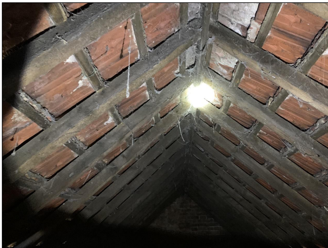
Plate 9 – The ridge beam, with heavy cobwebbing clearly present
