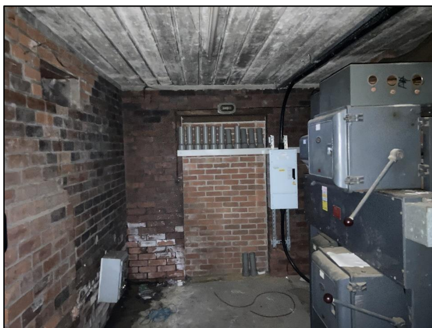
Photograph 29 showing the internal space of the plant room in Building 5
