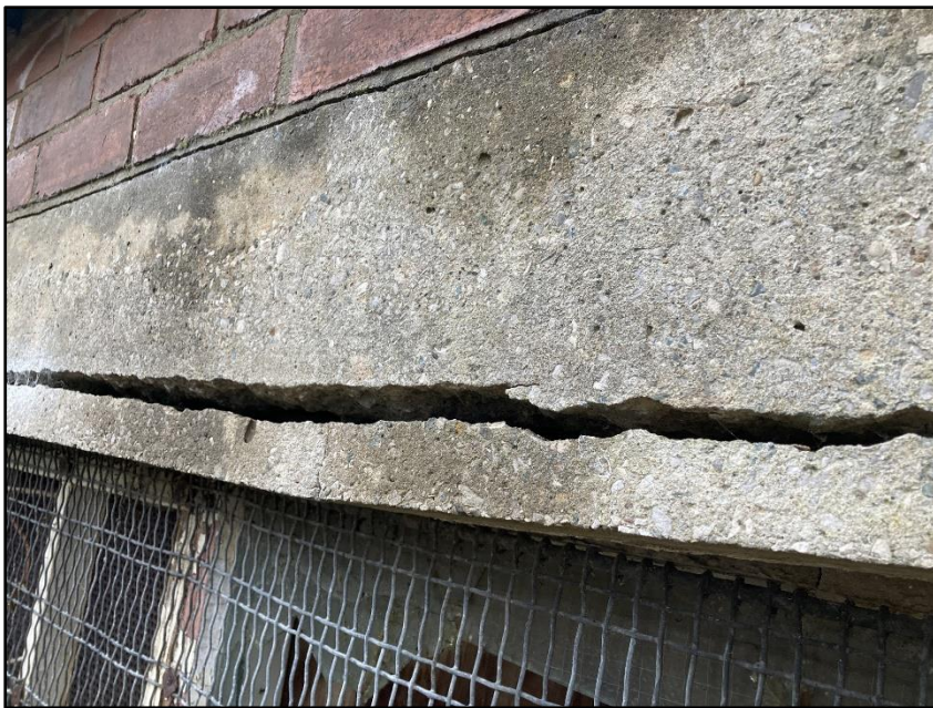
Photograph 13 showing the crack in the lintel on Building 2
