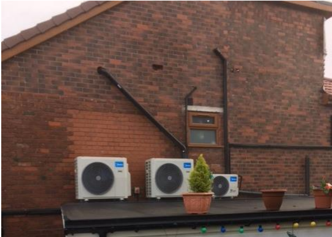
Image 8 – Photo of side elevation of host property demonstrating view of extraction units from the rear garden of No 50 Edenfield Road
