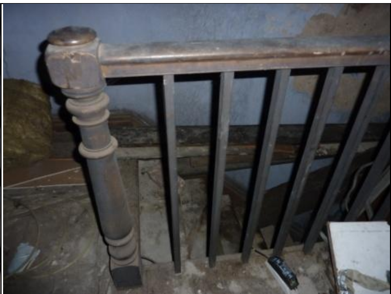
Redundant Attic Staircase
