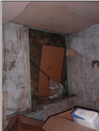
Blocked Window in the Northwest Room
