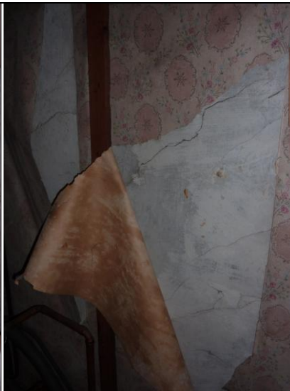
Plaster Wall with Peeling Wallpaper
