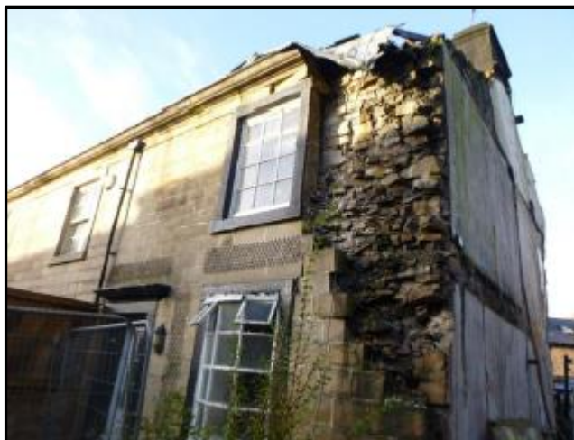
Figure 4: View of 4 East View damage to external façade
