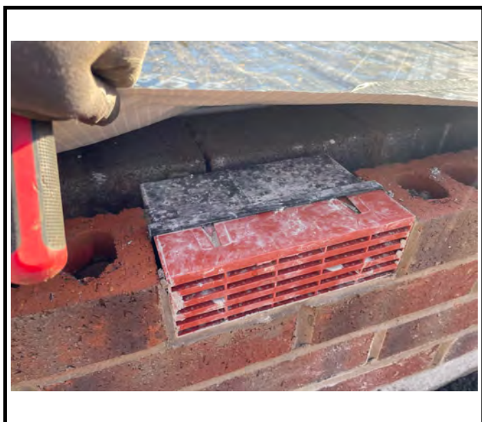
An air brick connected to a telescopic vent.
